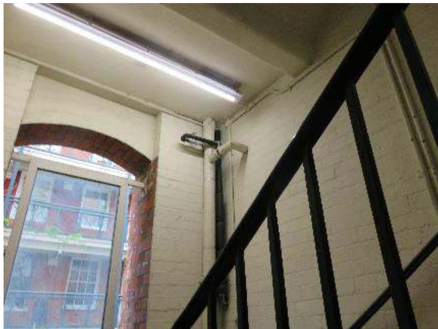
Rising Main with Potable branch in Beaumont Buildings
