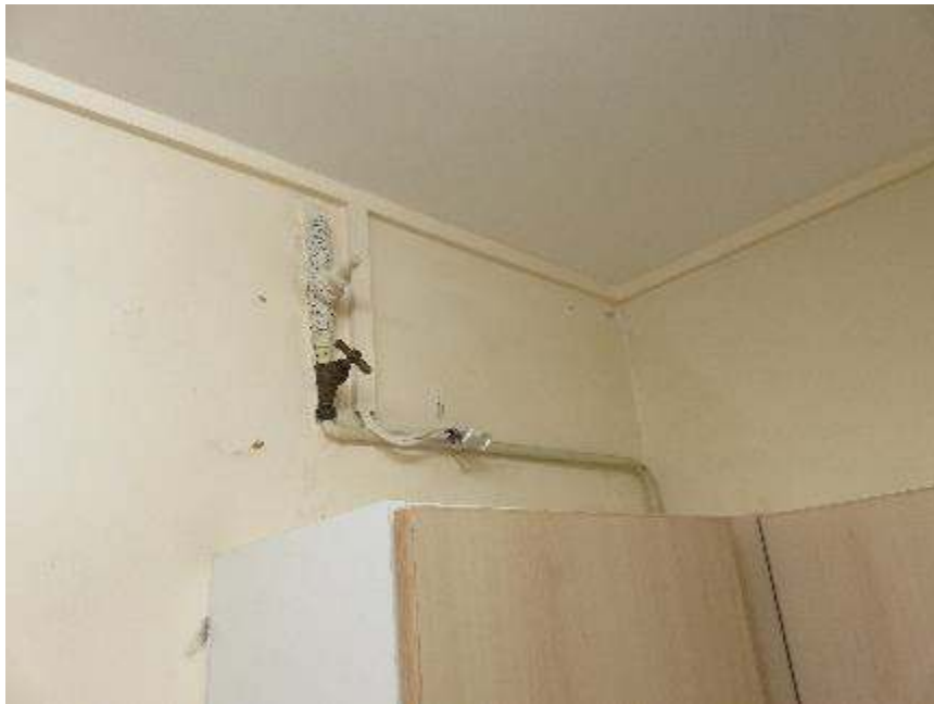
Some internal Pipework in Beaumont Buildings
