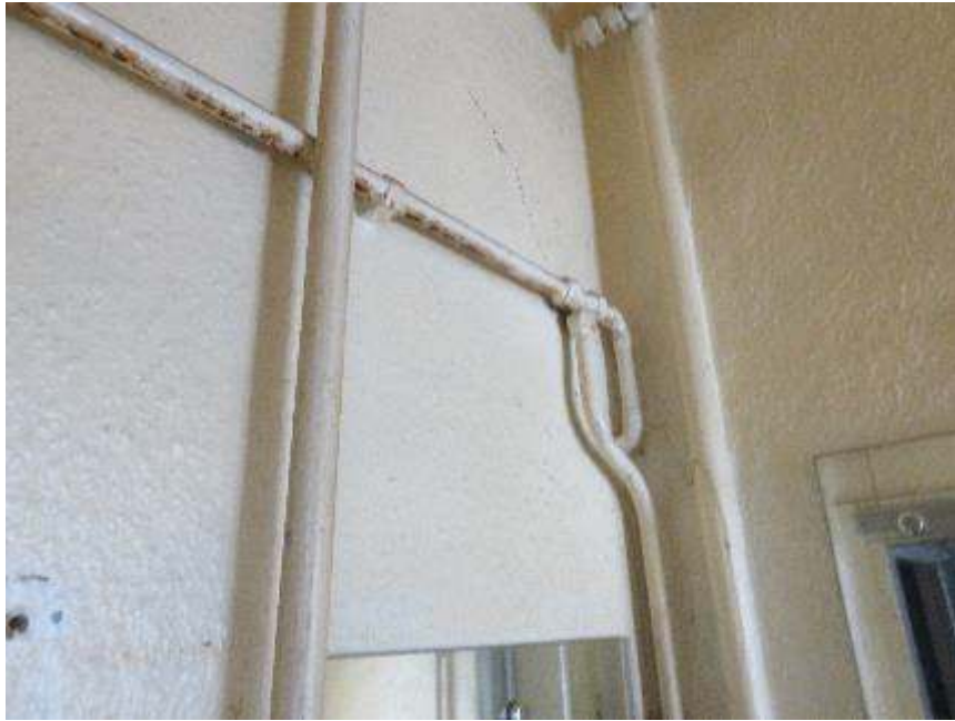
More internal pipework in flat in Sheridan Buildings.
