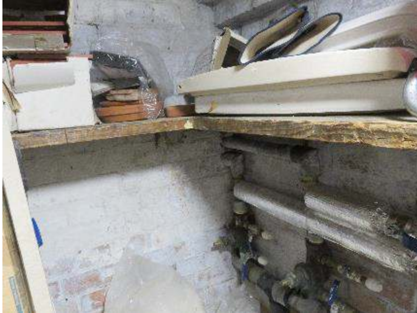
Incoming Water supply in Beaumont Buildings
