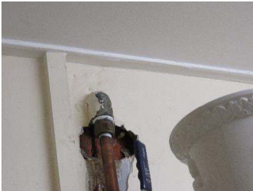
Some internal pipework in flat in Fletcher Buildings
