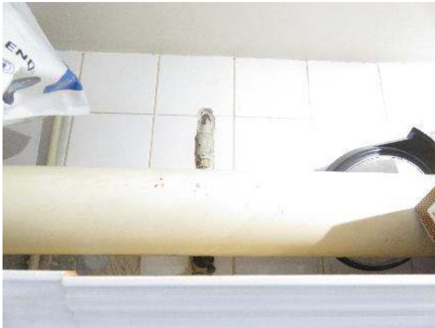
Some internal pipework in flat in Sheridan Buildings.
