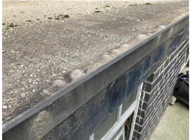
Blistering asphalt to communal heating room roof.
