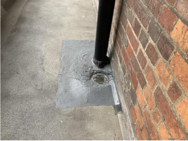
Liquid applied remedial coating indicating previous issues and repair history.
