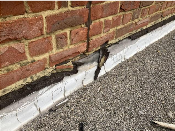
Further evidence of failed asphalt upstand.
