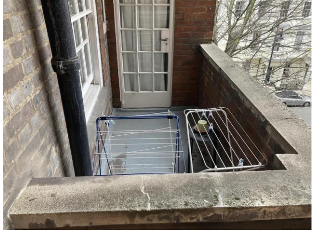
No access to private balconies.
