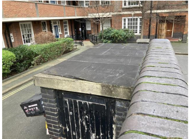
The bin store waterproofing is delaminating.
