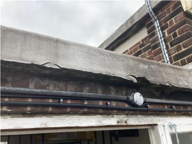
Asphalt to lift/tank roofs is failing. The drip edge is breaking away.
