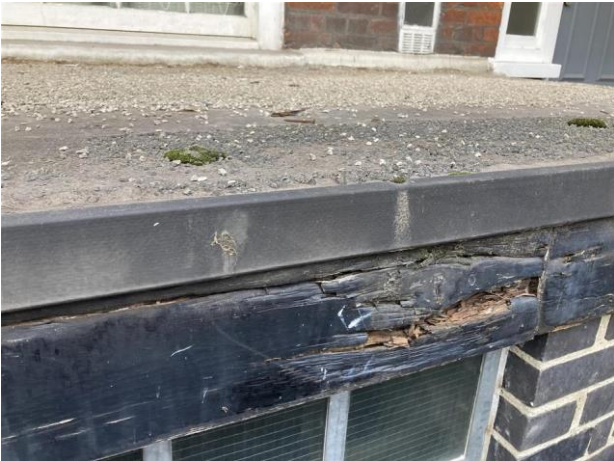
The fascia have reached the end of their life.
