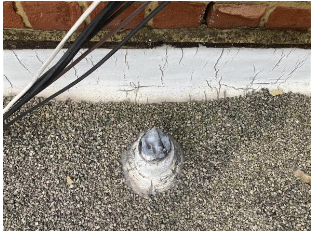
Termination to penetrations is no longer adequate.
