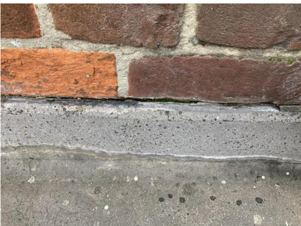
The asphalt upstand is beginning to come away from the brick parapet in areas, this will let water by.
