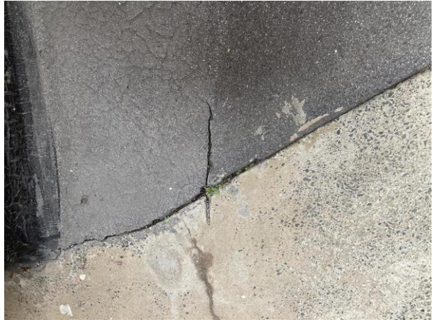
Split and cracks are occurring in areas.
