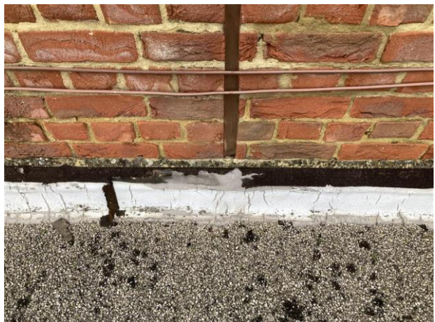
Advisory - vertical expansion joints should be renewed.
