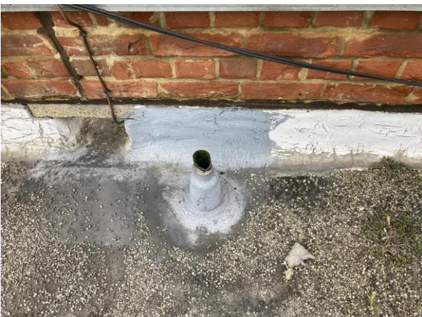
Liquid applied remedial coatings provide evidence of previous issues and repair history.
