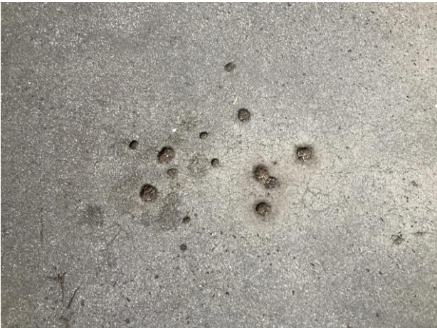
There are defects in the asphalt surface.
