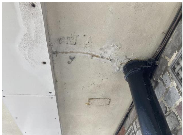
There is some damage to the concrete slab in areas.
