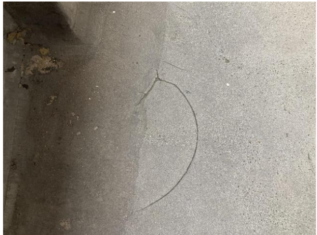
Splits and cracks are occurring in areas.
