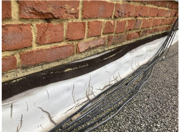
The asphalt upstand is failing and coming away from the brick parapet, this will let water by.
