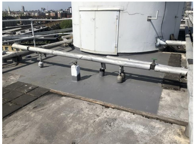
Evidence of previous repair suggests historic issues and reports of water ingress.
