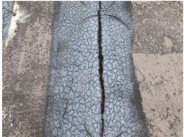
Defects in the asphalt will let water by.
