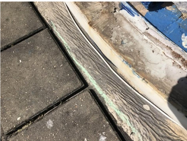
The asphalt is rippled and slumped, it has reached the end of its life.
