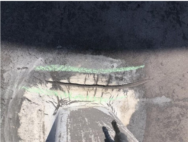
Further evidence of defects in the existing asphalt.
