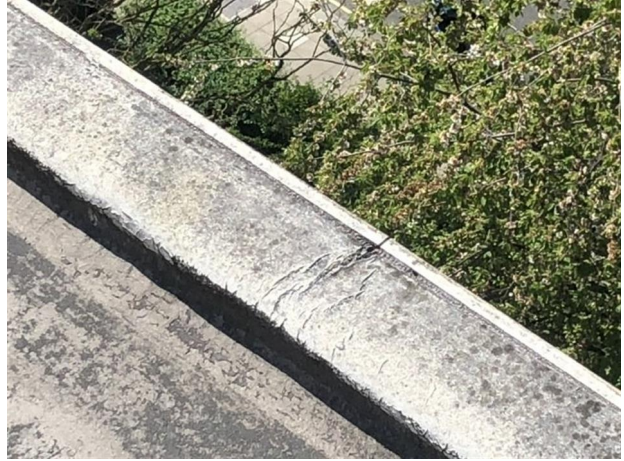
Cracks and splits are occurring in the asphalt.
