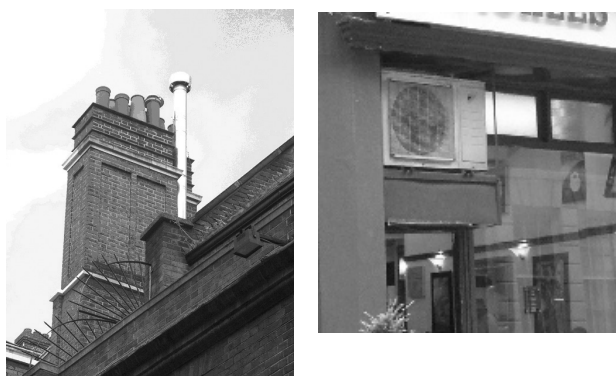
Figures 106 and 107: Flue to chimney at 22 Old Queen Street (left) and Air conditioning unit at 6 Old Queen Street (right)
