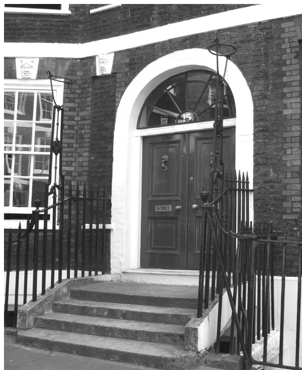
Figure 78: Original railings with urn and arrowhead finials and lamp holders either side of the stepped entrance
