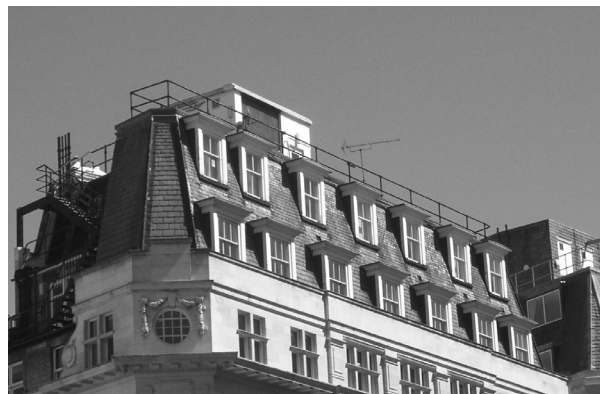
Figure 81: Tothill Street, Lift over-run/ plant room and railings set on a double height mansard.
