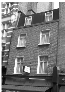
Figure 80: 16 Broadway. Windows have been replaced in aluminium with glazing bar pattern which does not reflect that of the original sashes and changes the proportions of the building as a whole
