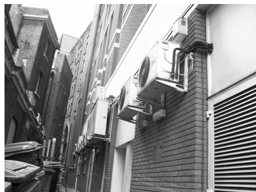
Figure 79: Un-screened air conditioning units to Strutton ground
