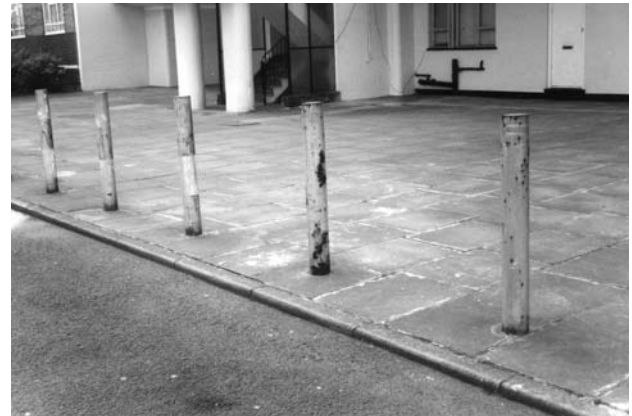
Figure 34: Poor maintenance of landscaping and street furniture
