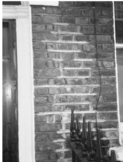
Figure 38: Poor standards of re-pointing are noticeable and blights the façade.
