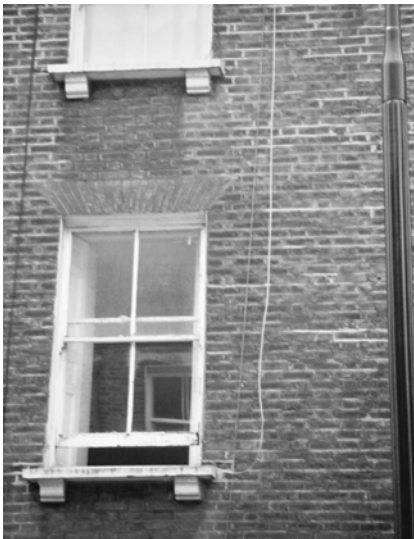
Figure 37: Wires run externally are unsightly accretions.
