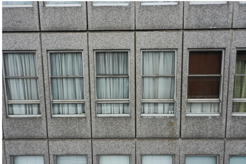
Photograph: Generic external view of Emanuel House East and West facades 1 st -5 th floors.
