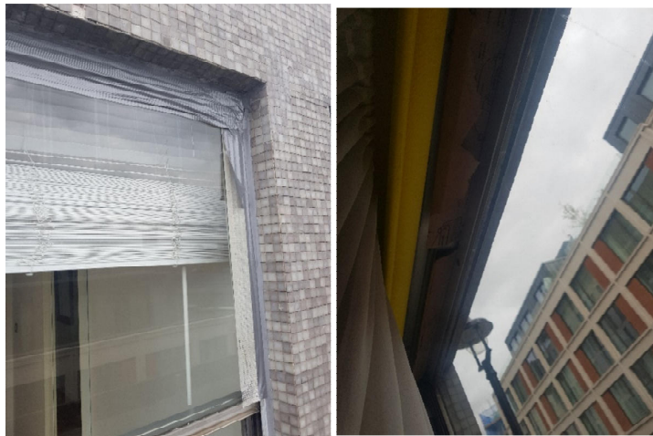
Photographs improvised draught proofing to sash windows duct tape and card board
