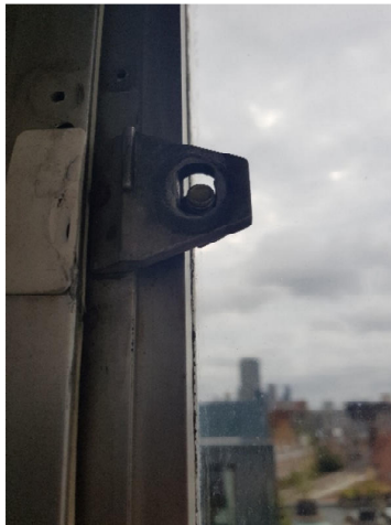
Photograph broken catch to offset pivot windows
