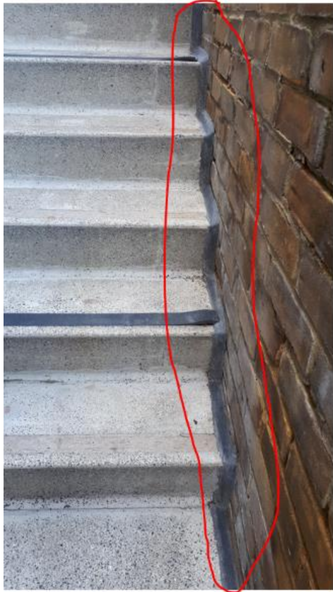
Photo 97. Same flank stairs, note re-jointing between tread/riser ends and brickwork. Some nosing strips missing and lifting.
