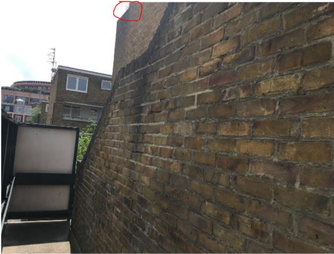
Photo 17. Same wall, different view and note the self-seeded vegetation (red) growing out of the private balcony parapet higher up the building; this is almost generic across all four Blocks.
