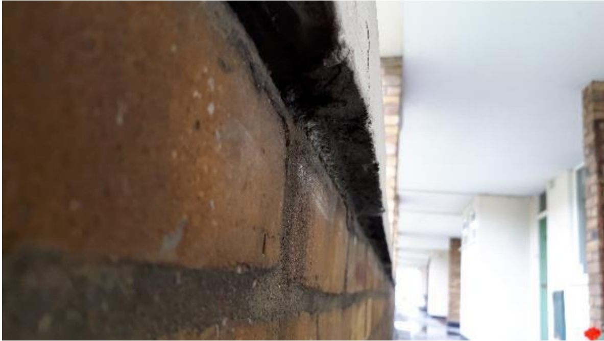
Photo 71. As-built coping simply too narrow as inside edge of drip groove should be a minimum 20mm clear of the brickwork face. Moisture has travelled back under the copings and with freeze thaw action on these north facing elevations as well as rebar corrosion has caused them to fail.
