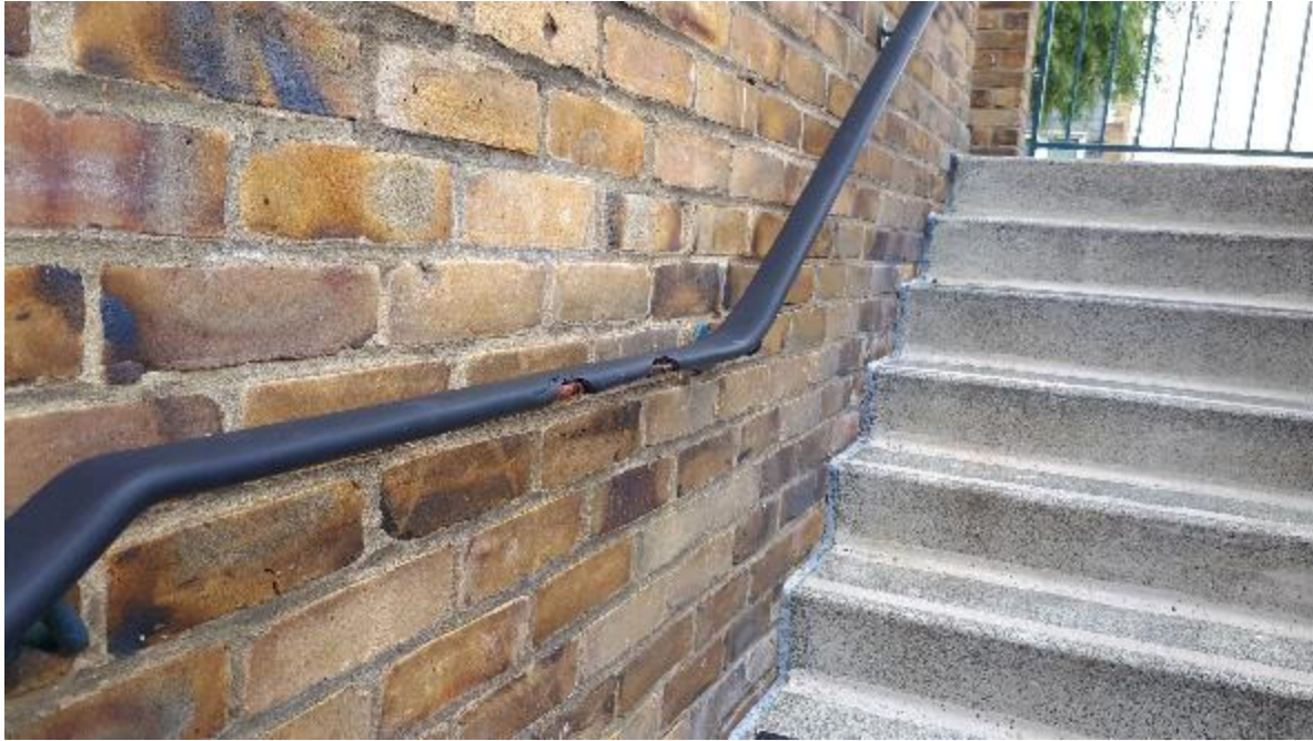
Photo 111. As on another Block, the handrail grip is defective.
