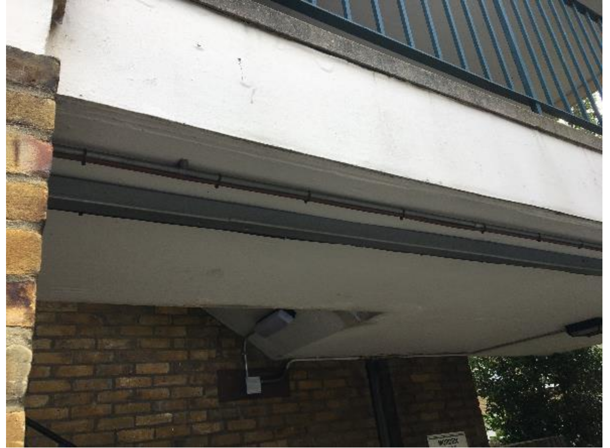
Photo 28. Stairwell soffit requiring redecoration.
