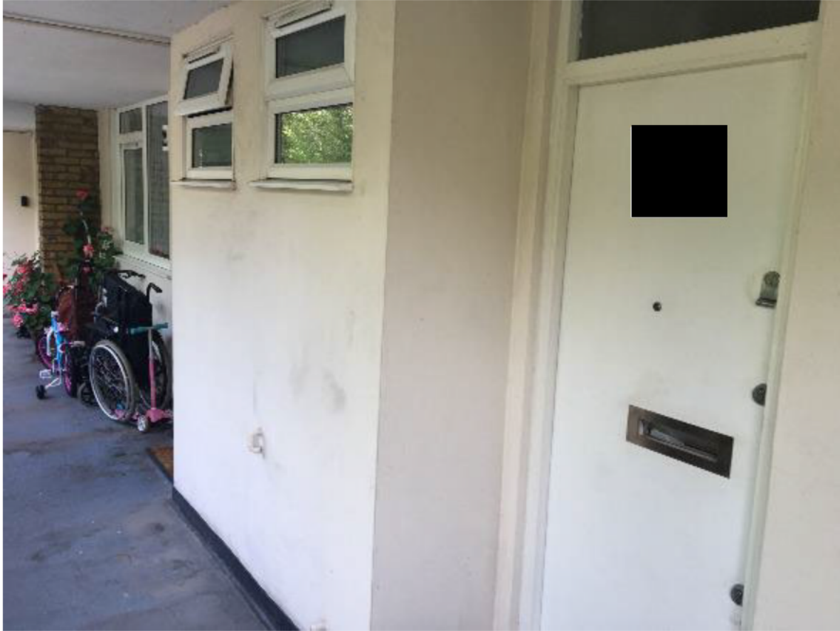
Photo 39. Close-up of decorations in fair condition exhibiting the usual signs of fair wear and tear. The windows and entrance doors are in fair condition, the PVCu components will need cleaning.
