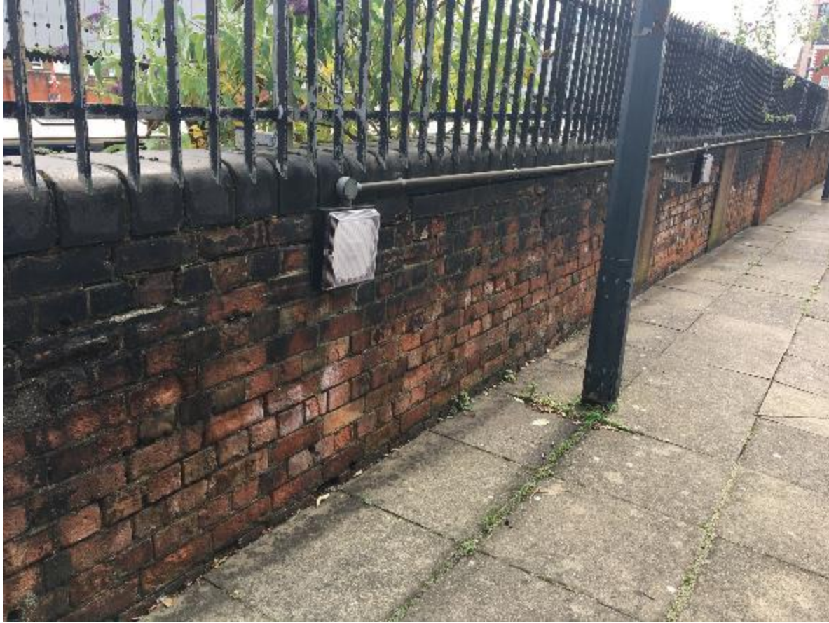
Photo 167. Defective pointing and spalling bricks to boundary wall adjacent railway as well as failing paintwork to railings.
