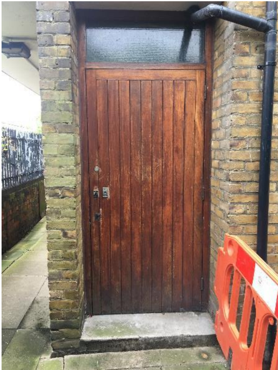
Photo 47. Generically across all four Blocks, decorations to store doors are in poor condition.
