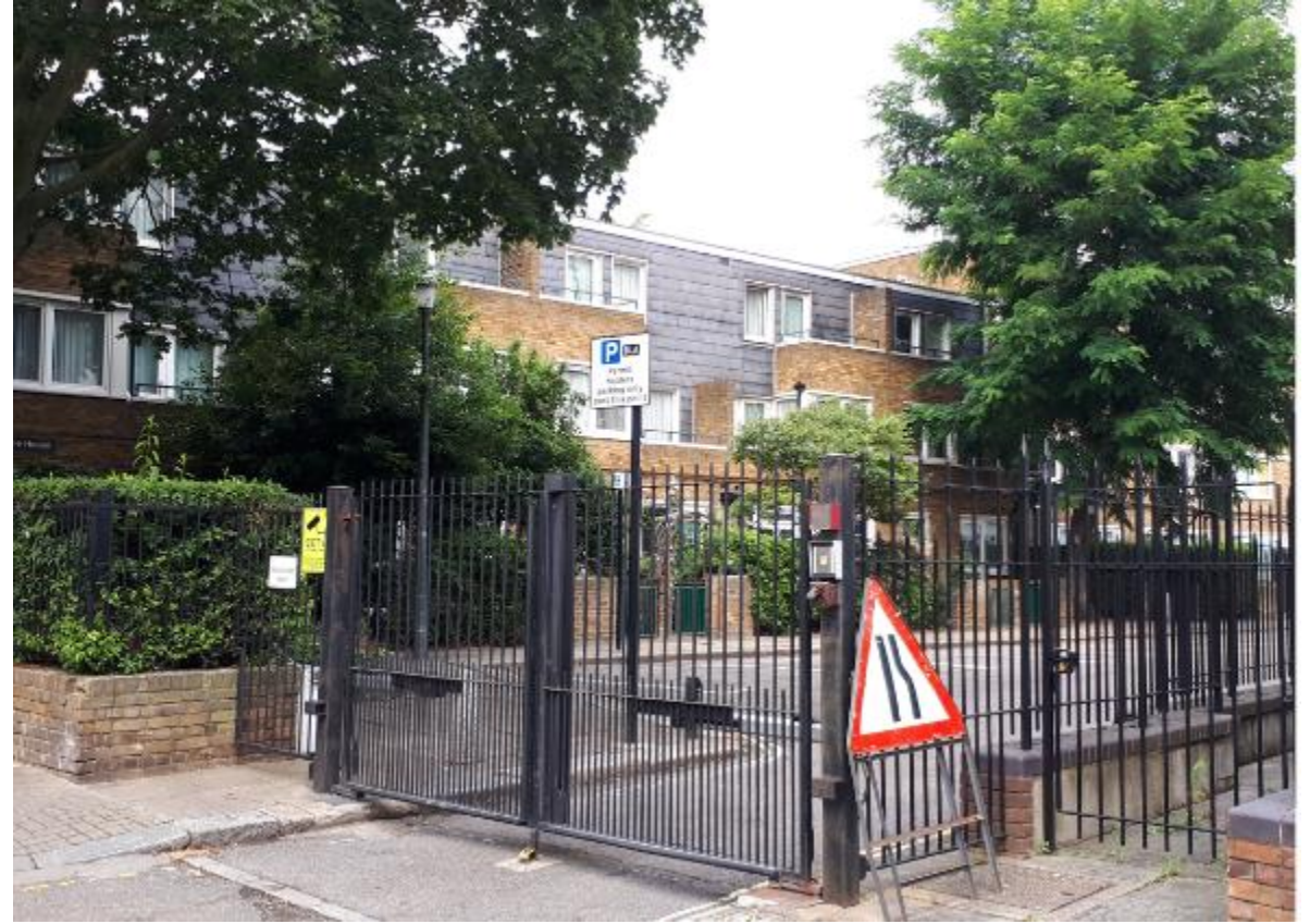
Photo 166. Signs of corrosion to vehicular gates.
