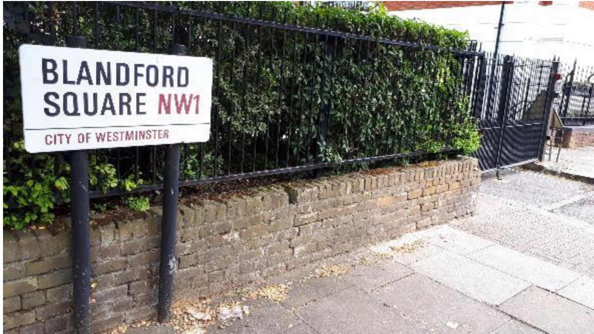
Photo 163. Another example of defective brickwork to the boundary walls.
