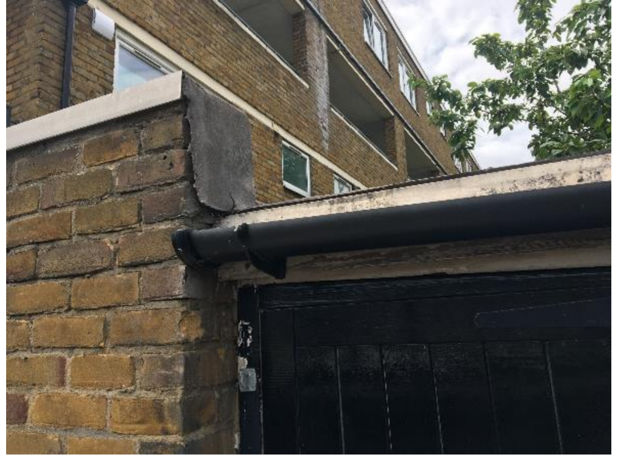
Photo 120. Second pram shed again showing defective mastic asphalt covering.
