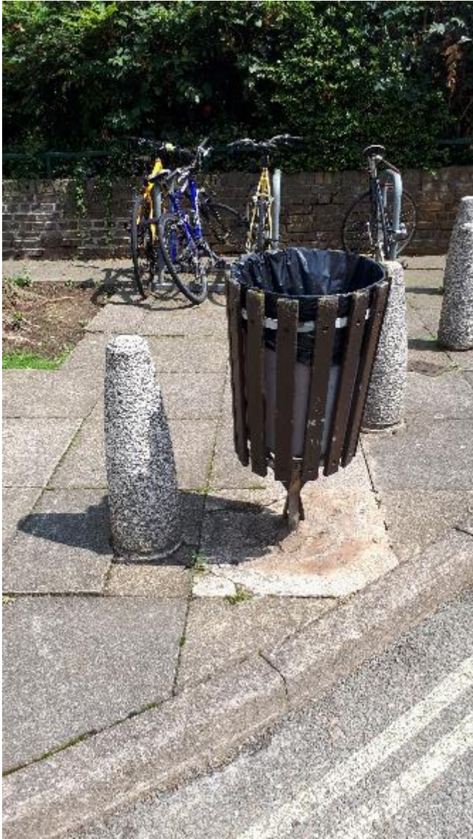
Photo 149. Decorations to litter bin failing.
