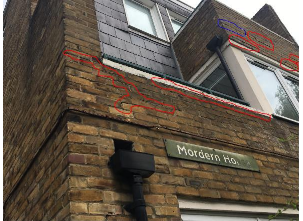
Photo 12. A generic defect to all Blocks is this localised defective pointing (red) to the 1 st and 2 nd flr rear private balcony parapets. Note the exposed DPC (blue) and the signage ought to be replaced.
