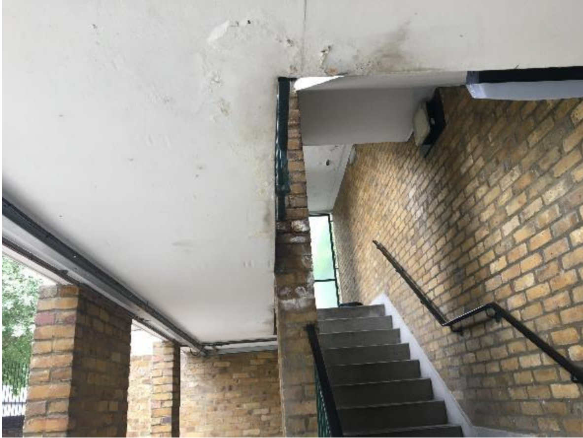
Photo 29. Evidence of water damage to decorations of soffit.
