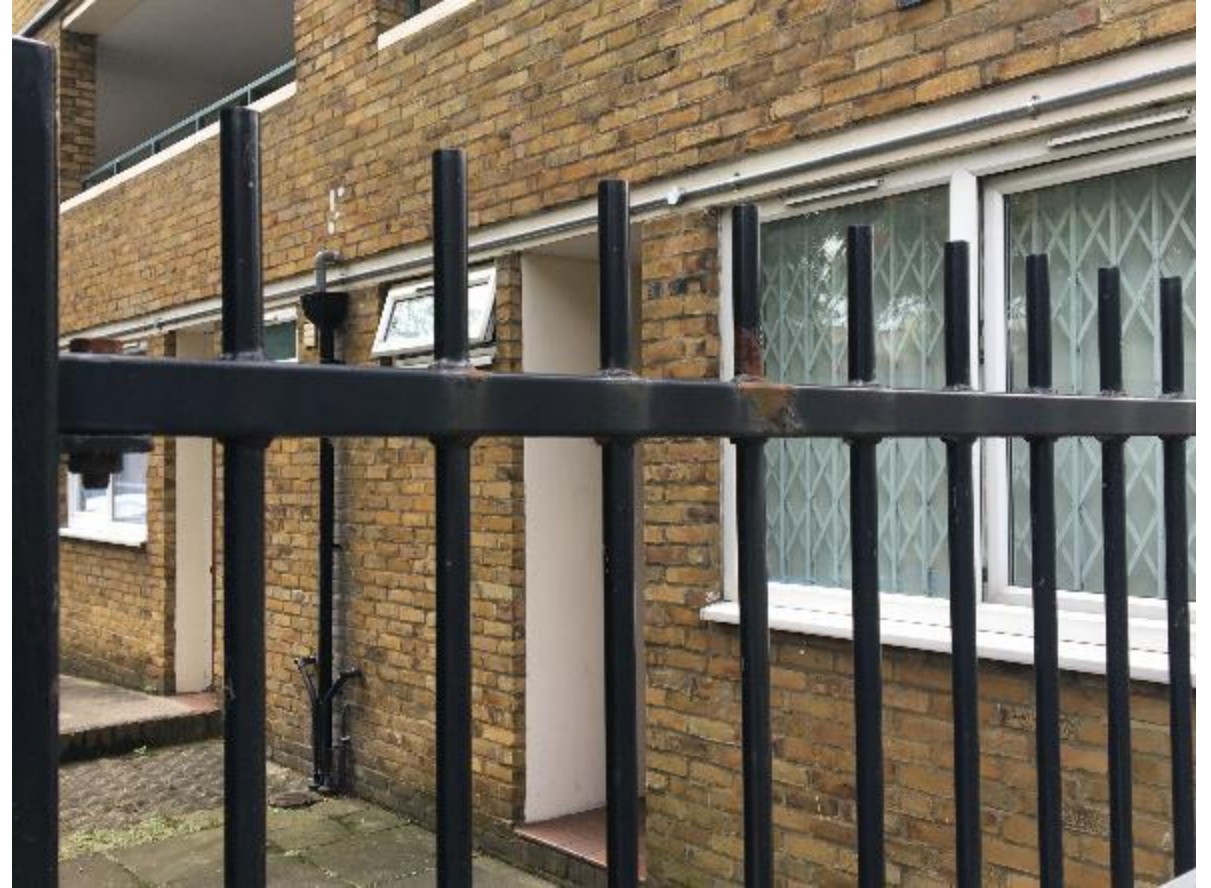
Photo 164. Powder coated paintwork to boundary railings failing.
