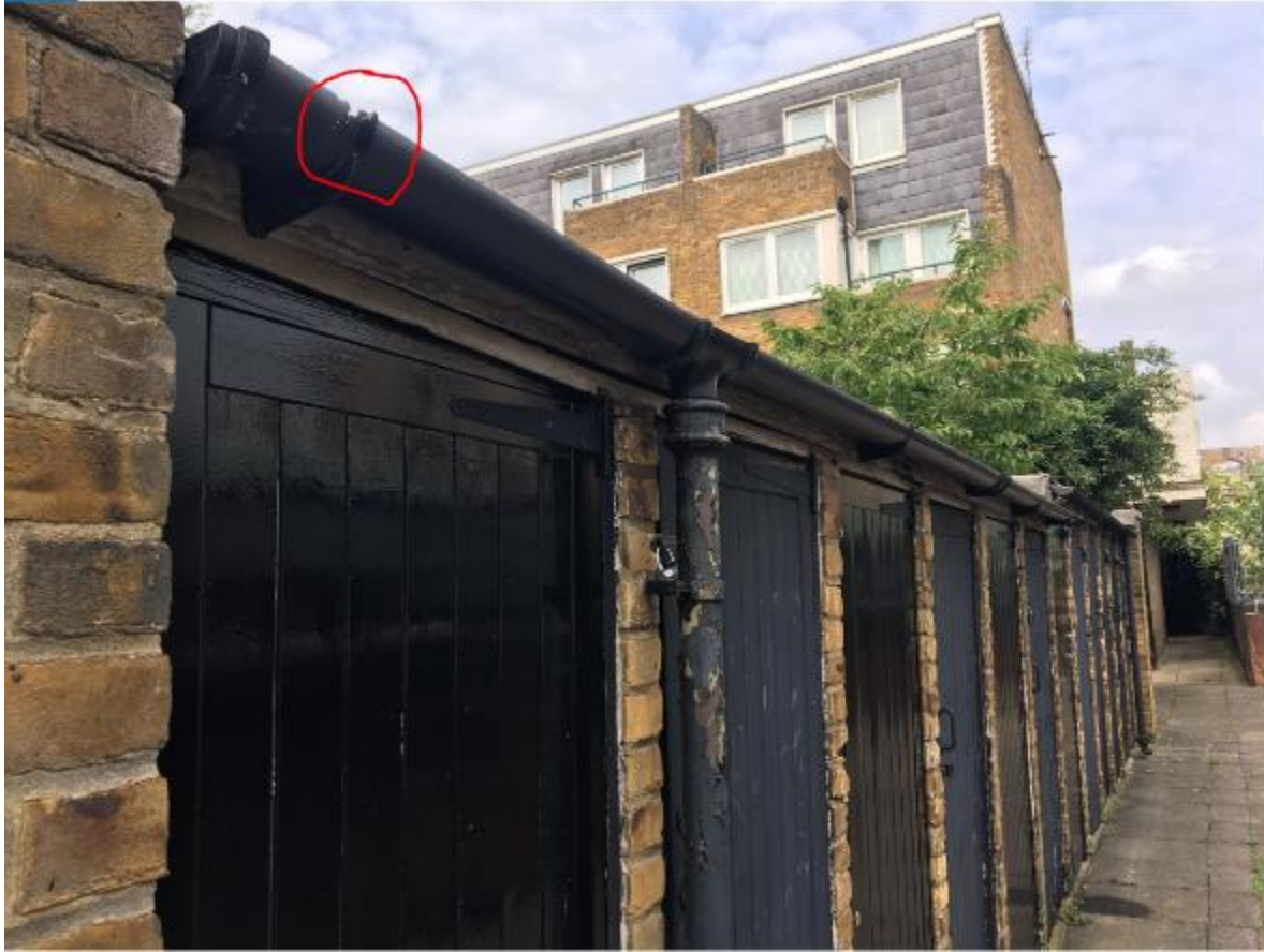
Photo 121. Second pram shed with defective PVCu guttering and failed paintwork to timber fascia and cast-iron downpipe.
