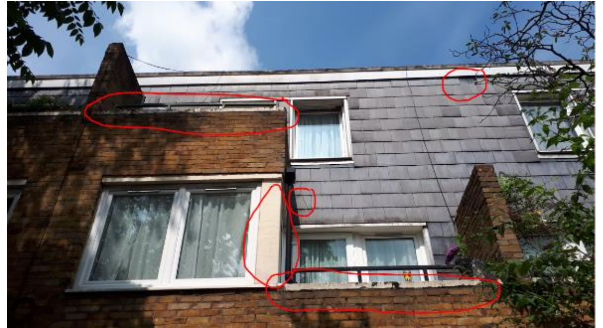
Photo 54. As on the rear elevations of other Blocks there is defective pointing, failing paintwork and the odd missing or broken vertical tile.
