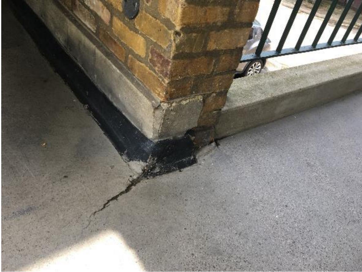
Photo 31. Showing splits to mastic asphalt covering of stairwell landing which could cause penetrating damp when area is washed down.
