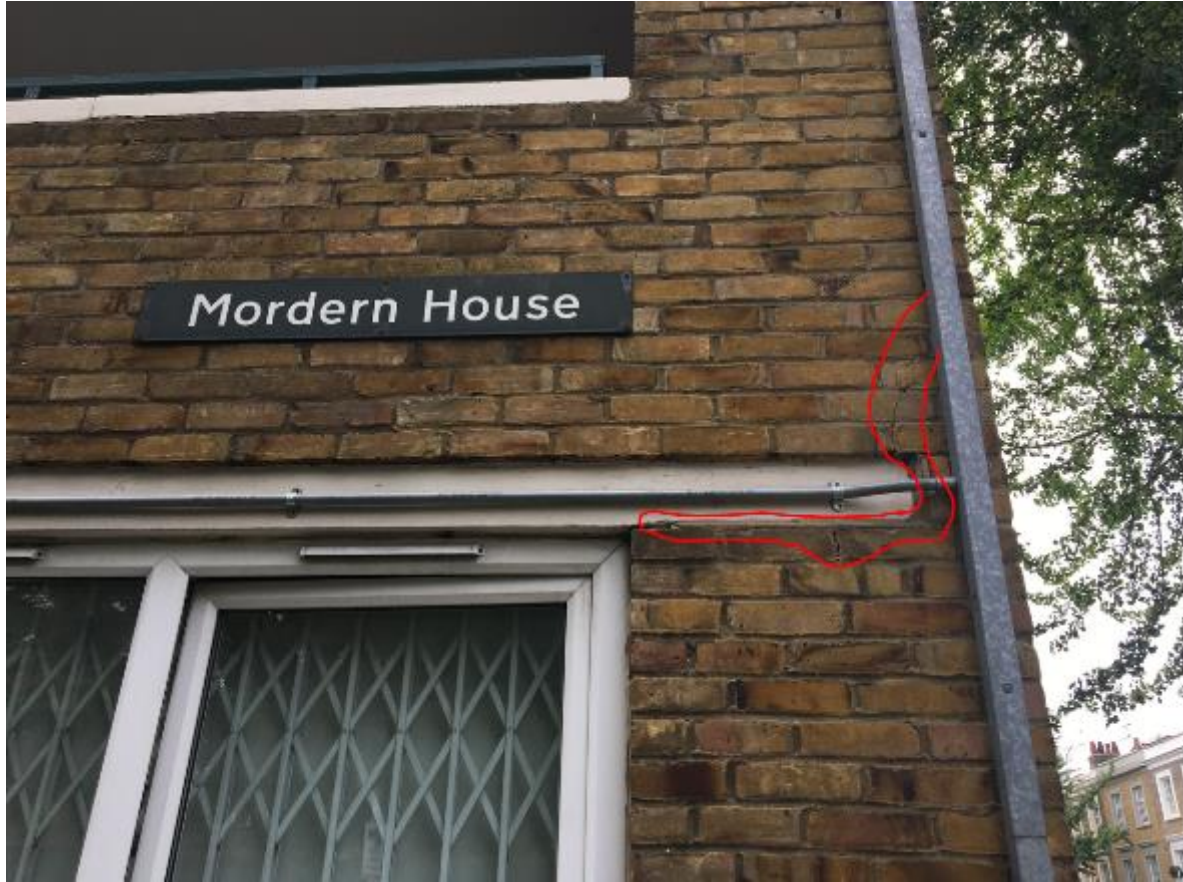
Photo 11. Evidence of localised settlement cracking to front RHS corner of Block. Nearby is a mature Ginkgo tree however, given the hairline width of the cracking it is considered not to be significant enough to warrant monitoring, at least for the present.
