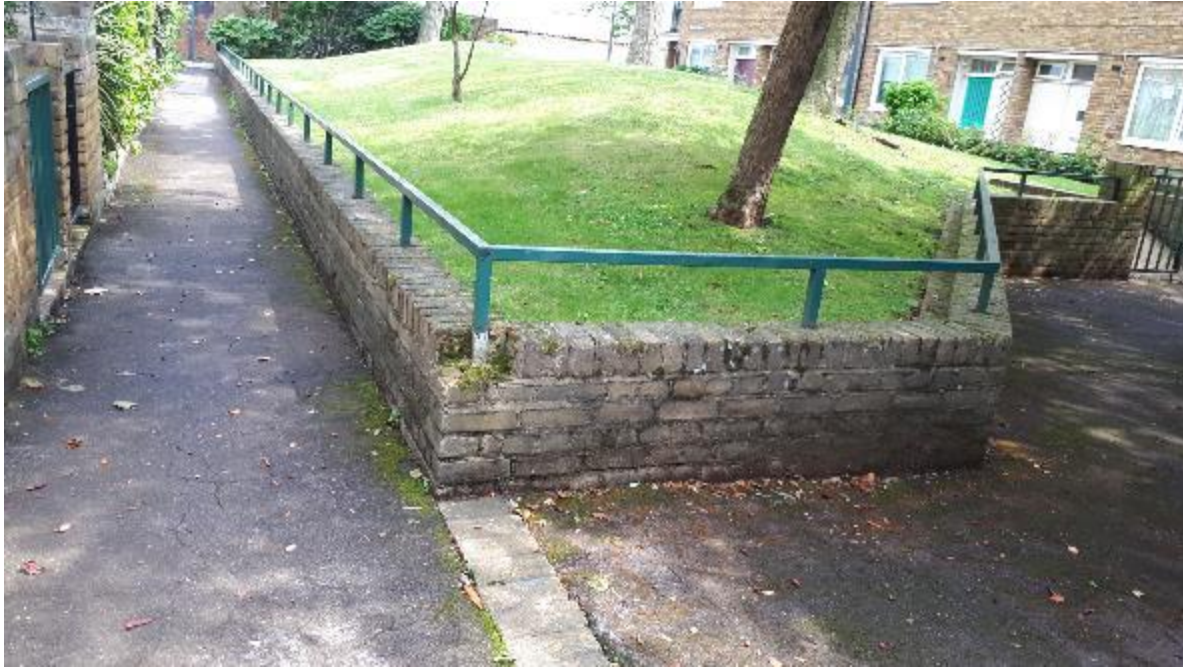
Photo 129. A simple case of replacing a missing brick however, the wall mounted rail needs repainting.
