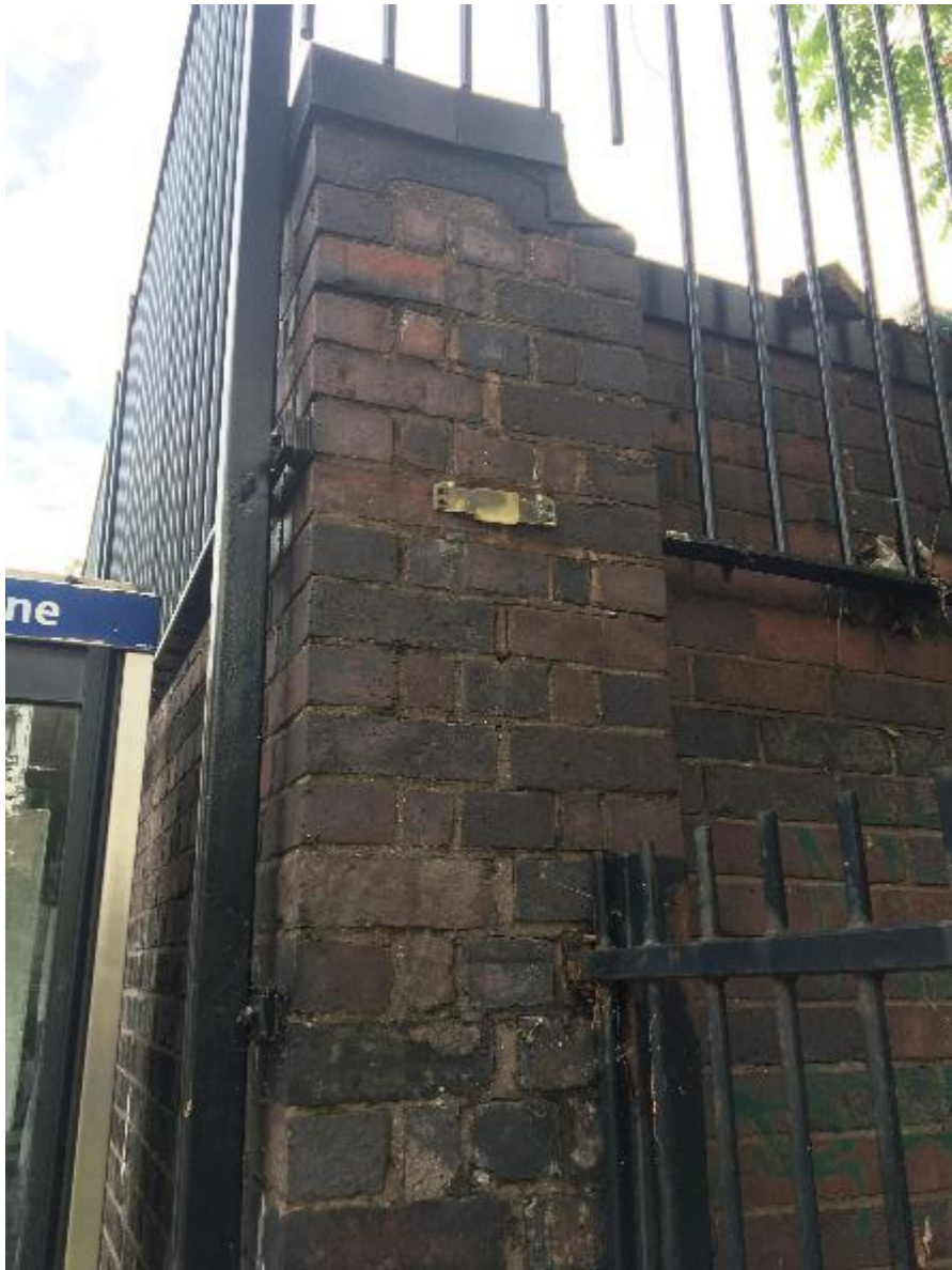
Photo 157. Corner of boundary showing old tell-tale crack monitoring gauge, the surveyor was unsure as to the ownership of this boundary line adjacent the phone box on the corner of Rossmore Rd and Harewood Ave. He was of the opinion that the cracking was not significant, and that any defective brickwork should be re-pointed.
