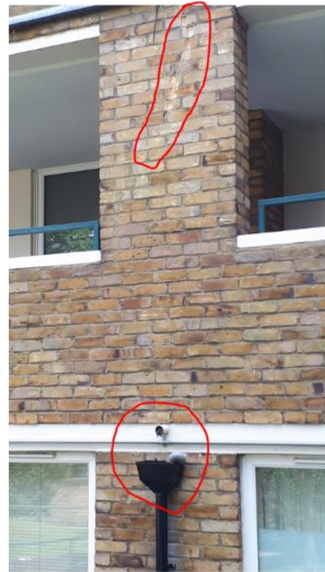
Photo 106. Showing evidence of historic crack repair preparation work at height to façade of four storey Block of Wimborne Hse. Plus, disconnected walkway drain pipe.
