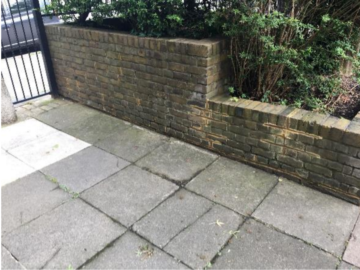
Photo 123. Retaining walls to raised beds showing evidence of previous brickwork repointing although there is more still to do.
