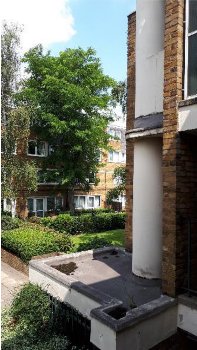
Photo 67. Mastic asphalt covering to bin store roof and bin chute collar roof requires attention.
