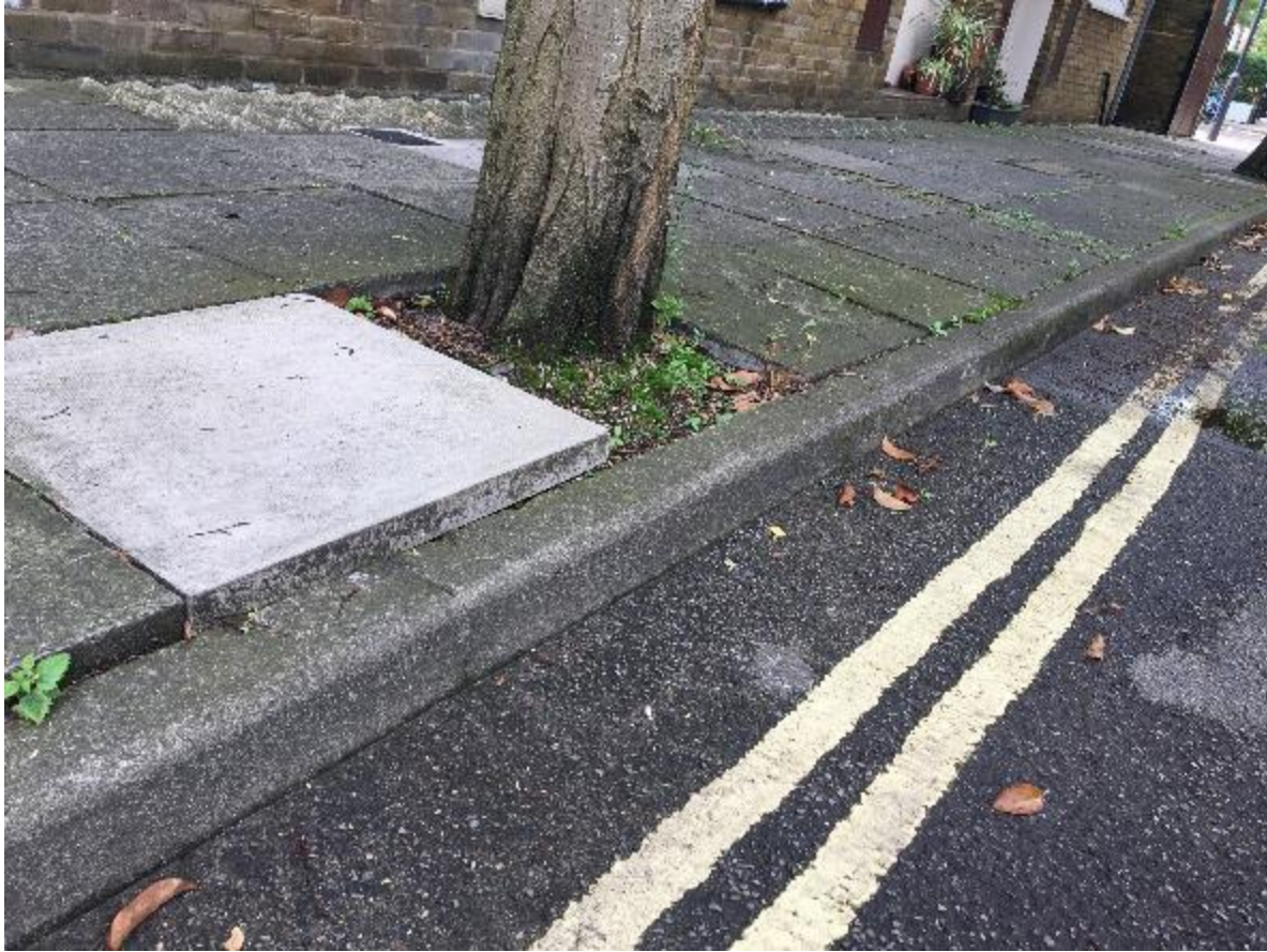
Photo 139. Example of tree root heave and paving displacement.
