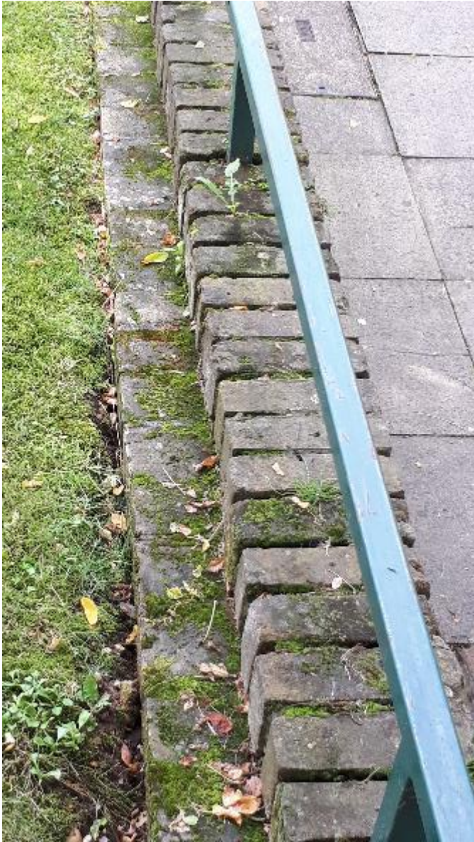
Photo 131. Solider courses require patch repointing.
