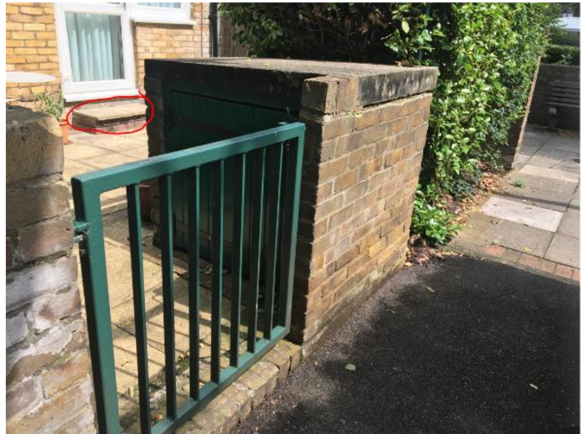
Photo 48. Generally across all four Blocks the decorations to private bin stores and gates is in fair to poor condition. However, the rear entrance door paving slab steps appear unstable.
