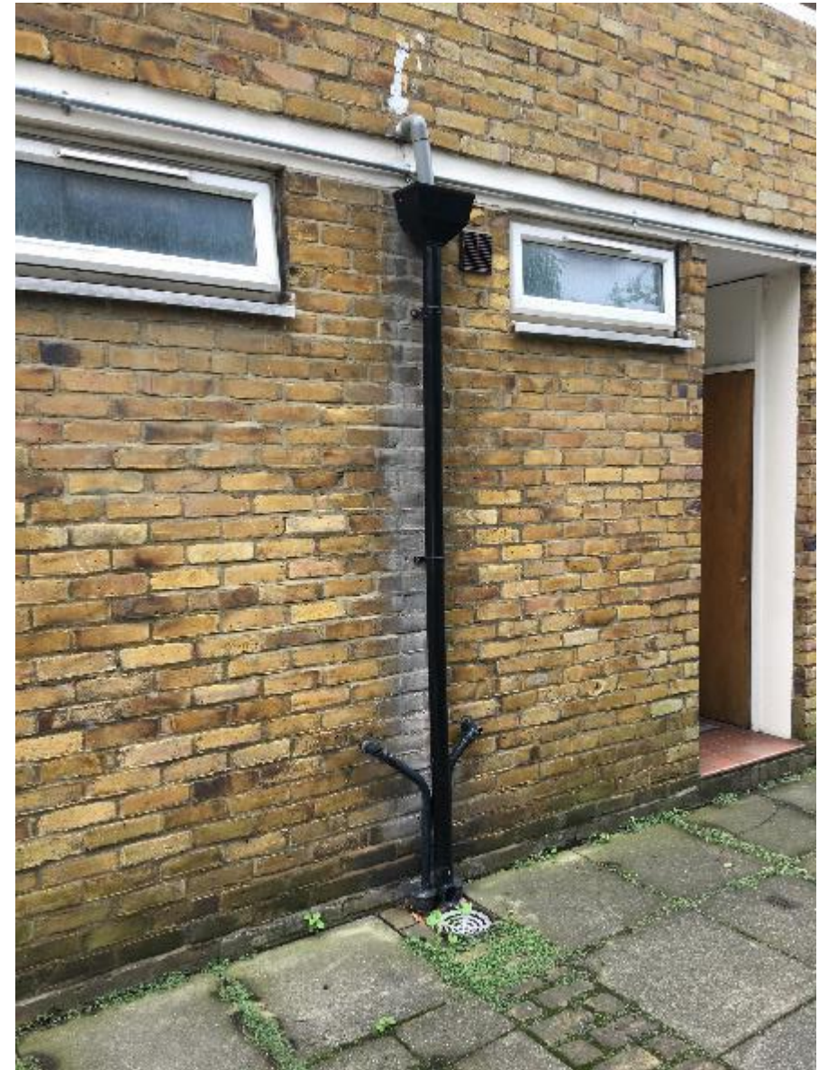
Photo 4. Front elevation rainwater goods serving communal walkways considered to be in good condition as they appear to be relatively new. However, consideration should be given to the removal of historic limescale build-up on the brickwork typically found across the Blocks.
