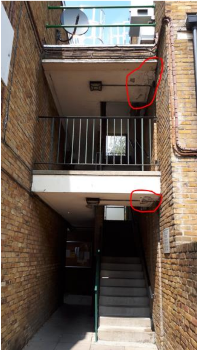
Photo 61. Roof leak to Lascelles' stairwell, downpipe also probably defective as such, leak manifesting below landing.
