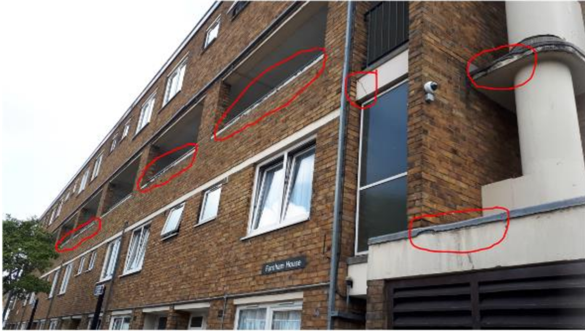
Photo 93. Generic defects to façade of Farnham Hse as found elsewhere across Blocks.
