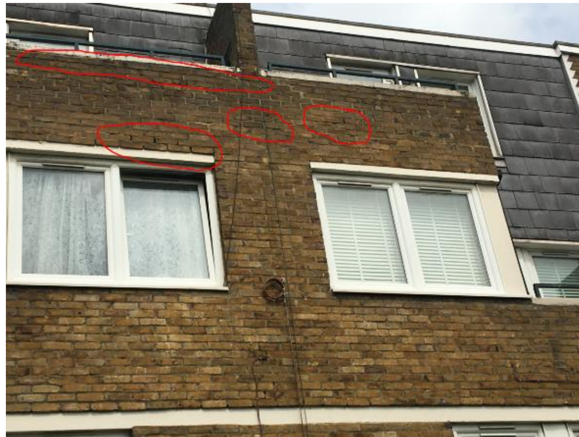
Photo 14. Again on all Blocks, there is defective pointing (red) to private balcony parapets. Note the need to repoint between copings and brickwork.
