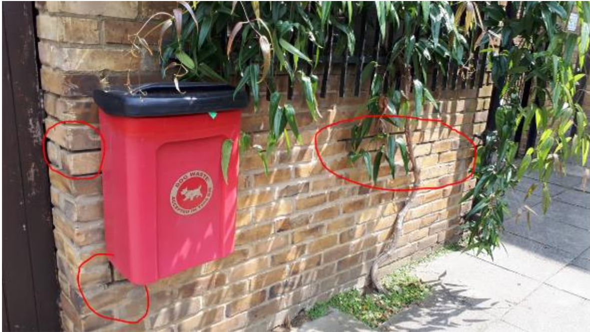
Photo 91. Eroded pointing to bin store.
