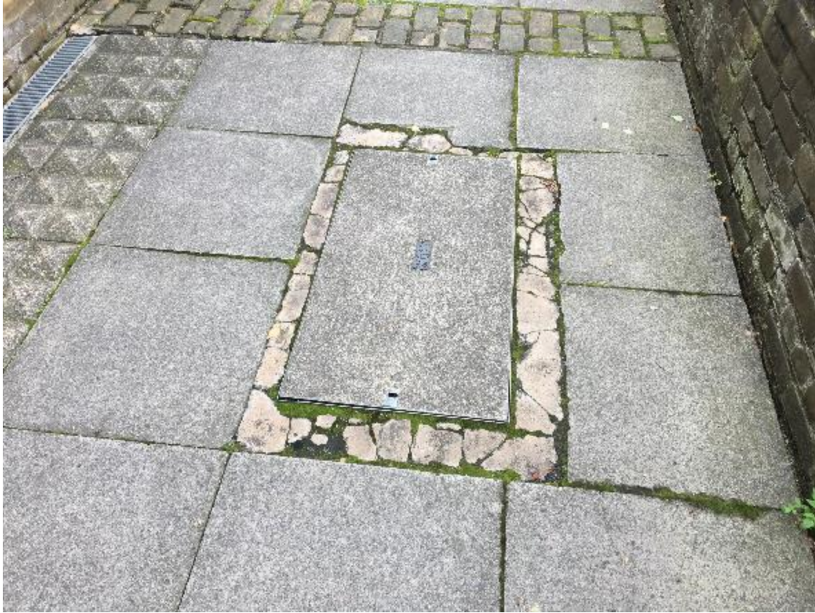
Photo 143. Inspection chamber frame needs re-flaunching.
