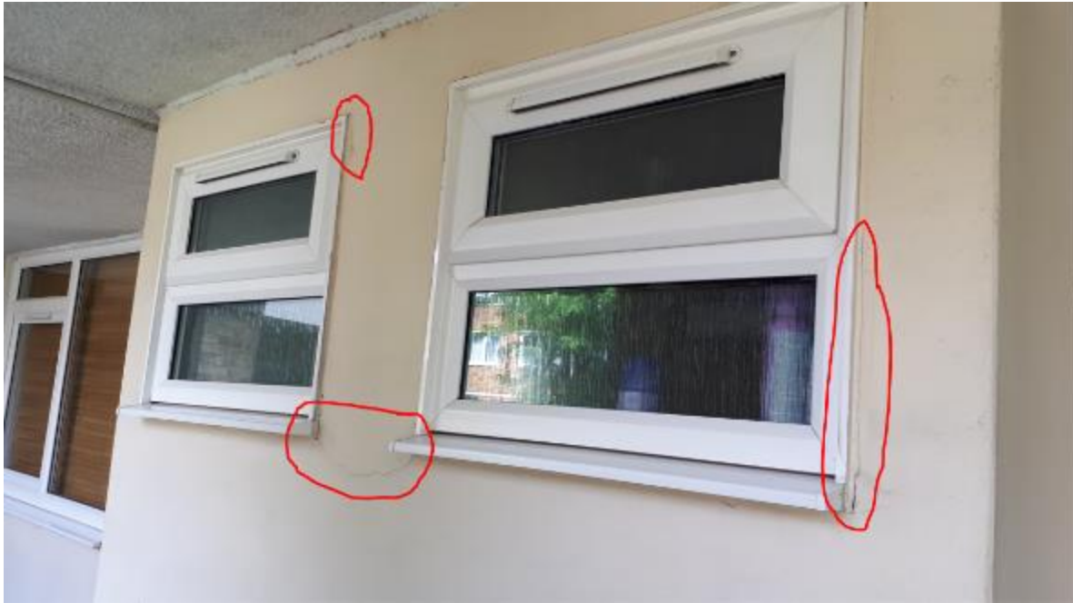
Photo 73. Not of particular concern are the hairline cracks to the rendered finishes, probably caused by the vibration of closing the windows.
