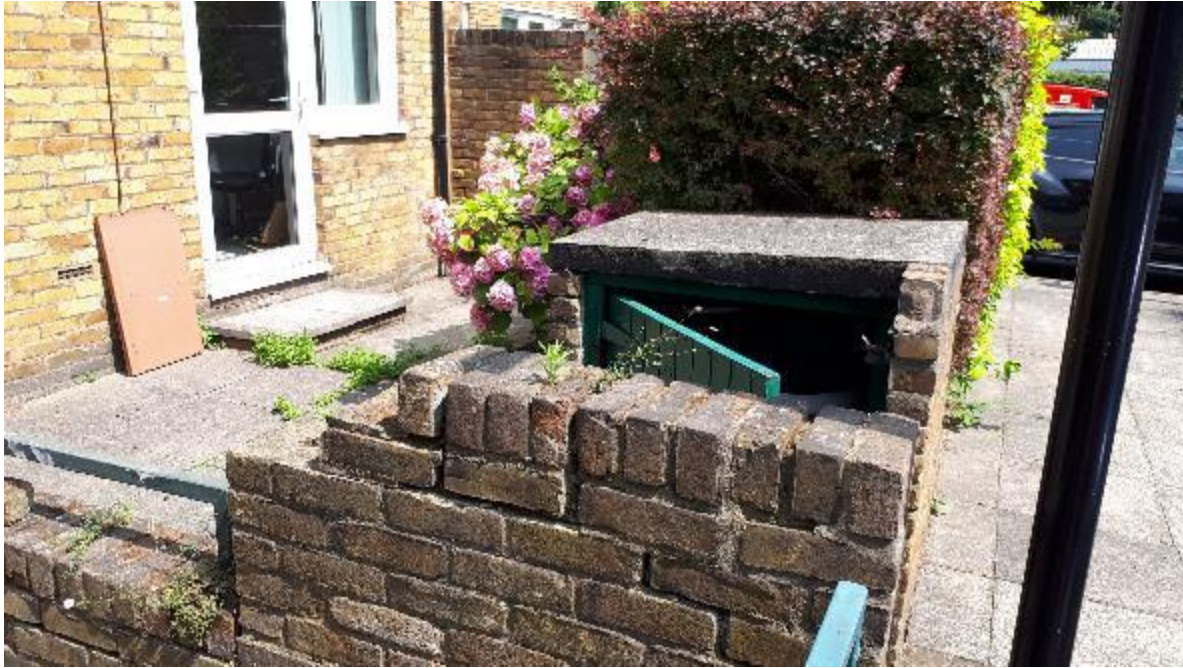
Photo 83. Defective brickwork to rear boundaries of flats, found to a lesser degree elsewhere.
