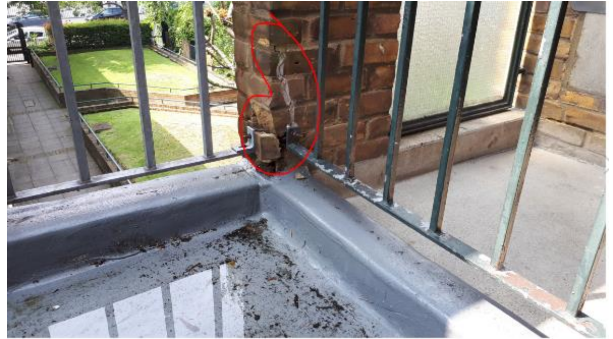
Photo 64. Same roof section, note impact damage to brickwork and evidence of historic repair.
