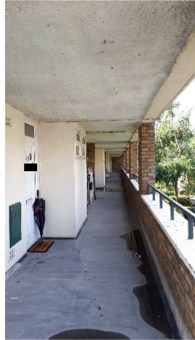
Photo 68. As on other Blocks, the mastic asphalt covering to deck of walkway is in good condition.
