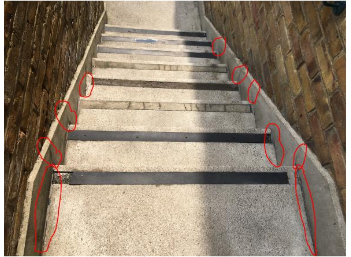
Photo 22. Same steps with highlighted cracking which could conceivably be points of rainwater penetration causing problem below.
