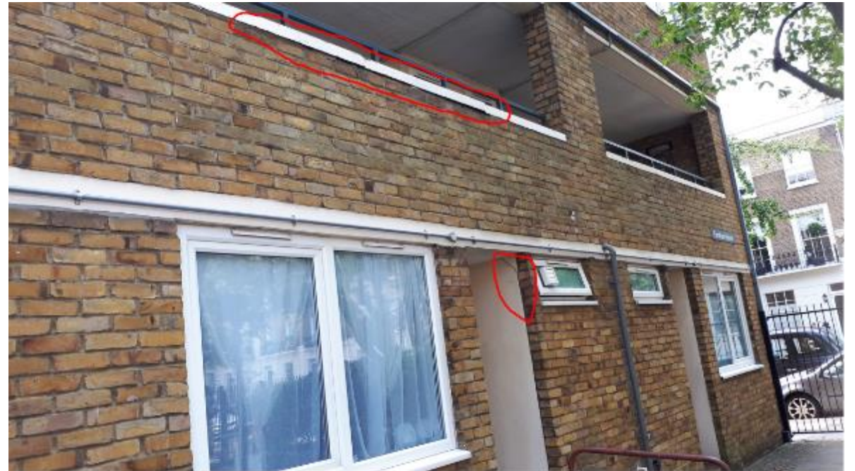
Photo 86. Generic pointing failure beneath copings to walkways as found on other Blocks. There is minor settlement cracking lower down.
