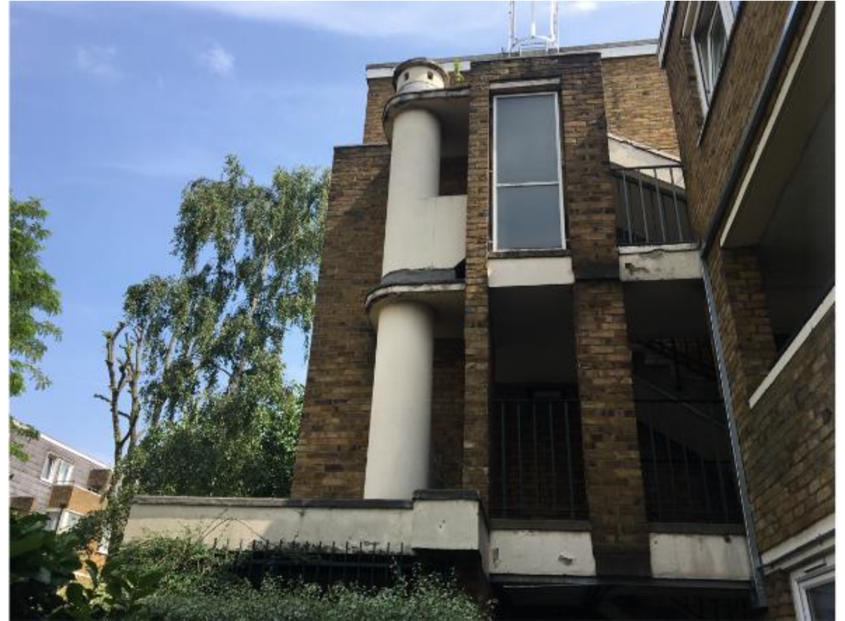
Photo 60. Again, failing decorations and self-seeded vegetation which if not removed will disturb brickwork.
