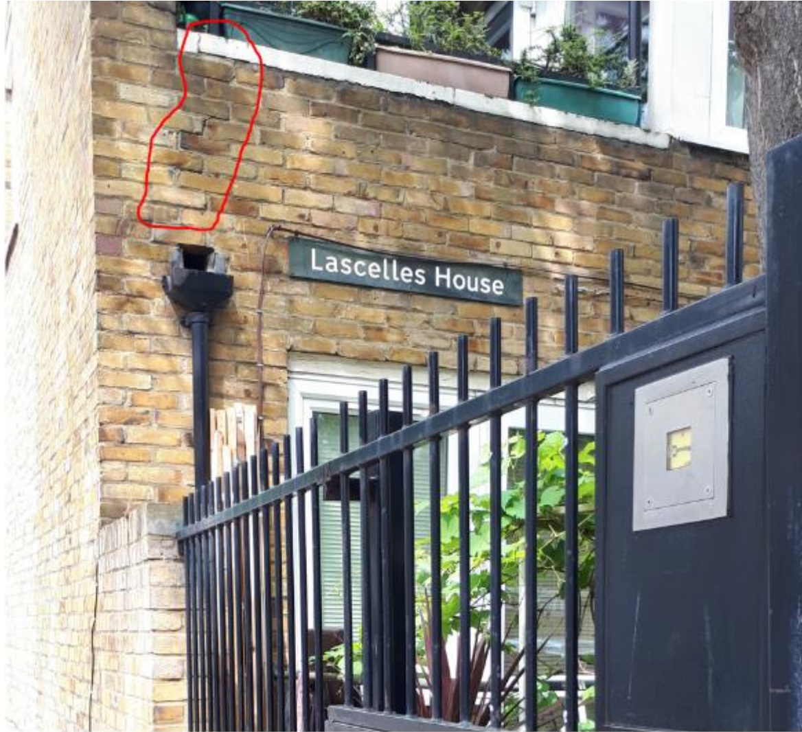
Photo 53. Similar cracking as found to the rear of Mordern Hse here, one could simply repoint the brickwork.
