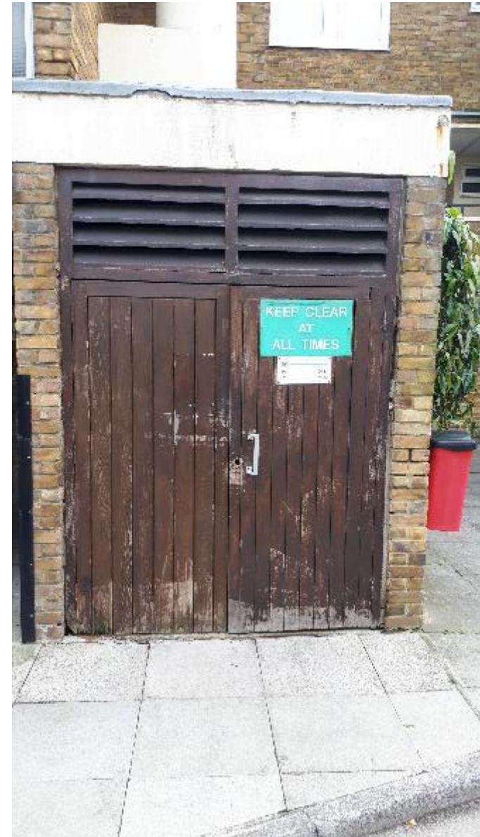
Photo 92. Repair and redecoration of bin store doors required at Farnham Hse.
