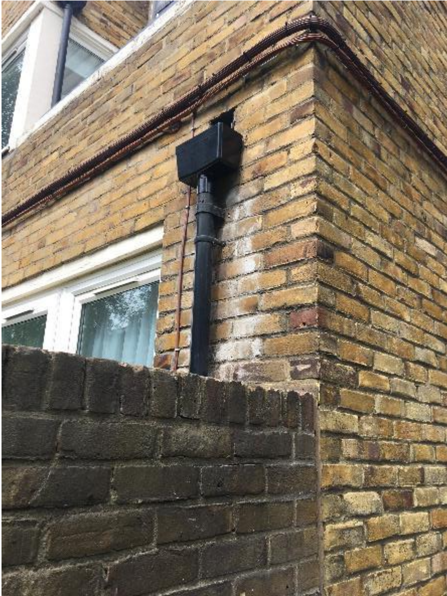
Photo 7. Example as per previous photo.
