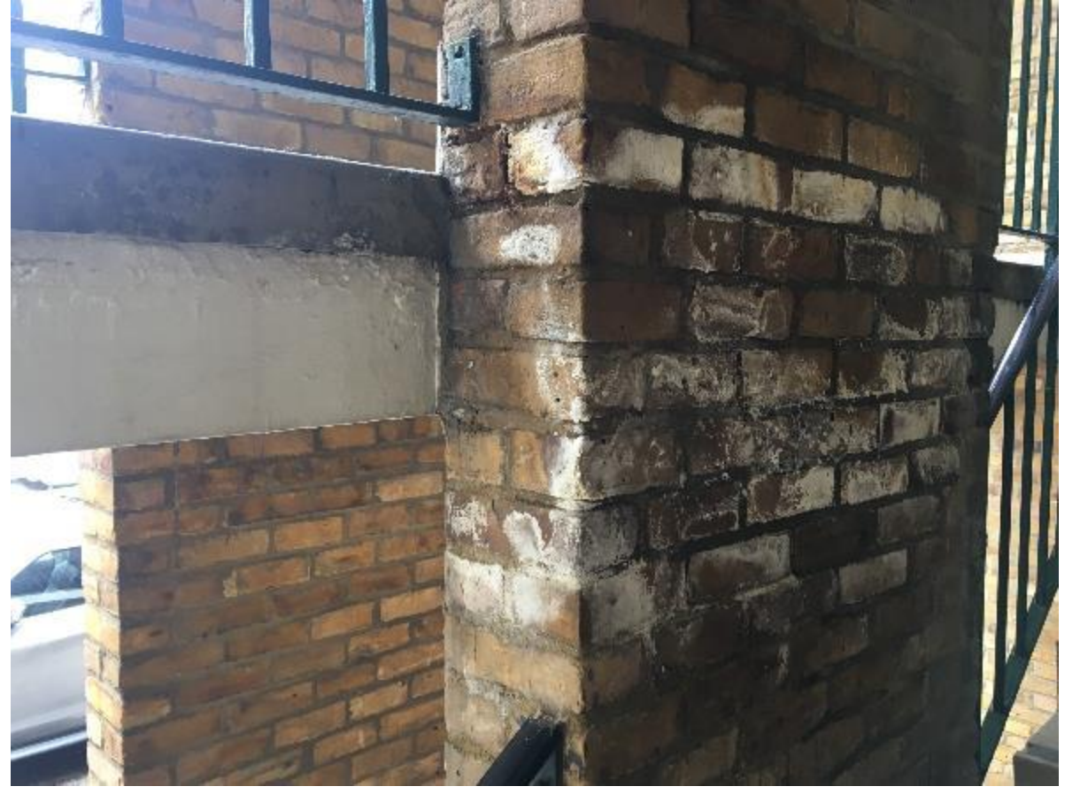
Photo 30. Evidence of damp in the form of hygroscopic salts on surface of stairwell pillar.
