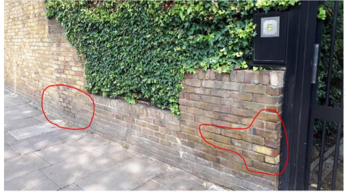
Photo 162. Here it is simply a case of re-pointing defective sections of brickwork.
