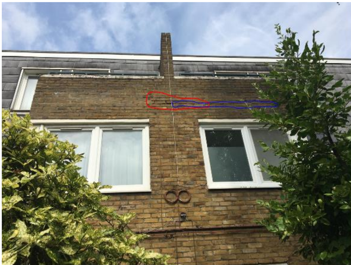
Photo 13. A generic defect found on all Blocks of localised defective pointing (red) to 2 nd flr rear private balcony parapet, note exposed DPC (blue).
