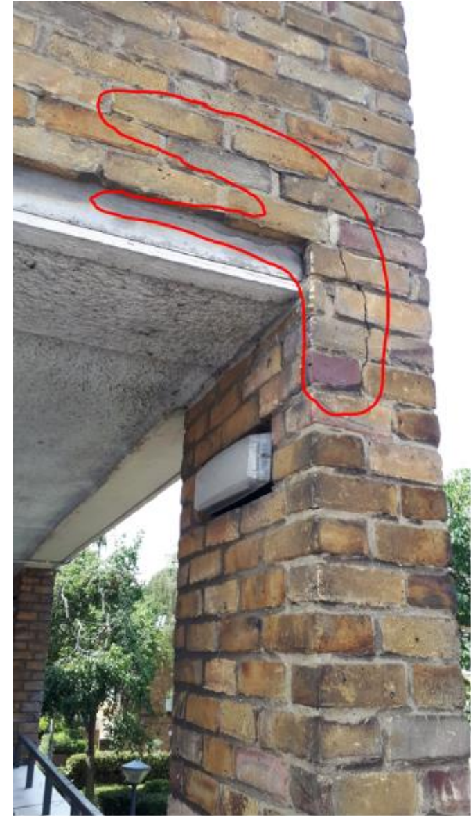
Photo 82. Same set of stairs, Lascelles Hse, movement and/or thermal cracking, concrete abutting brickwork, possibly exacerbated by nearby trains.
