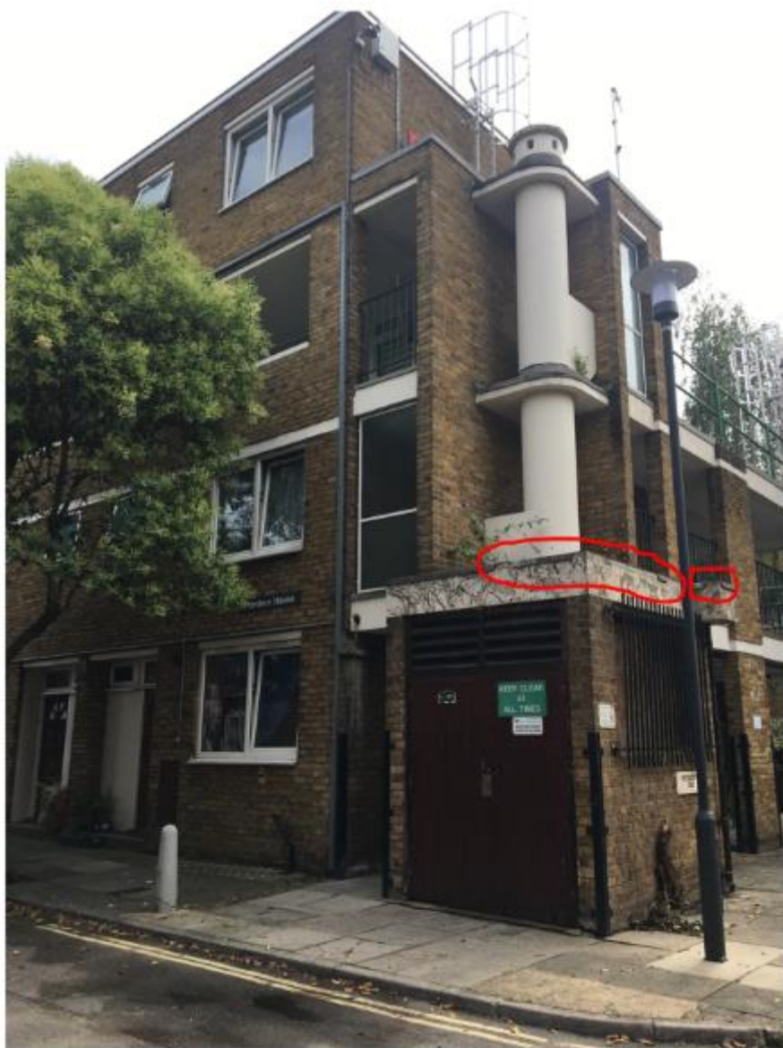
Photo 25. Showing open stairwell with bin store and chute. Note the failing mastic asphalt covering and self-seeded vegetation.
