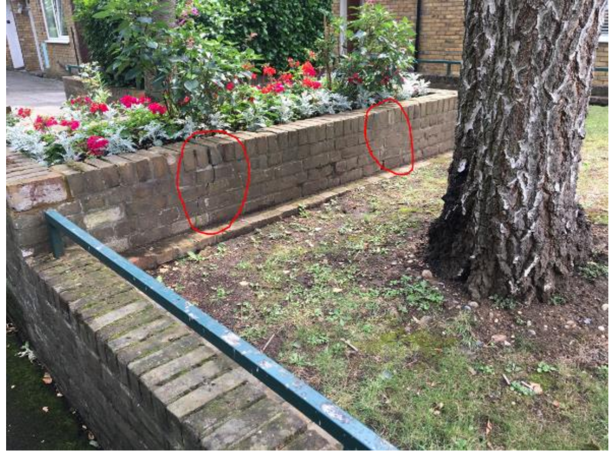
Photo 128. Simply repointing as and when required is probably the most inexpensive and practical way of tackling the ongoing problem of movement cracking. The use of HeliBars could simply shift the cracking elsewhere along the walls.
