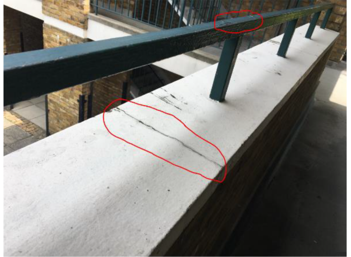
Photo 40. Generic to all Blocks is failing paintwork to wall mounted parapet guard rails as well as, paintwork to copings. The copings are once weathered, shedding rainwater onto the walkways plus, the joints are failing resulting in water ingress and subsequent concrete failure where drip grooves are sometimes choked with mortar exacerbating the defect.
