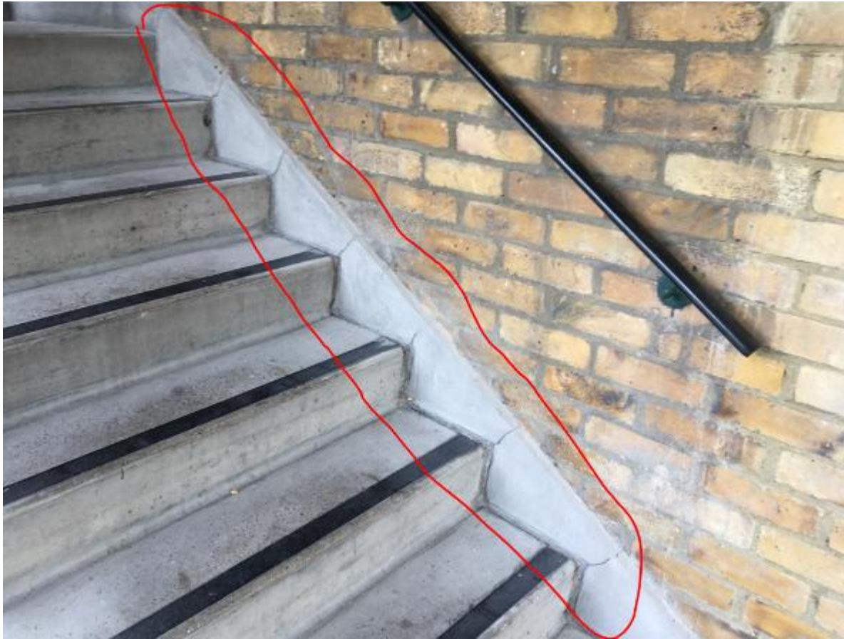
Photo 33. Showing cracking to wall stringer of stairs which may be the cause of moisture penetration below when treads are being washed down.
