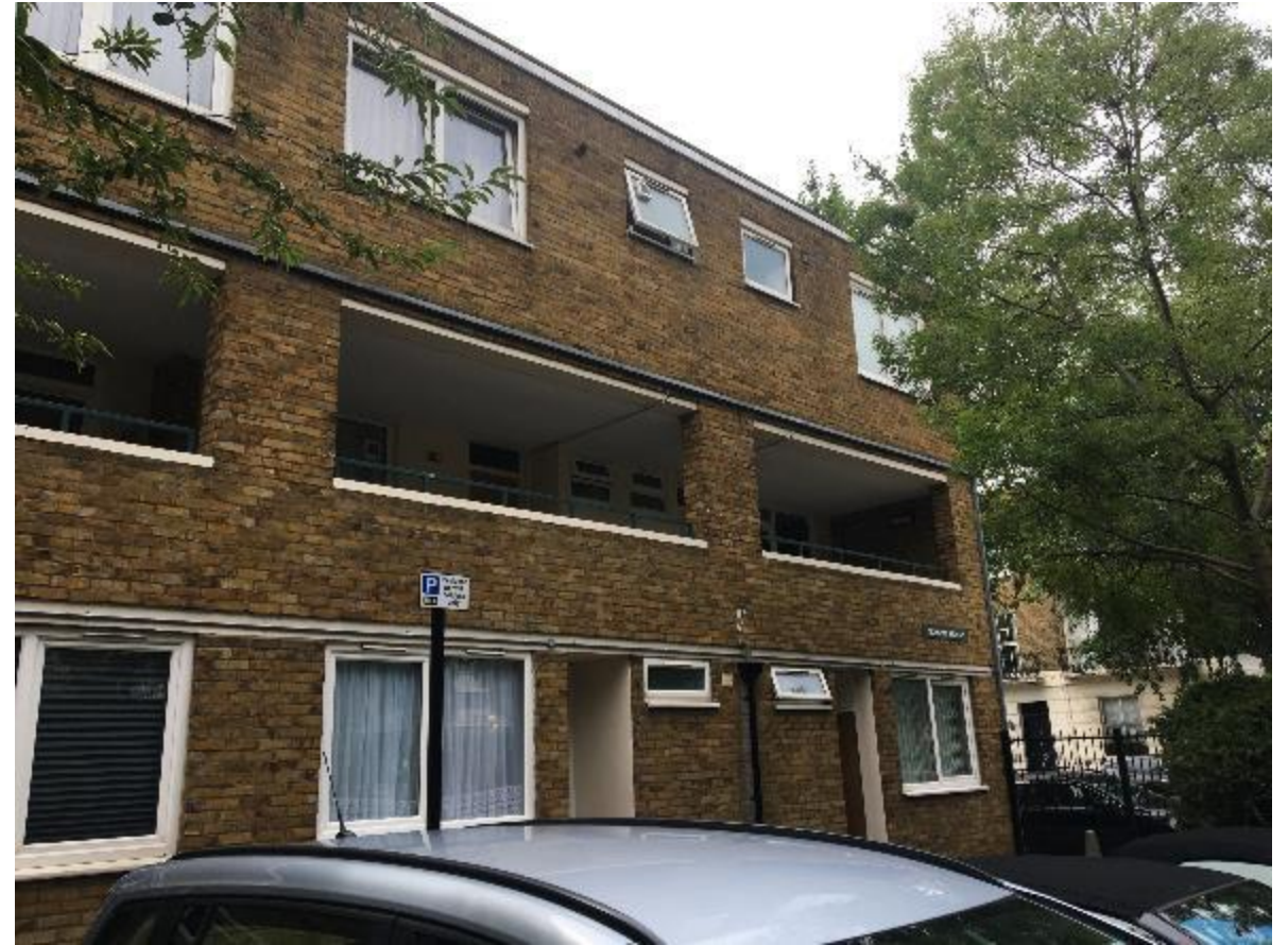
Photo 2. Front elevation fascia boards, the Council's brief states that no roofing works are planned in its next cyclical decoration programme. However, at Modern Hse despite the assumed PVCu or possibly aluminium powder coated boards to the main roofs being in good condition, consideration should be given to their cleaning.
