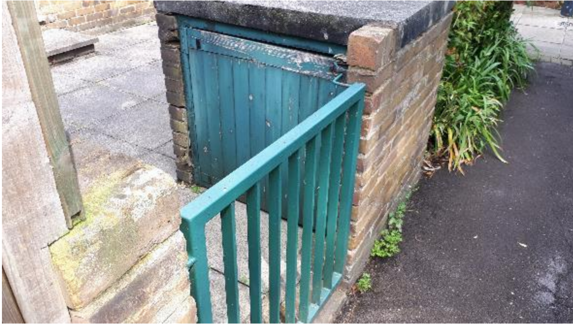
Photo 101. As on other Blocks, failing paintwork to bin stores and gates.
