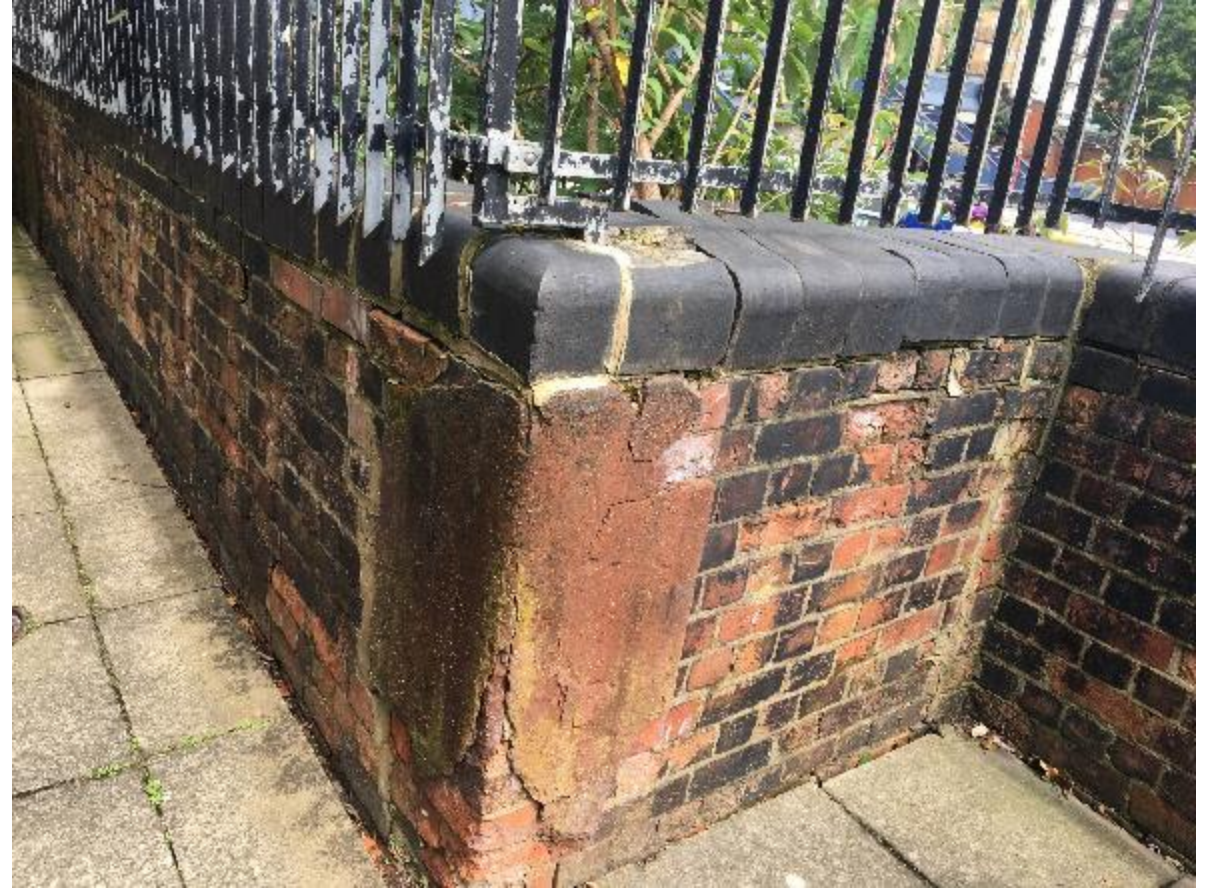
Photo 168. Same boundary wall this time showing displaced copings.
