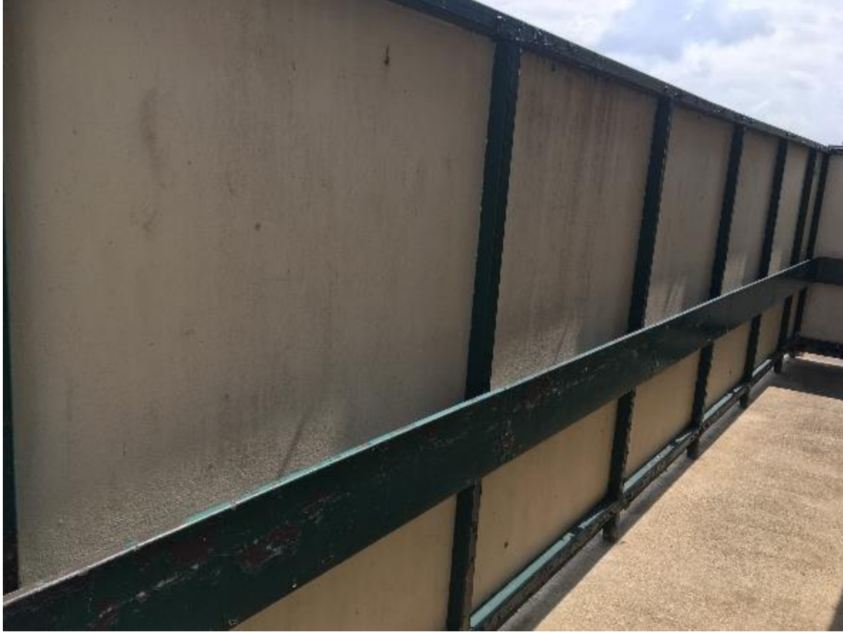
Photo 19. Failed paintwork to guarding of same steps.
