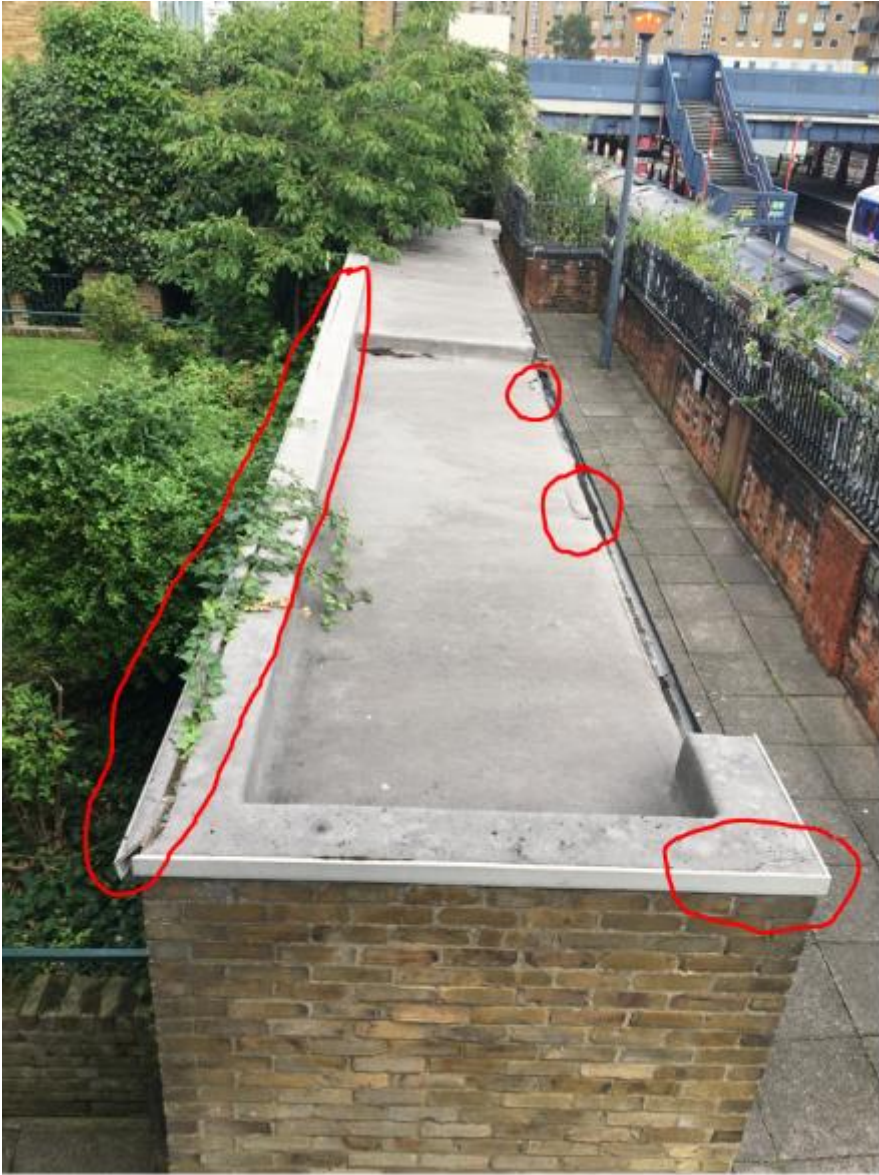
Photo 119. Second pram shed with defective mastic asphalt roof covering.
