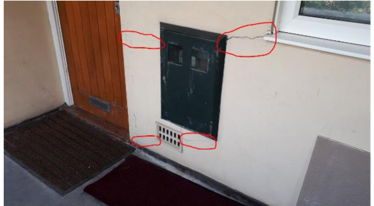
Photo 74. Again, most likely to be vibration, movement cracking.
