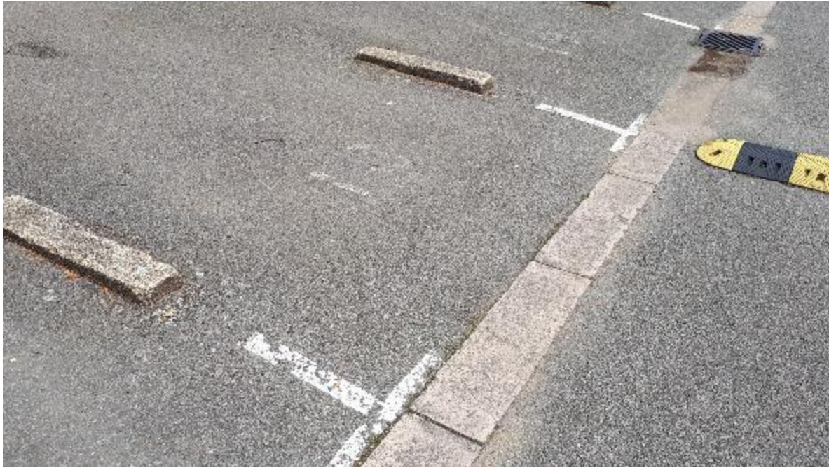
Photo 155. Same carpark where number markings to bays and lines are worn.
