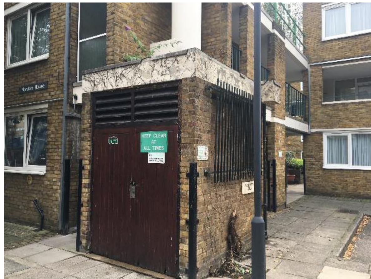
Photo 26. Close-up of bin store, doors of which in need of repair and redecoration.
