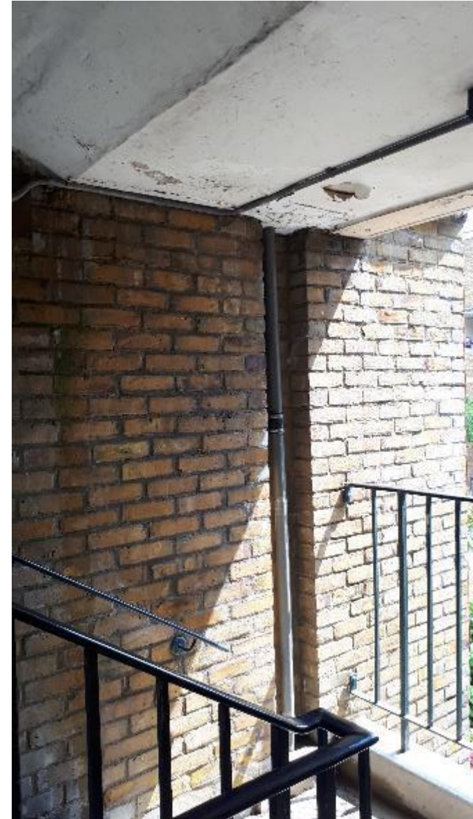
Photo 66. Again as shown in photo 61, water damage to decorations of stairwell soffit.
