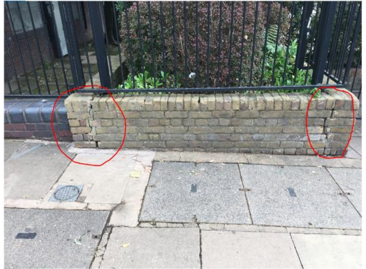
Photo 158. Showing movement cracking to ends of dwarf boundary wall. Given the wall is adjacent a public footpath and the width of the cracking plus evidence of failed historic pointing repairs, the Council should consider using HeliBars to stitch the brick work as a belt and braces approach to rectifying the defect.
