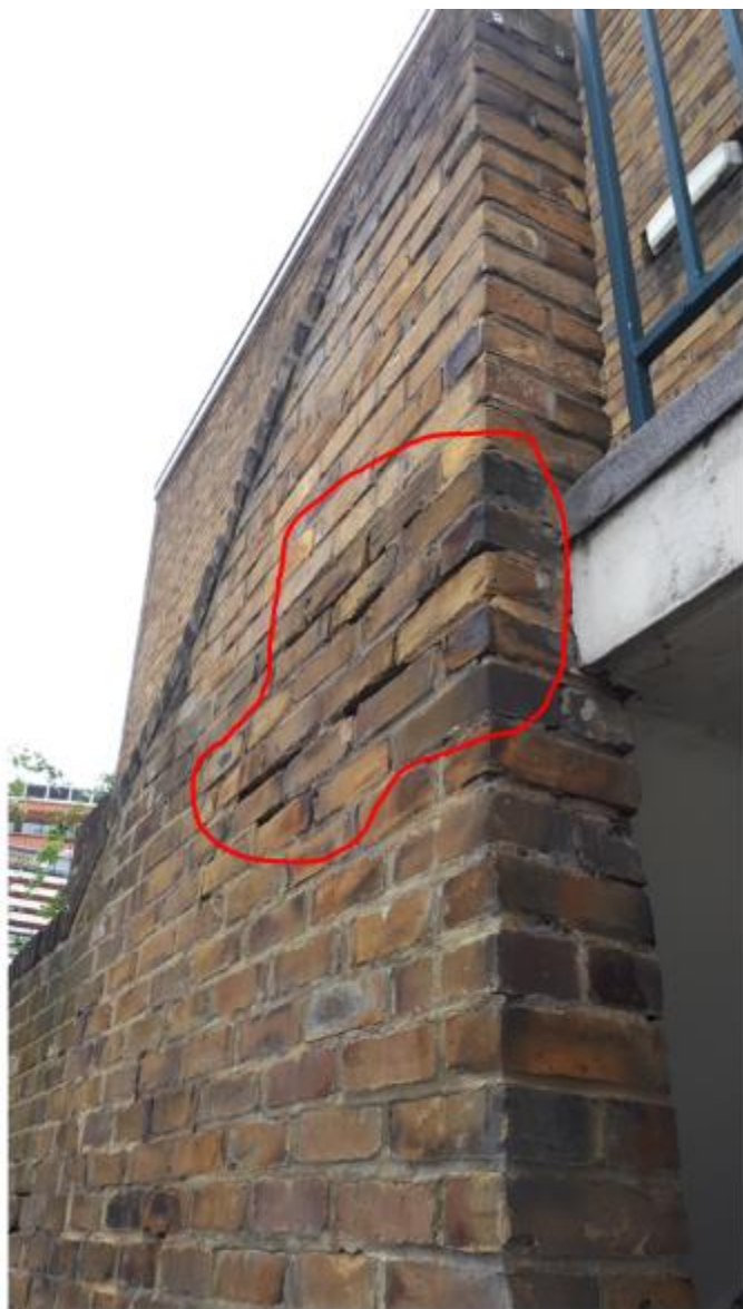
Photo 109. Same stairs and as on other Blocks the pointing is defective.
