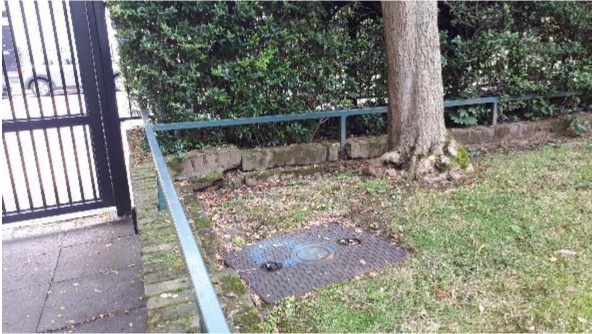
Photo 127. Here one would have to either re-bed the displaced brickwork or demolish the wall as there is a boundary wall behind it. What is a concern, is likely tree root damage to below ground drainage.
