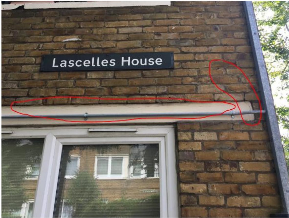
Photo 51. Lascelles House, where as at Mordern Hse, the cracking to the front elevation corner adjacent Harewood Avenue is considered to be of minor significance.
