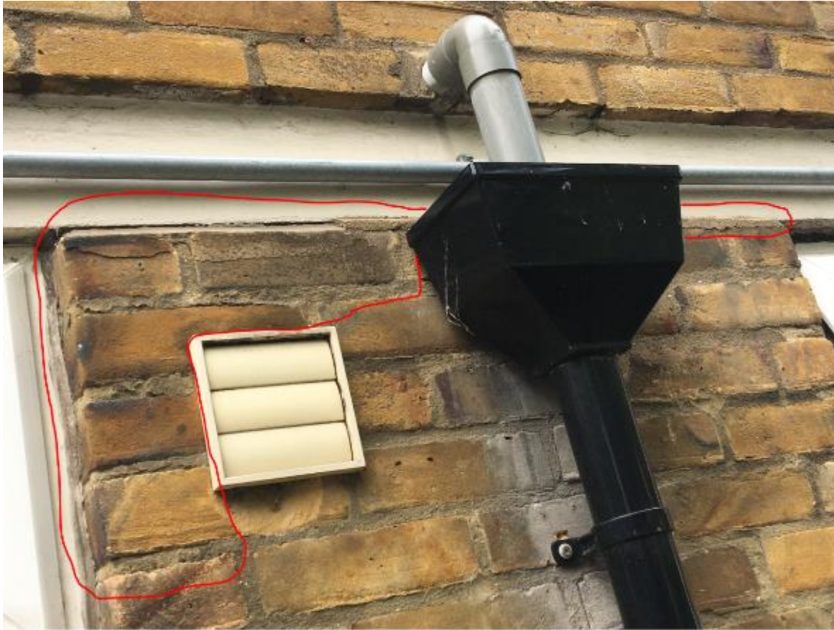
Photo 15. Likely to be a generic defect found on all Blocks of localised defective pointing to top corners of grd flr front window openings where there appears to be some minor, assumed thermal movement cracking.
