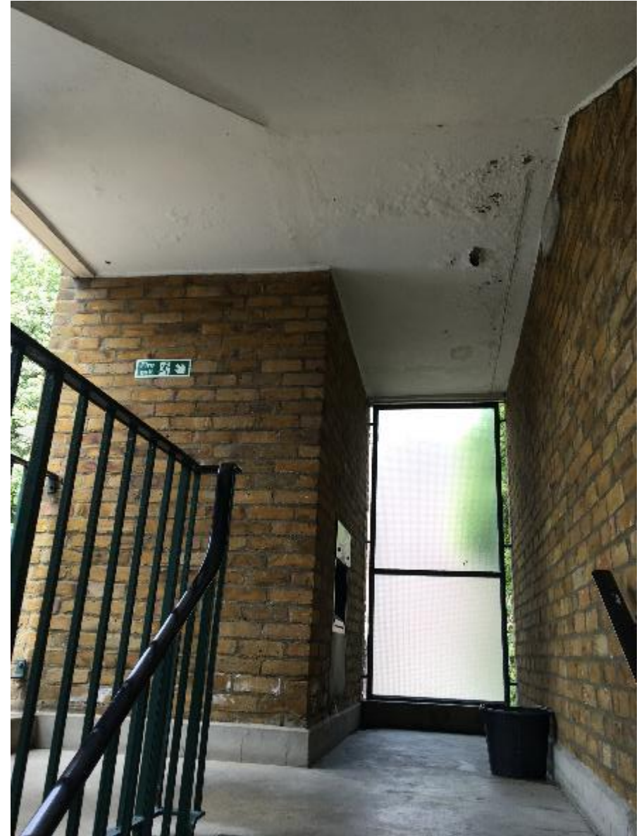
Photo 32. Evidence of penetrating damp to roof soffit of Mordern Hse stairwell. Note the bucket of water used to wash the floor or might be there to catch a roof leak.
