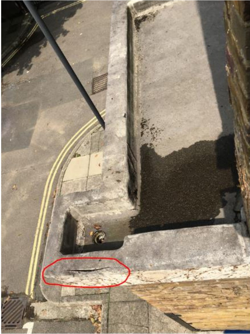
Photo 27. Defective mastic asphalt covering to bin store roof.
