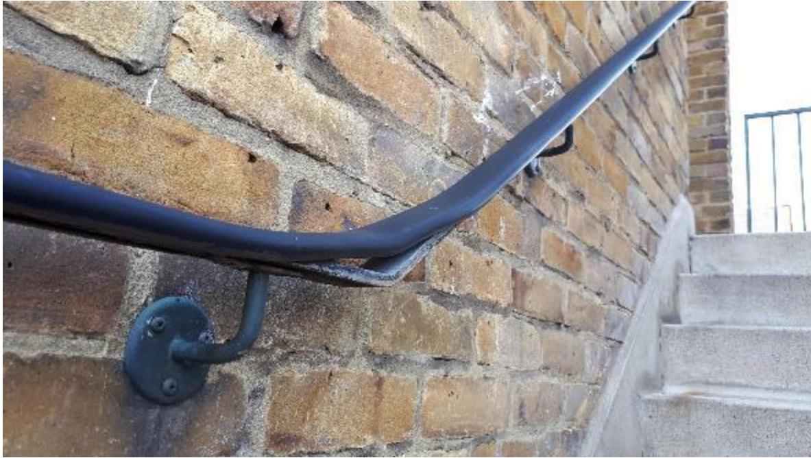
Photo 81. Same set of stairs, handrail grip debonding.
