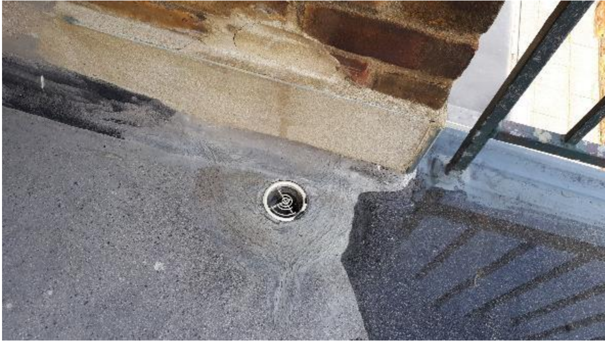
Photo 75. Grilles to walkway outlets broken across all Blocks.
