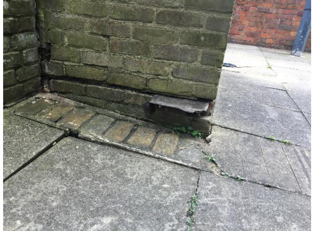
Photo 122. Second pram shed with defective DPC.
