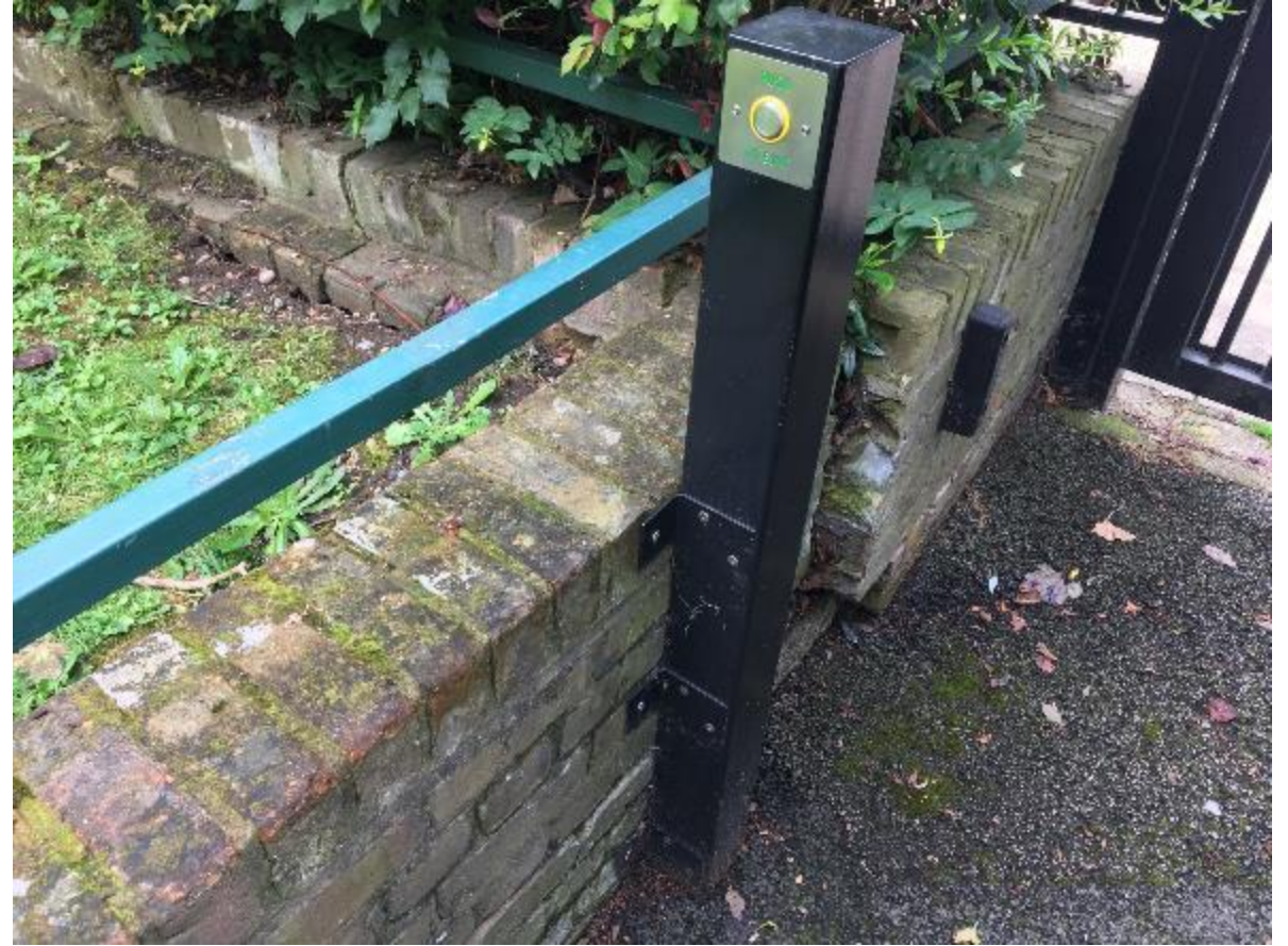
Photo 130. An example of just how much the retaining walls have been displaced.
