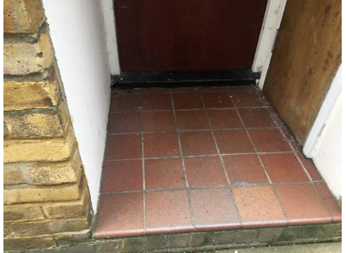
Photo 42. Ground floor front entrance steps to flats in good condition however despite being under cover, the decorations to entrance and store doors are tired.
