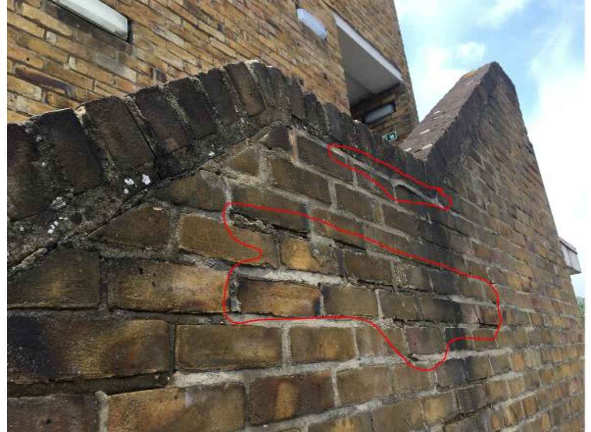
Photo 16. A generic defect found across all Blocks of localised failed pointing (red) to parapet guarding of steps adjacent railway. Note the black staining of the brickwork corresponding to the change in slope of the solid course coping.
