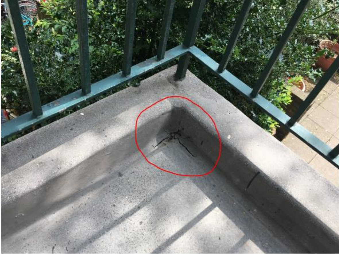
Photo 35. Mastic asphalt repair required to communal stairs landing, note failing paintwork to guarding.
