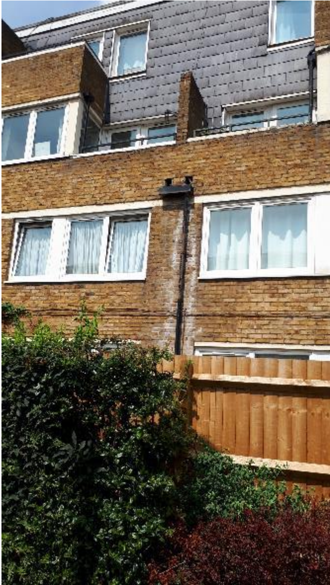
Photo 55. As on other Blocks, there is failing paintwork to rear elevation RWGs and subsequent corrosion of hoppers.
