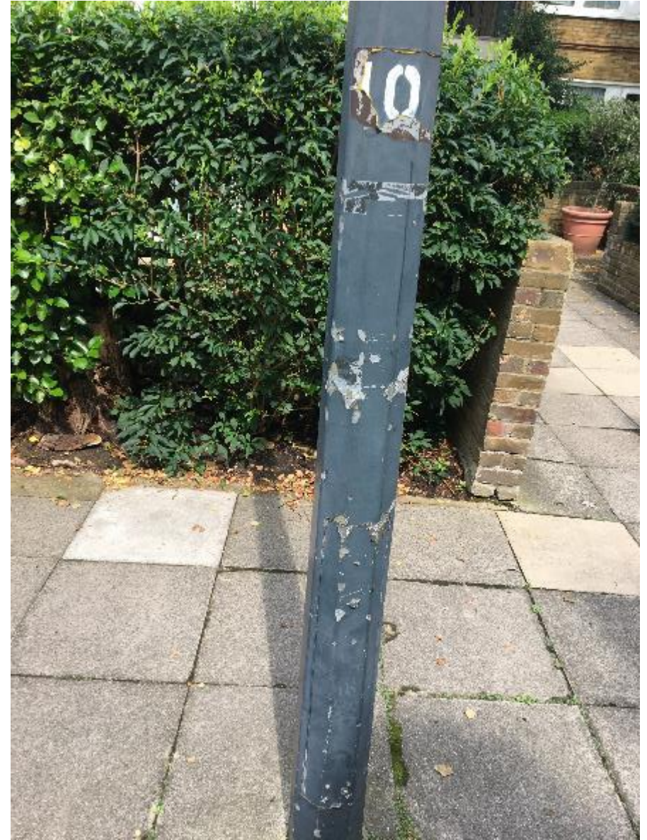
Photo 150. Paintwork to lamp post failing.
