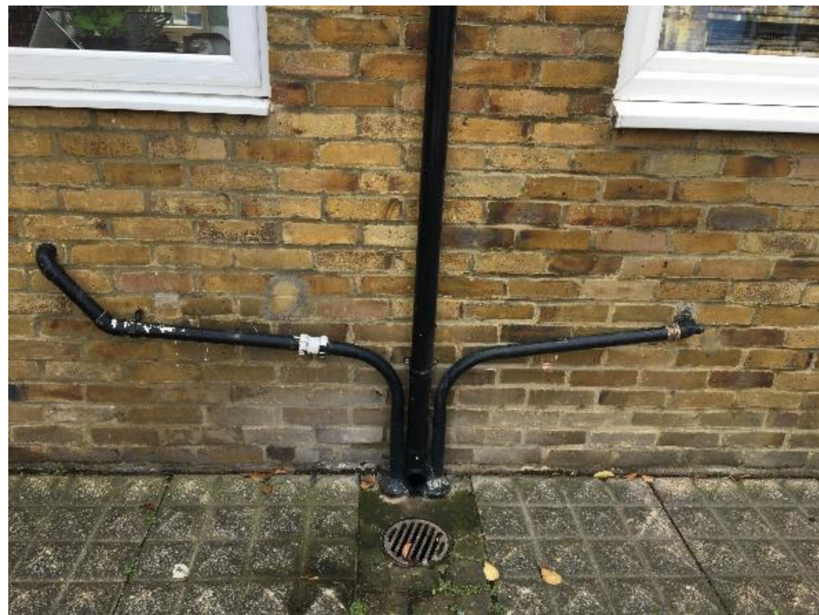
Photo 44. Generally, the paintwork to waste water pipes is failing.
