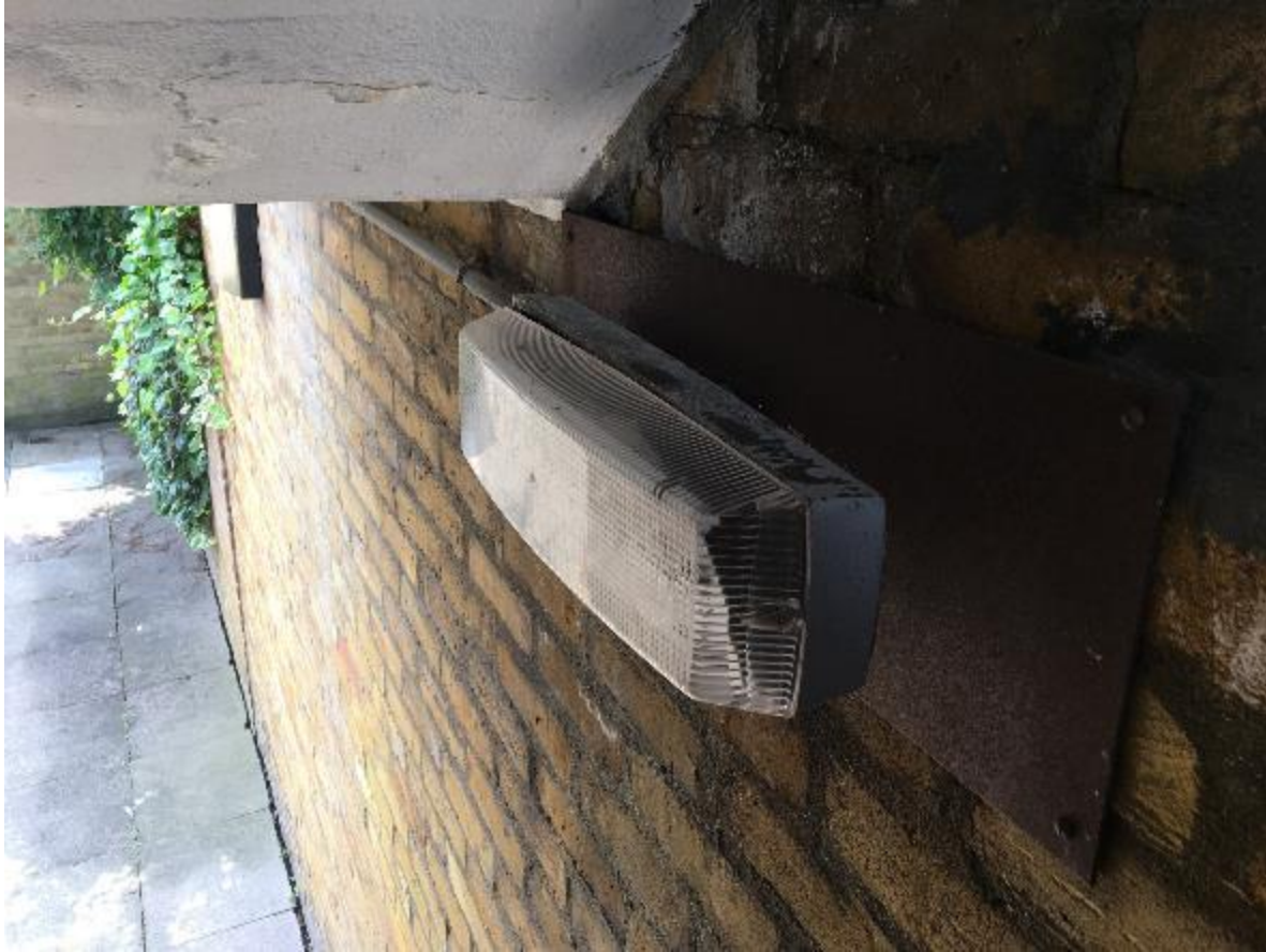
Photo 21. Same defect on other side, here the skirting above is defective.
