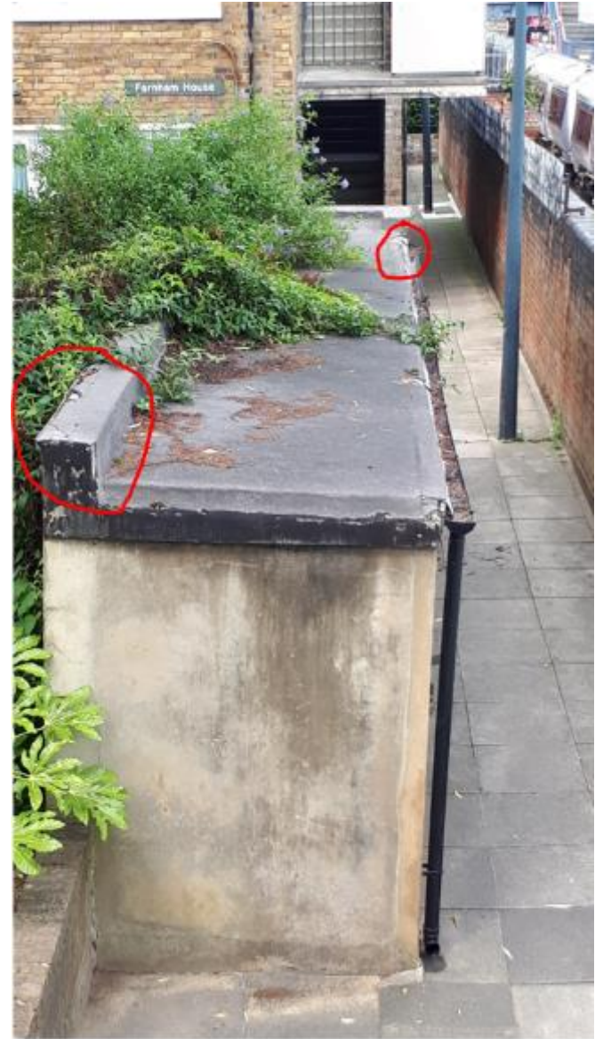
Photo 116. Same pram shed with defective mastic asphalt roof covering.
