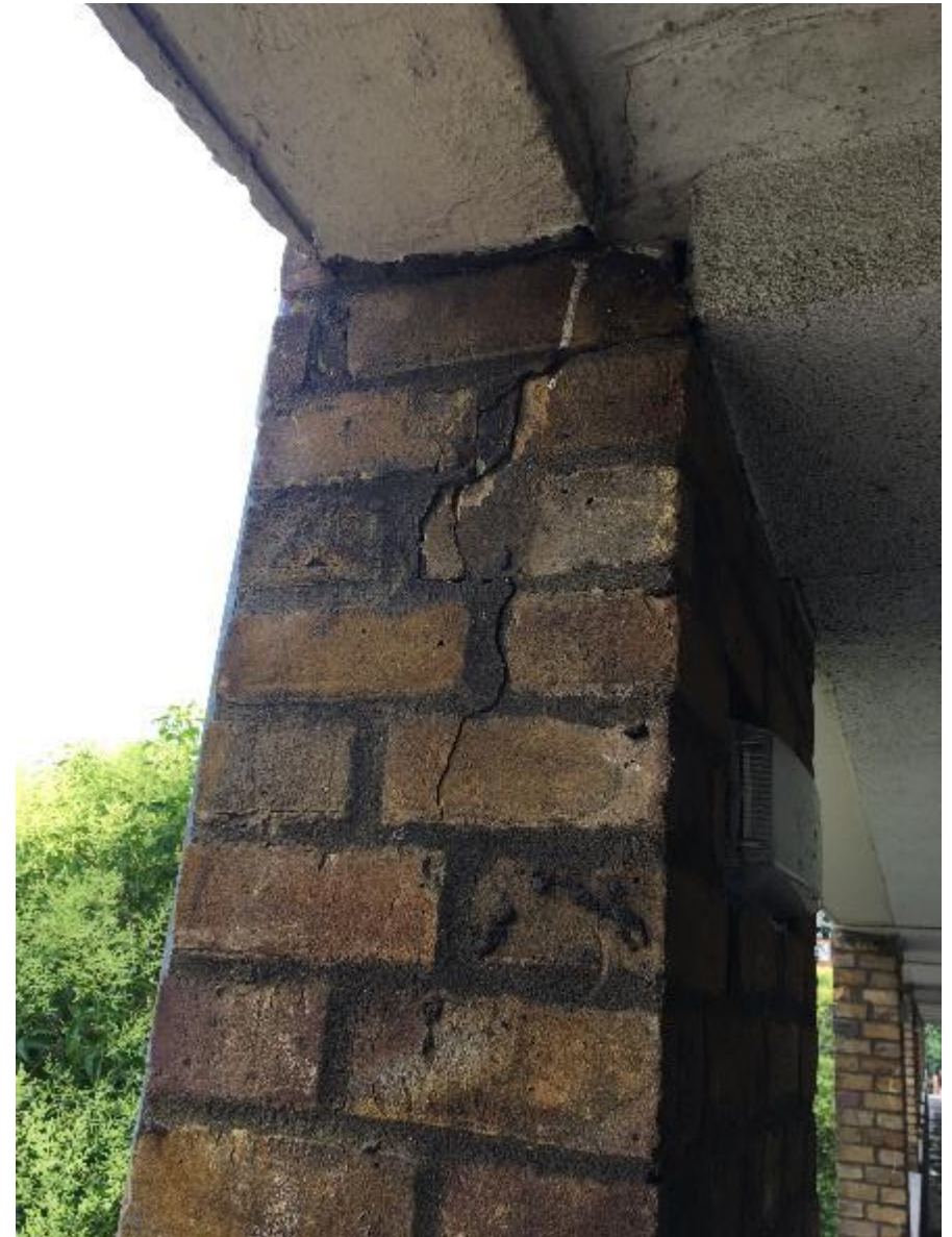
Photo 24. Same defect, different pillar.
