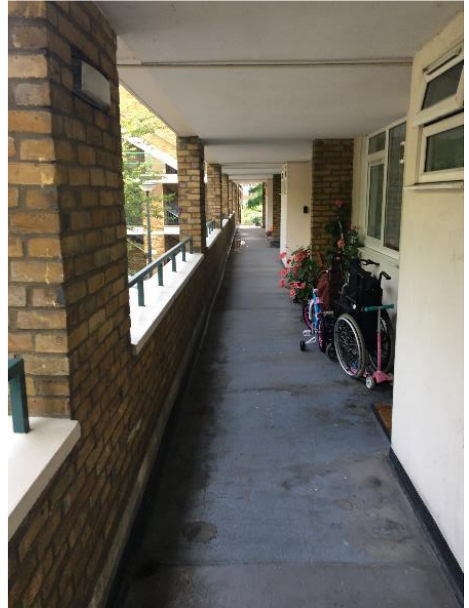
Photo 38. Example of a typical communal walkway where generically across all Blocks the decorated soffits and flat frontages are in fair condition exhibiting the usual signs of fair wear and tear. The mastic asphalt covering to the decks are in fair to good condition although surface coatings are worn.
