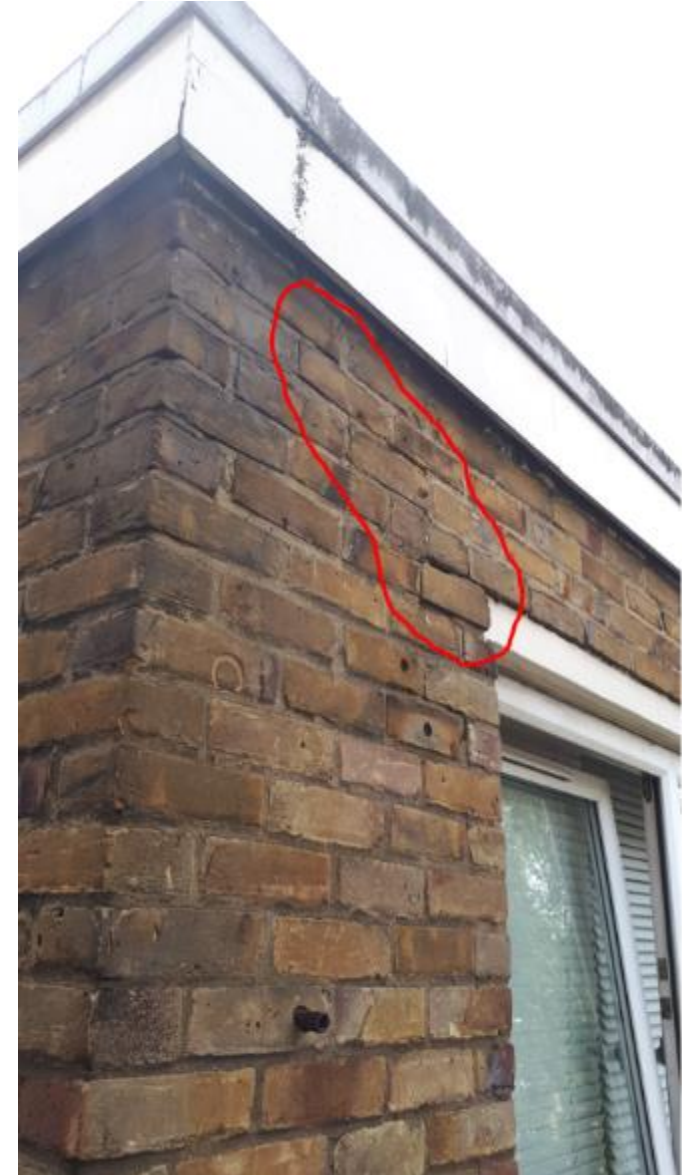
Photo 58. Front elevation as seen from communal stairwell landing showing defective pointing as well as failing paintwork to timber fascia.
