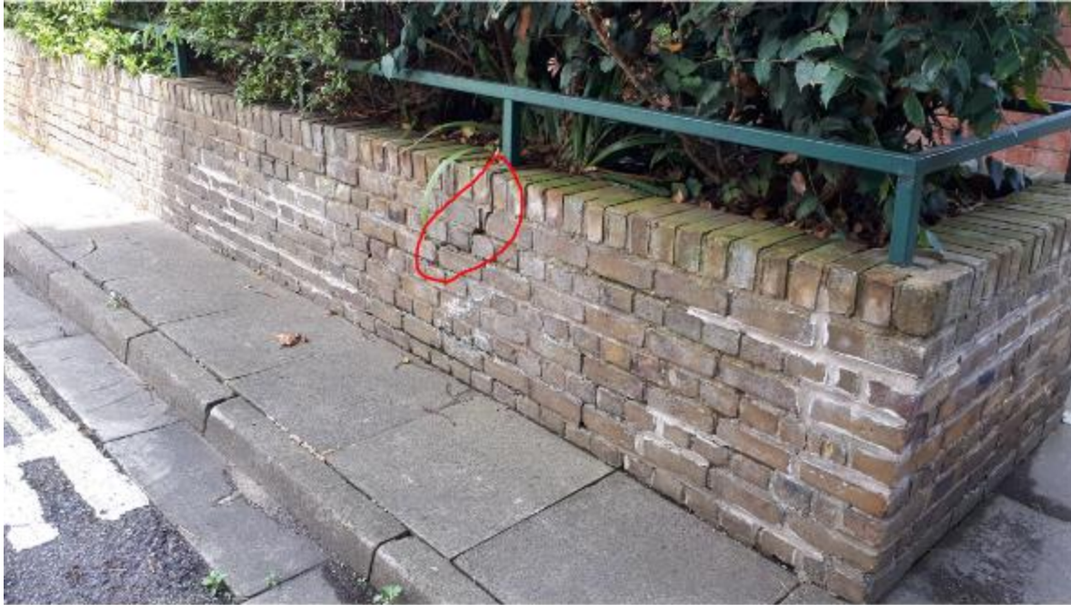
Photo 125. Again, showing retaining walls to raised beds and evidence of previous repointing although there is more still to do. Repointing as and when required is probably the most inexpensive and practical way of tackling the ongoing problem of movement cracking as trees and shrubs continue to grow; that and seasonal cutting back of vegetation and lopping of trees. The use of HeliBars could simply shift the cracking to elsewhere along the walls.
