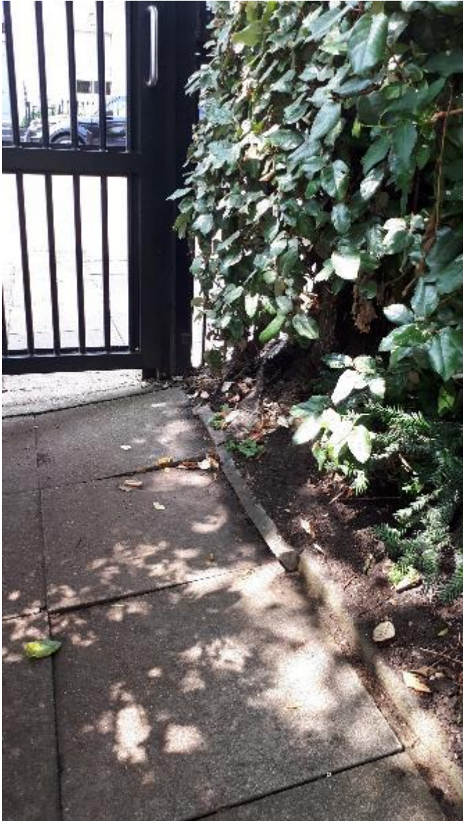
Photo 141. Paving slab and edging displacement.
