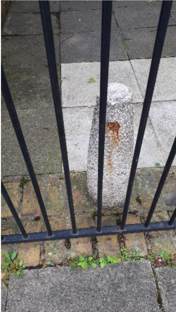
Photo 151. Early signs of rebar corrosion to bollard.
