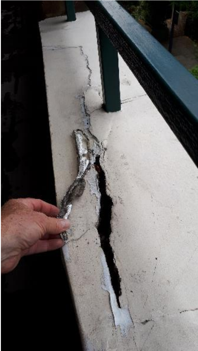
Photo 113. As on other Blocks the walkway copings are defective, here the cracking has been filled with mastic.
