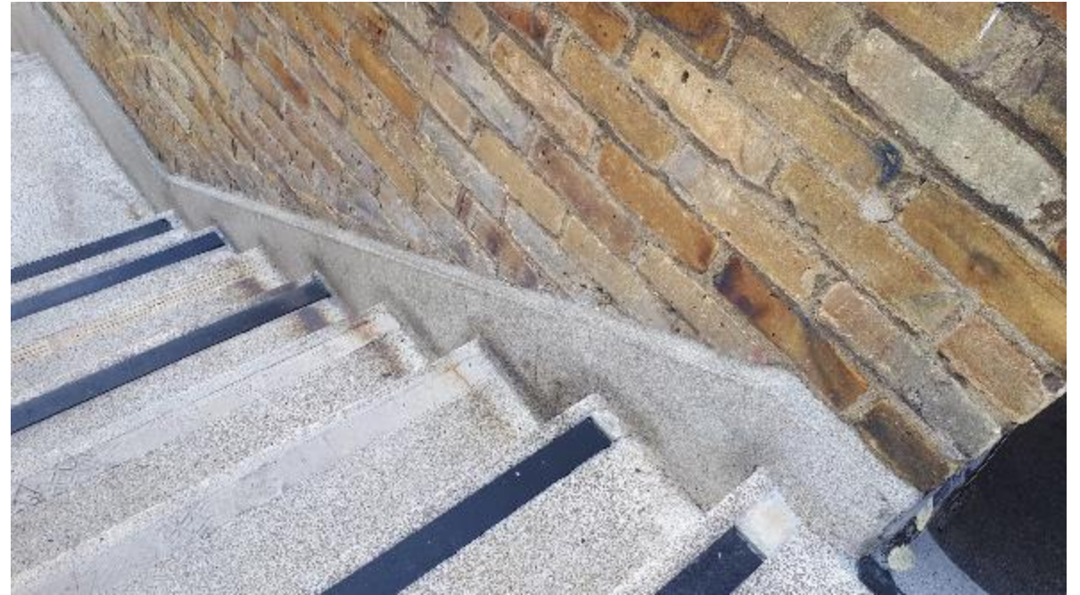
Photo 80. Same stairs, showing cracking to re-rendered wall stringer plus, missing and shrunken nosing strips.
