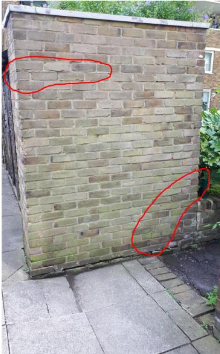
Photo 117. Same pram shed showing need for localised repointing of brickwork, any hairline stepped cracking considered to be of minor significance.
