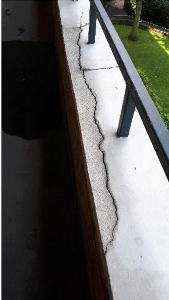
Photo 69. As on other Blocks, the coping is once weathered, shredding rainwater onto the walkway deck. Here the coping drip groove is choked with historic repair mortar (see next photo). The surveyor is of the opinion that the as-built 12inch (305mm) wide coping is not wide enough to effectively shed water away from the face of the brickwork. The inside edge of the drip groove should be a minimum of 20mm away from the brickwork face which was not always found to be the case as the thickness of the walls varied.
