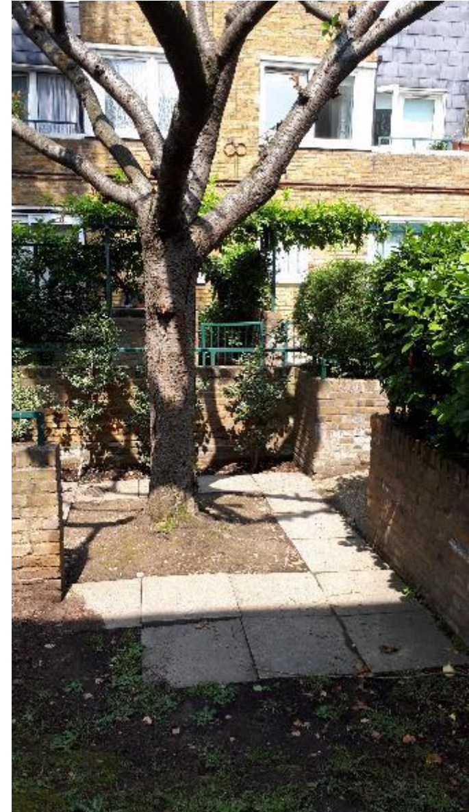
Photo 134. Paving slab heave caused by roots despite tree being lopped, in this case it would be better to replace the paving for grass.
