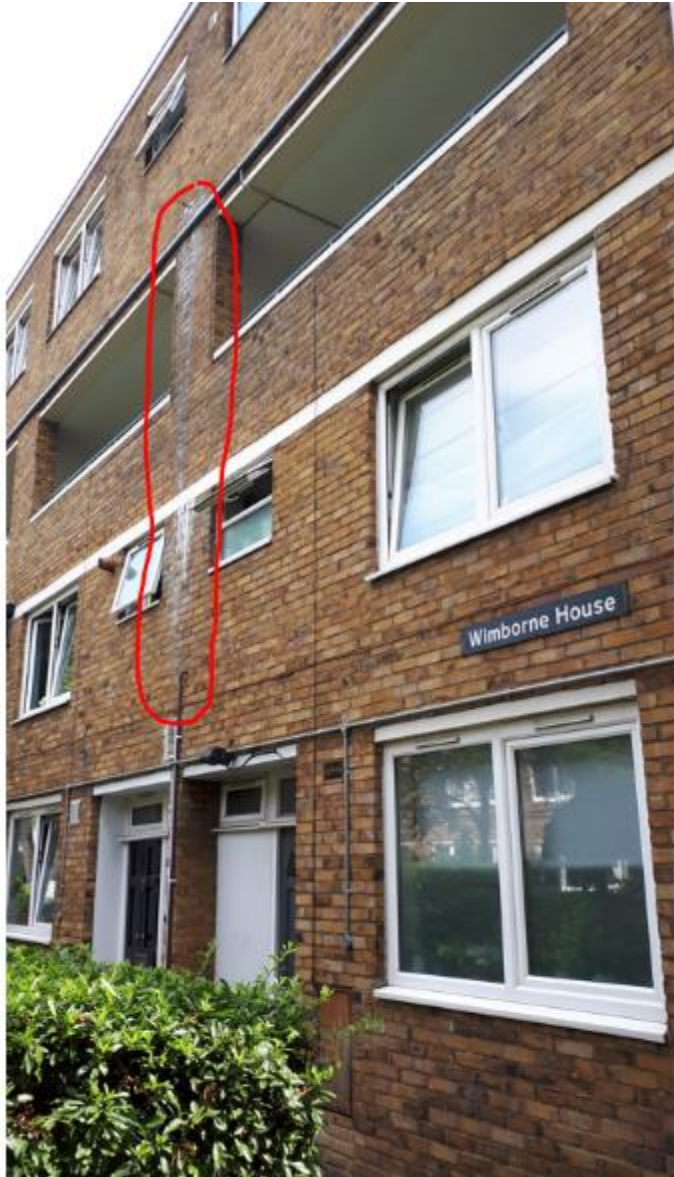
Photo 107. Significant limescale build-up to façade of four storey Wimborne Hse Block.
