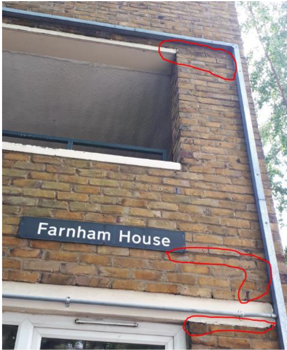
Photo 85. Similar cracking as seen on the other Blocks.
