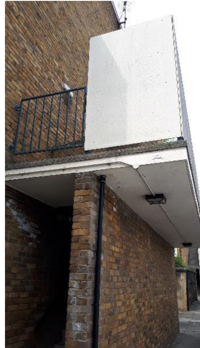
Photo 108. As on other Blocks, failing decorations to stairs nearest railway.
