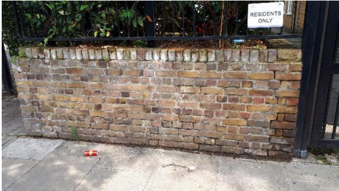
Photo 161. Same wall with defective brickwork.
