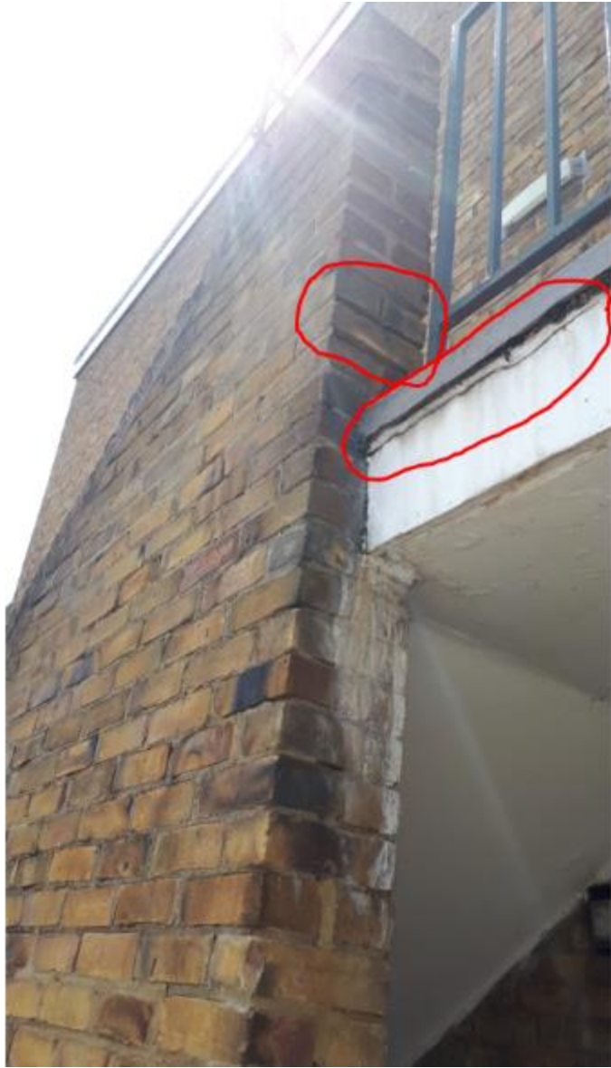
Photo 79. Same stairs, defective pointing and cracking are probable points of water ingress, seeping out below the soffit indicated by heavy limescale build-up.
