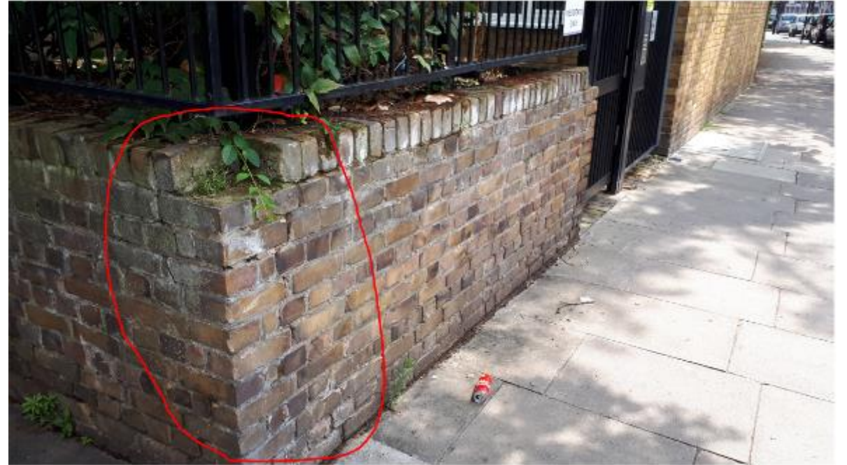
Photo 160. Again, showing movement cracking to ends of a boundary wall. Given the wall is adjacent a public footpath, the Council should consider using HeliBars to stitch the brick work as a belt and braces approach to rectifying the defect; normally one would simply repoint it.
