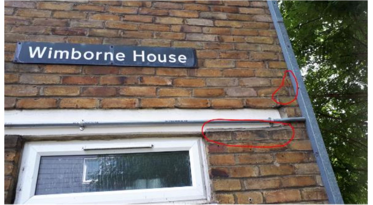
Photo 102. Wimborne House, same location as on other Blocks (front elevation, RHS end adjacent Harewood Avenue) showing evidence of minor movement cracking considered not to be an immediate cause for concern despite close proximity of mature acacia trees, see next couple of photos.
