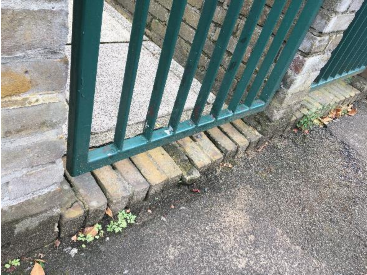
Photo 49. In some cases, the brick steps to rear garden gates are defective.
