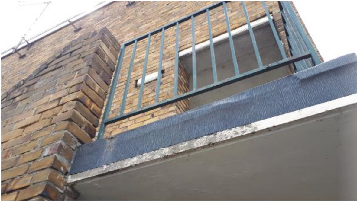
Photo 95. Farnham Hse stairs adjacent railway, note defective pointing to brickwork and historic covering repair carried out to mitigate moisture penetration.
