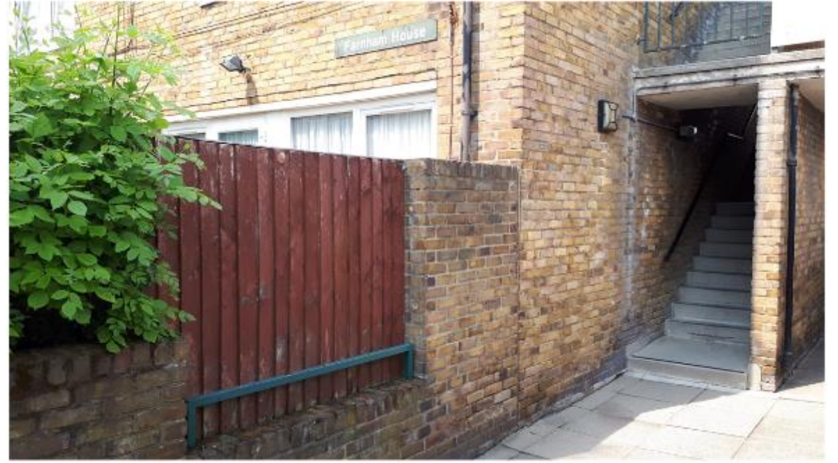
Photo 94. Generic limescale build-up, defective brickwork pointing and failed decorations.
