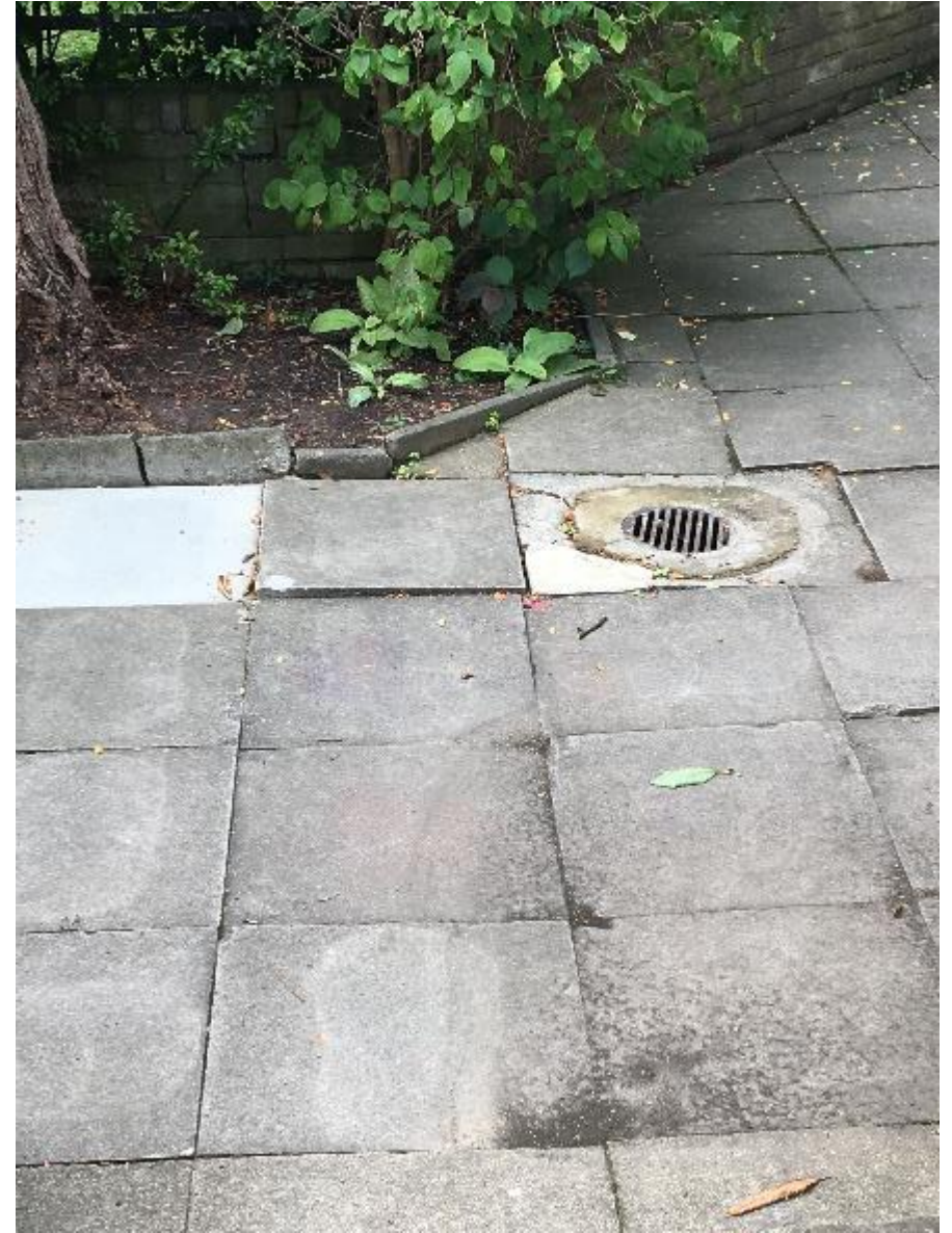
Photo 142. As previous photo but with possible drainage damage.
