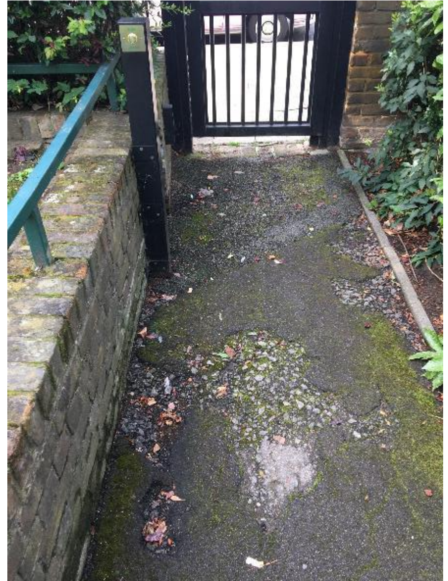
Photo 138. As previous photo.
