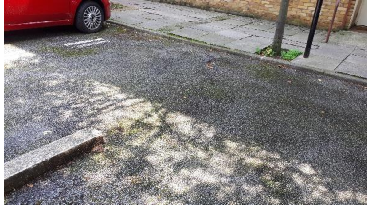
Photo 154. Same carpark where the tarmac is breaking up.
