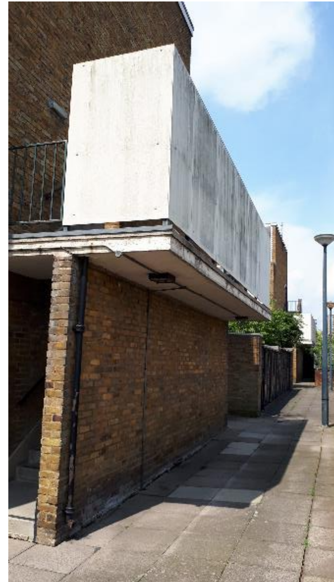
Photo 76. As on other Blocks at the railway end, the landing guarding needs redecorating.
