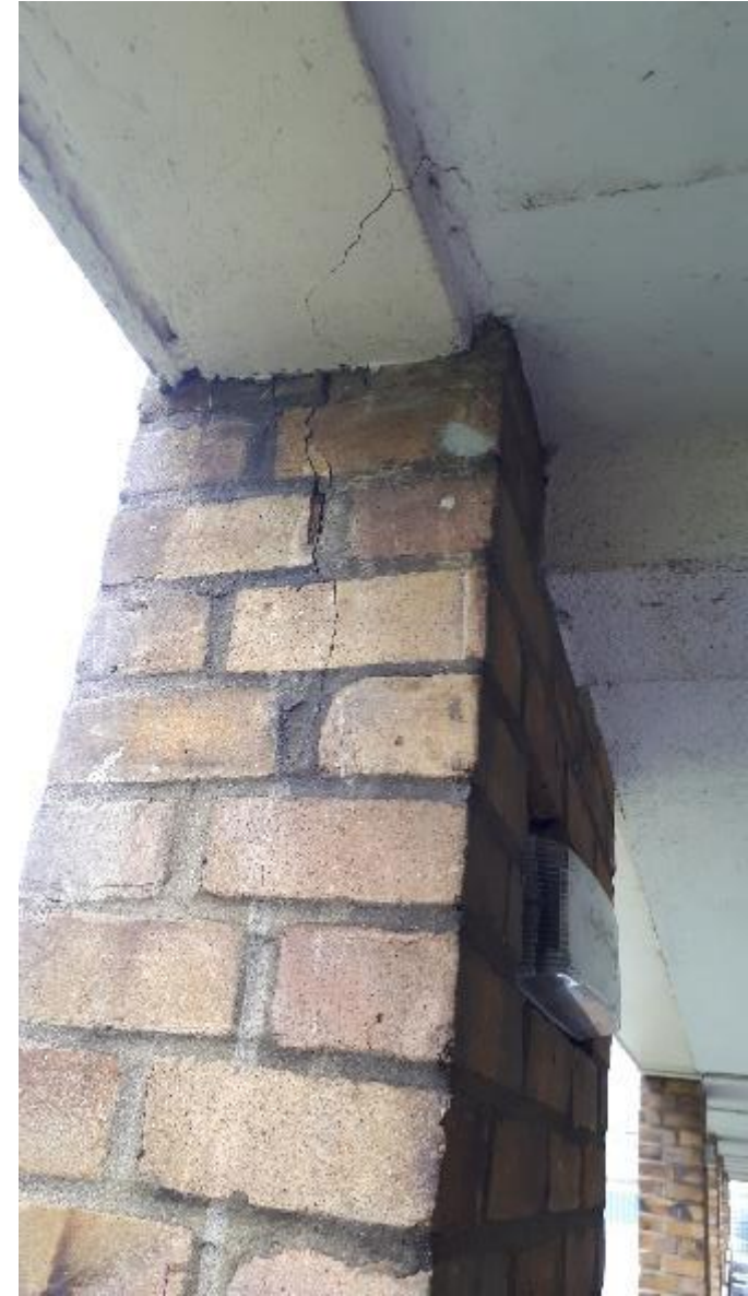
Photo 112. As on other Blocks, here on Wimborne the brickwork walkway pillar is cracked.
