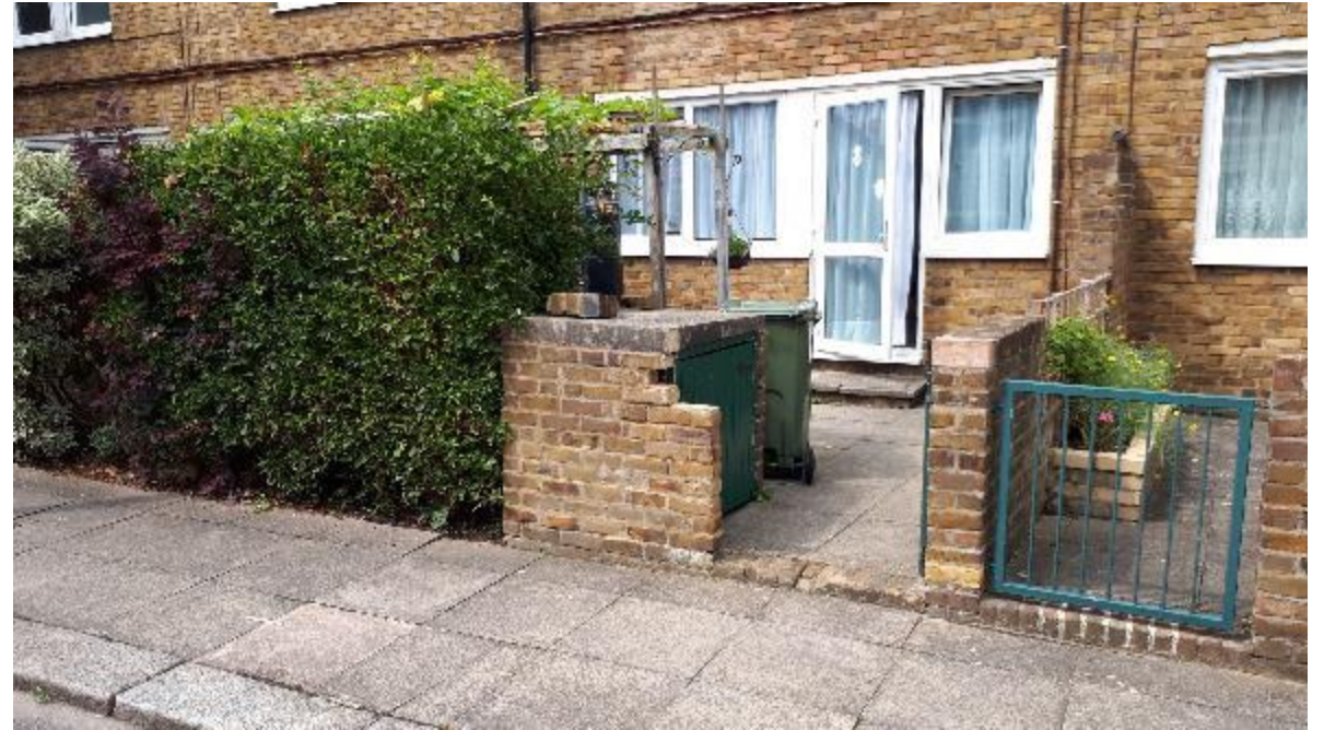
Photo 114. As elsewhere, the private garden boundary walls at Wimborne Hse are defective.
