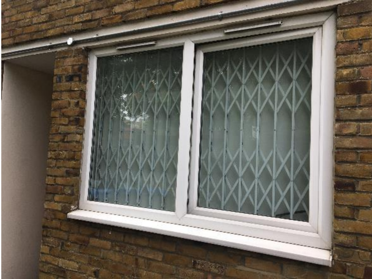
Photo 41. Back down at ground level, typical window in good condition and consideration should be given to cleaning the PVCu.
