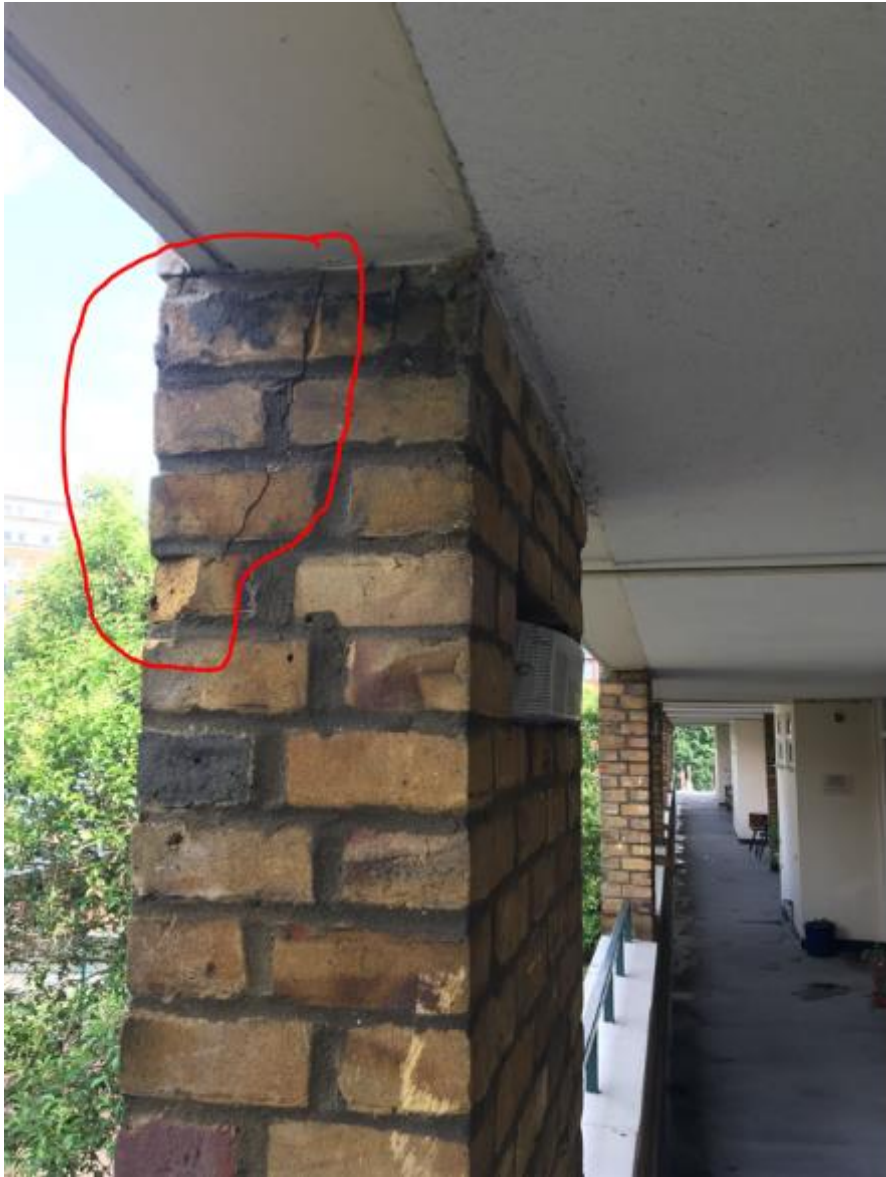
Photo 23. Cracking to brick pillar of communal walkway at Mordern Hse, possibly caused by vertical compression. Note the width of the historical repointing mortar.
