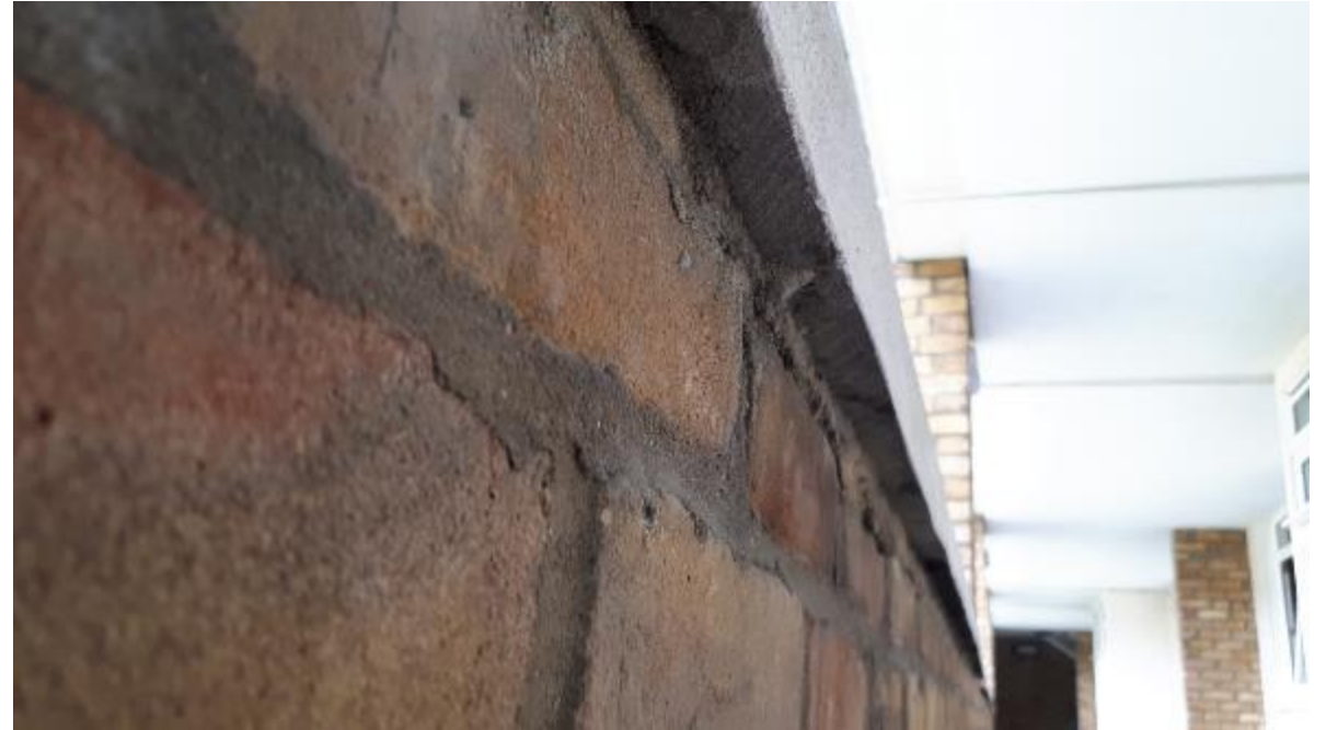
Photo 70. Showing historic repair mortar choking drip groove.
