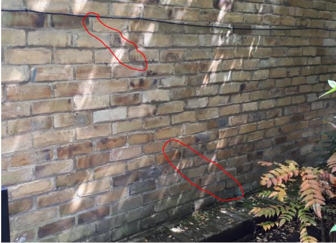
Photo 103. Close-up of stepped movement cracking to flank elevation considered to be of minor significance given width of cracks and fact that the bricks are not fractured.
