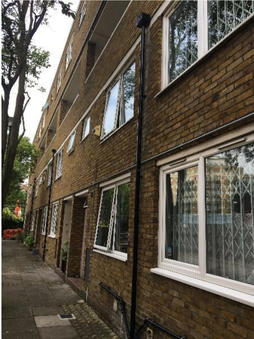
Photo 5. Again, showing front elevation rainwater goods serving communal walkways which are considered to be in good condition as they appear to be relatively new.
