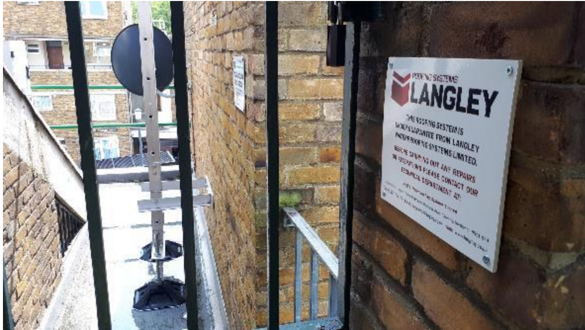
Photo 63. Same roof section and evidence of replacement/overlay covering.
