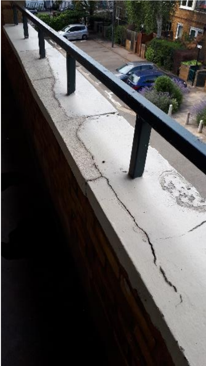
Photo 99. Generic walkway coping failure.
