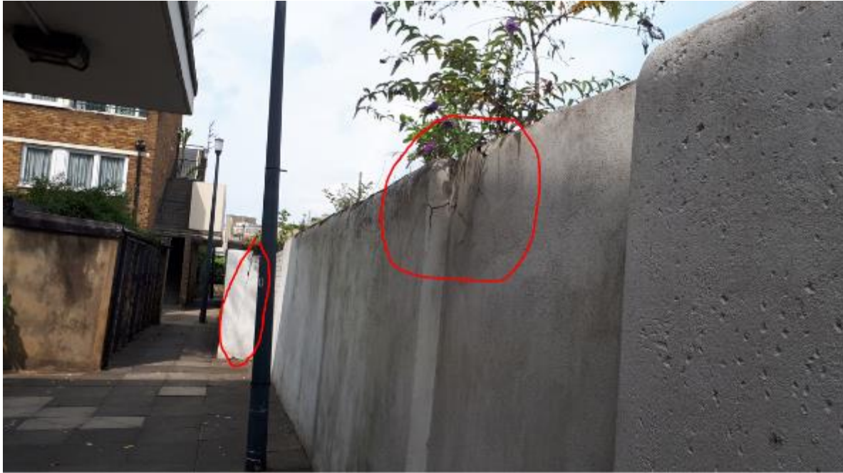
Photo 169. Showing failed render finishes to same boundary wall.
