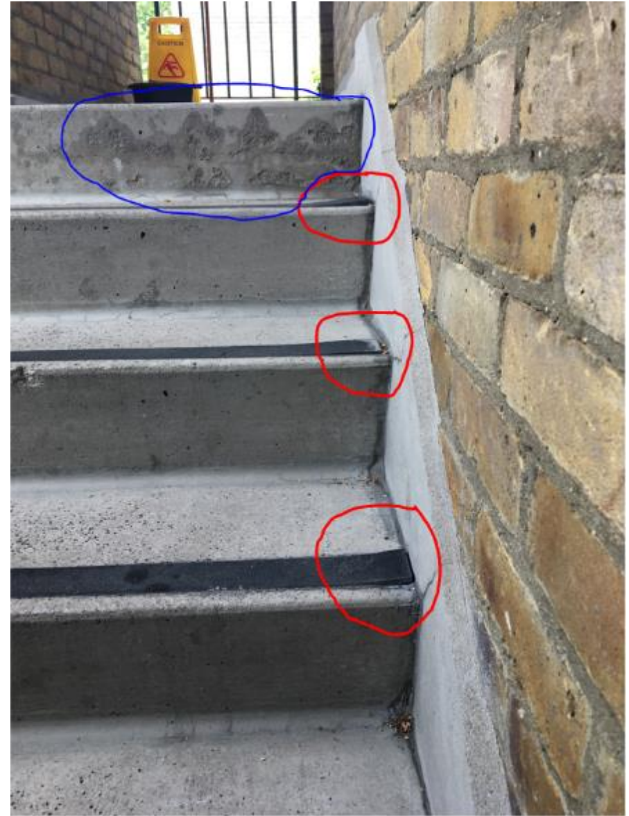
Photo 34. Rubberised strips lifting (red) also note the residual damp (blue) left after stairs have been washed down.
