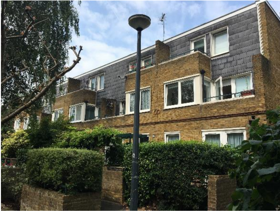
Photo 3. Rear elevation fascia boards.
