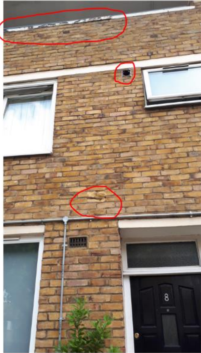
Photo 87. Again, generic defective coping and pointing plus, missing extract fan duct grille and impact damage to brickwork.
