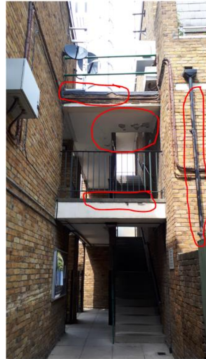
Photo 98. Rear view of Farnham Hse stairwell showing generic defects as found on the other Blocks i.e., failing decorations and mastic asphalt.
