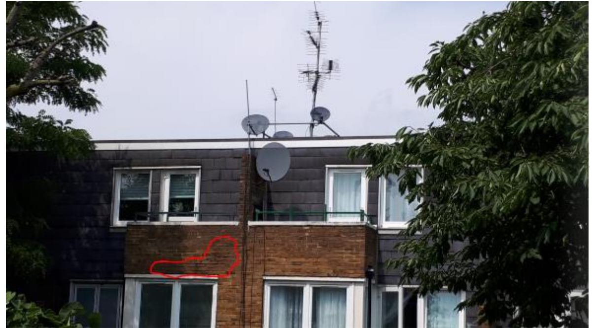
Photo 56. Again as on other Blocks, there is defective brickwork pointing at height.
