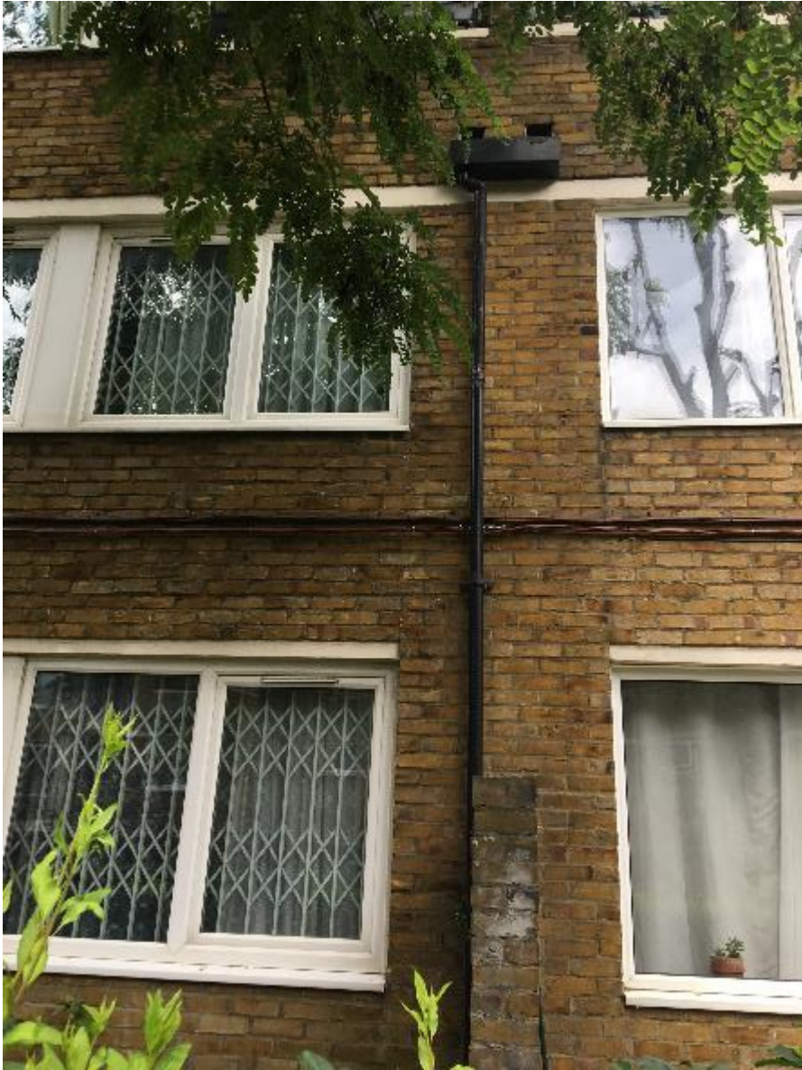
Photo 9. Across the Blocks, the painted and assumed cast-iron or galvanised steel rainwater goods serving the 2 nd flr private balconies to the four storey Blocks are in fair condition but will require rust treatment and redecoration.
