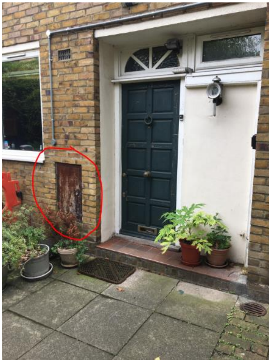
Photo 43. Generally, decorations to ground floor entrances looking tired particularly meter cupboard doors.
