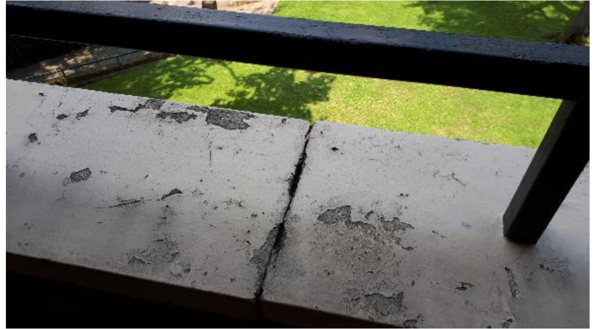
Photo 72. Defective coping joints let rainwater in and corrode rebars, exacerbating the defect.
