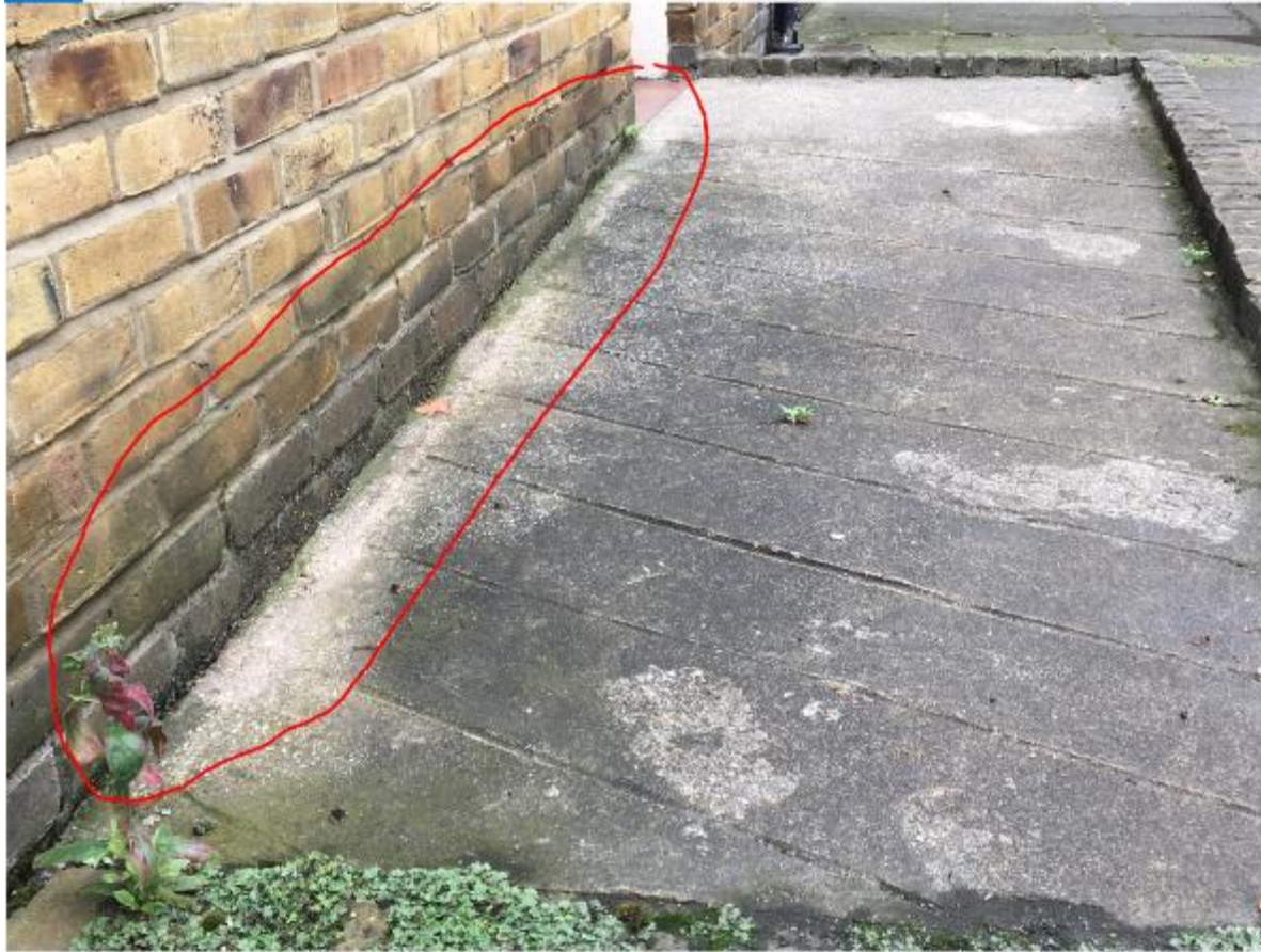
Photo 45. Ramp against wall is bridging the DPC however, it is a cavity wall and unless the cavity is breached by builder's debris or mortar snots, it is not a problem with regard to penetrating damp.
