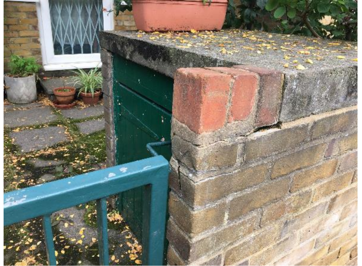
Photo 50. In many cases the rear garden boundary wall brickwork is suffering from impact damage.
