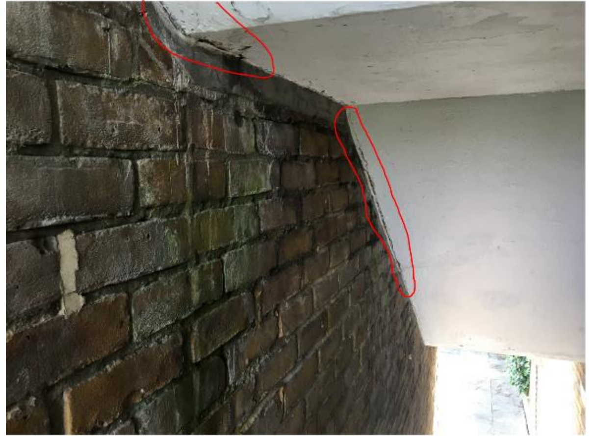
Photo 20. Evidence of water penetration between soffit and wall of same steps, either the outer face of the brickwork needs repointing and/or the riser and tread skirting above has failed.
