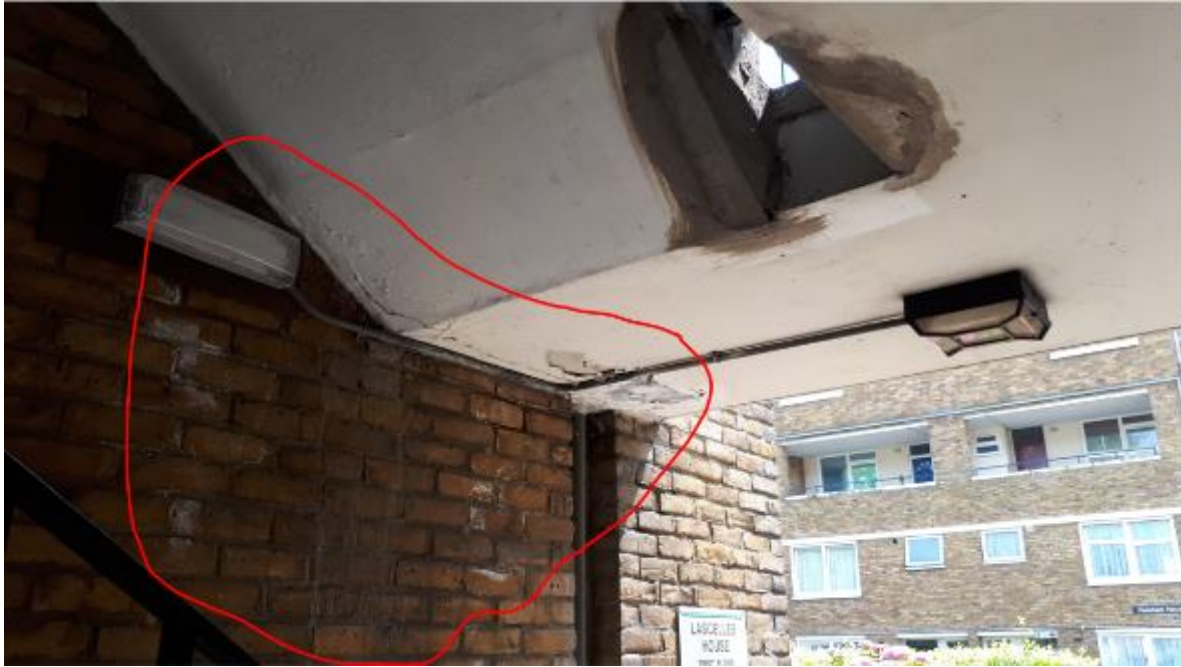
Photo 65. As shown in photo 61, water damage to decorations of stairwell soffit, note past repair to core.
