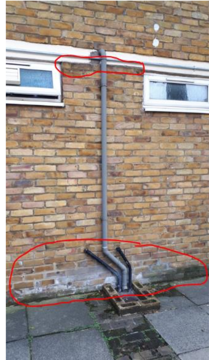
Photo 88. Arguably looks worse than what it is unless wall cavity and DPC have been breached. Repointing required between windows, a defect found on other Blocks.
