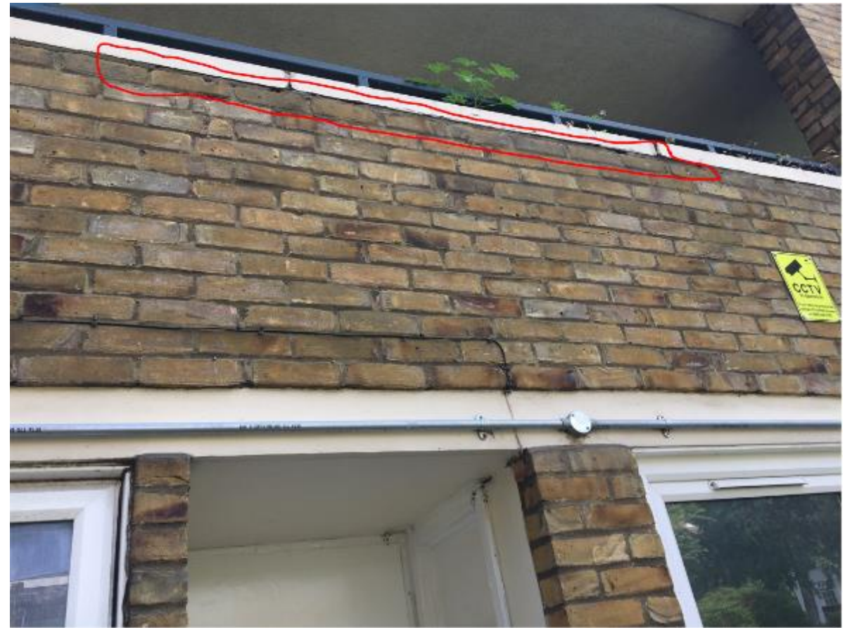
Photo 52. Here, as is generally the case across the Blocks, the communal walkway parapet copings are failing due to moisture penetration and freeze thaw action.
