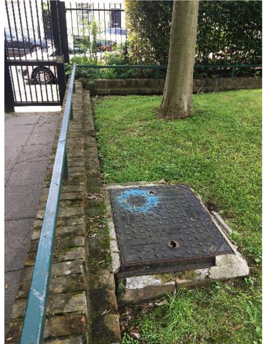
Photo 132. Inspection chamber frame needs re-flaunching.
