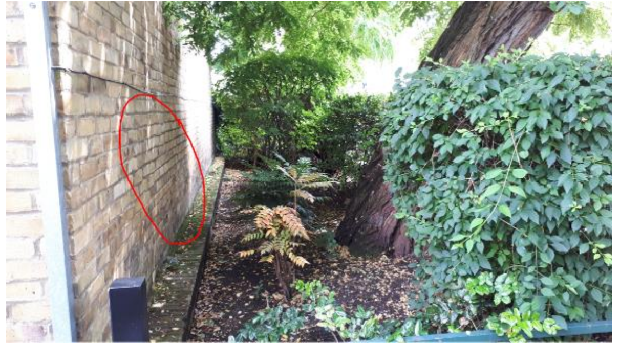
Photo 104. Showing location of same stepped cracking in relation to acacia tree.
