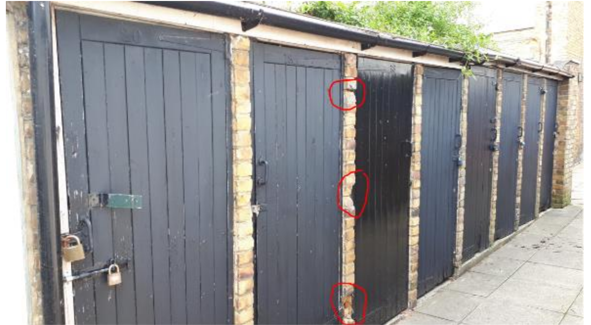
Photo 118. Pram shed brickwork and joinery repairs required as well as redecoration.
