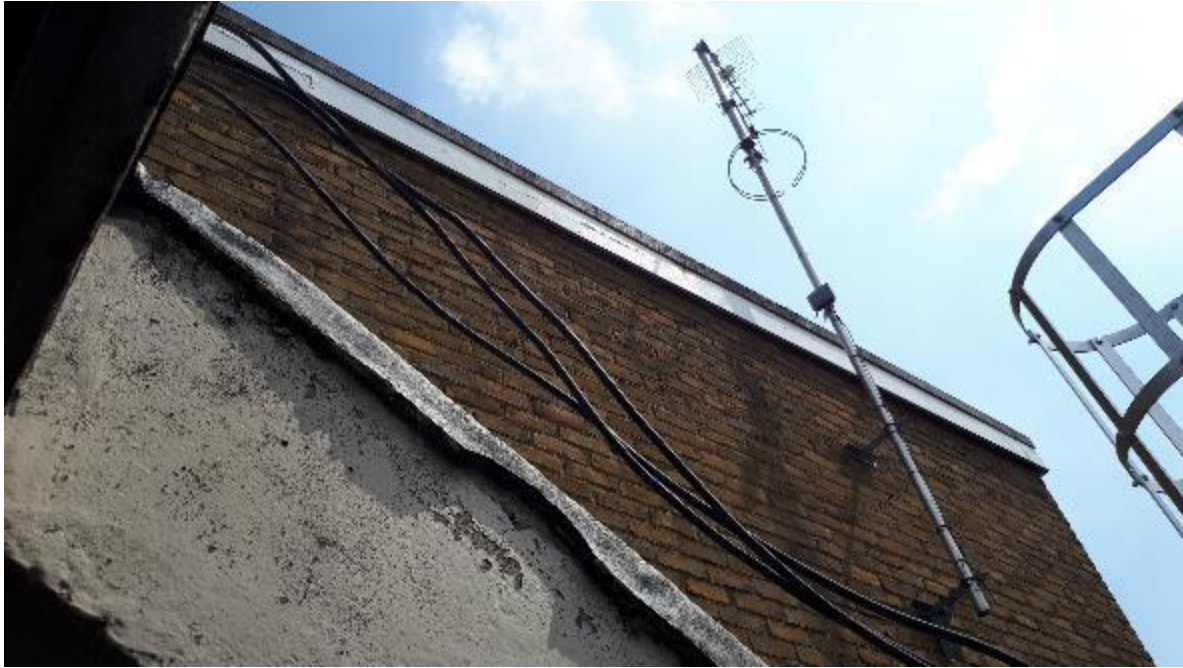
Photo 59. Again showing failed paintwork at height.
