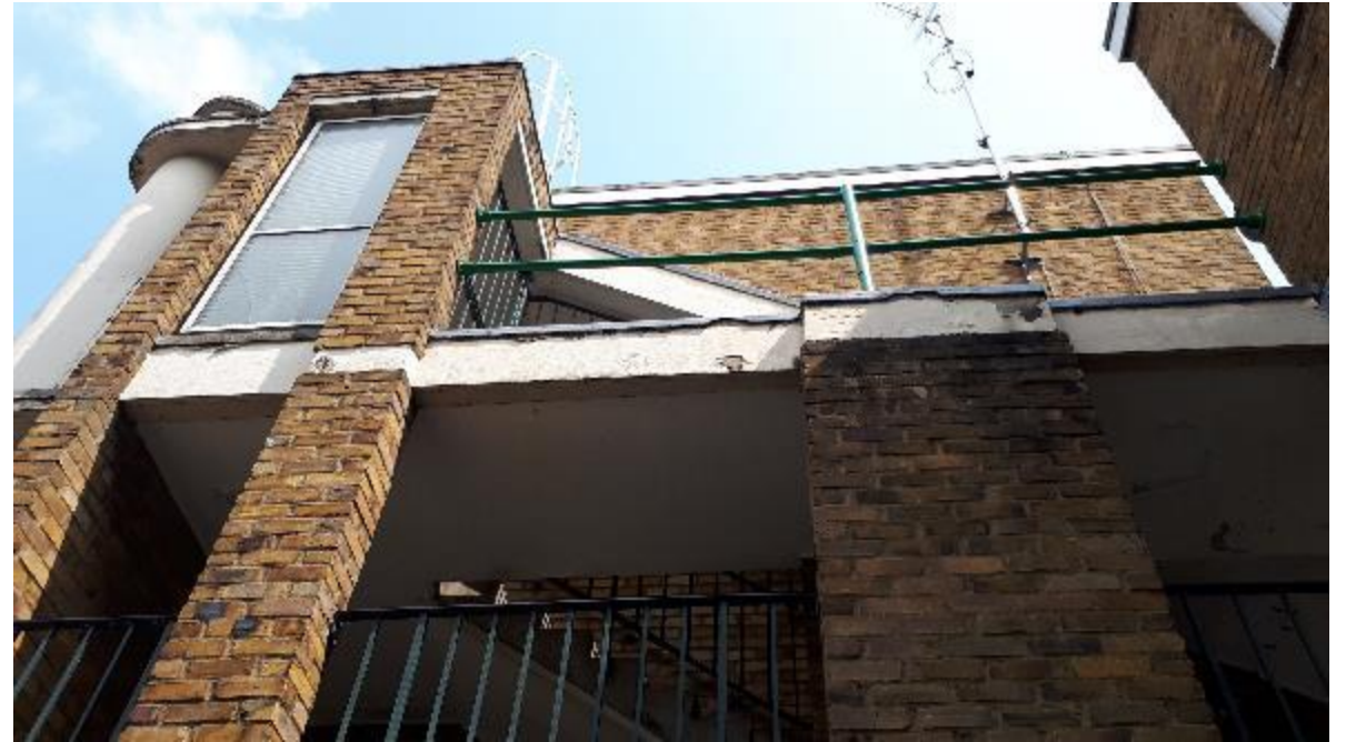
Photo 90. Failing decorations and defective mastic asphalt coverings.
