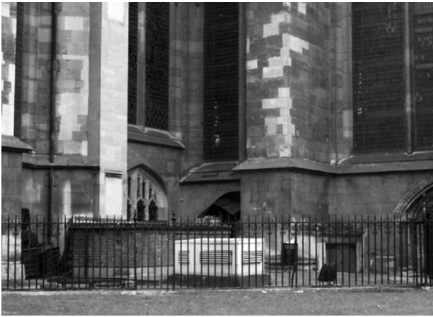
Figure 144: Air-conditioning unit to the front of Westminster Abbey
