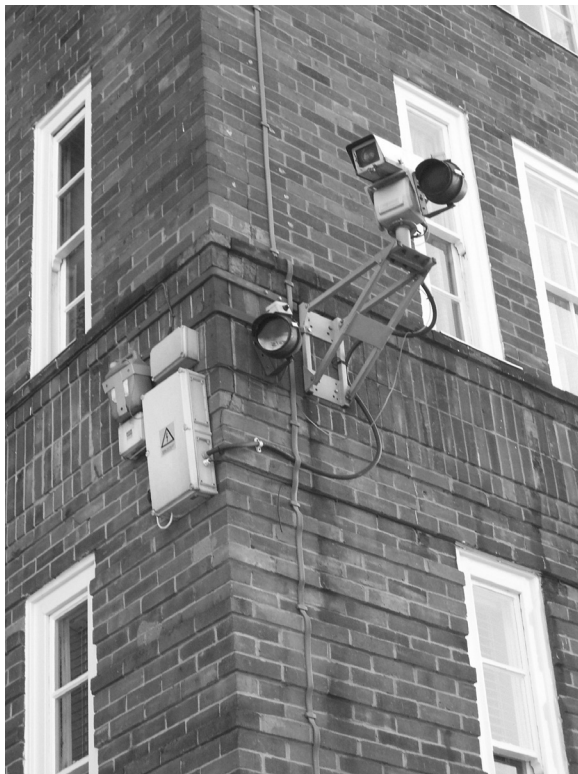
Figure 60: unsympathetically placed CCTV camera equipment
