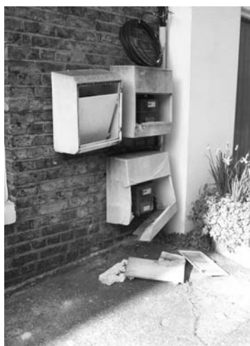
Figure 147: Poorly maintained service boxes, Linhope Street
