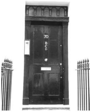
Figure 37: 4-panel door with attractive rectangular fanlight, repeated across buildings on northwest section of Balcombe Street
