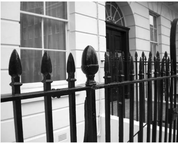
Figure 99 & 100: There are a wide range of different finials to railings in the conservation area, including spearhead, fleur-de-lys and Arrowhead finials
