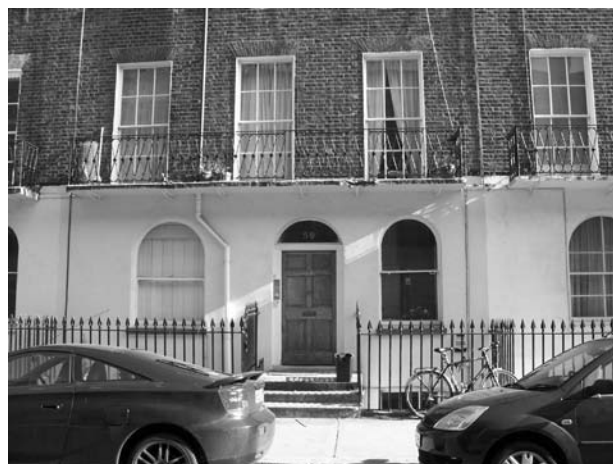
Figure 140: Example of windows which have lost their original glazing bar pattern to the ground floor (No 59 Balcombe Street).
