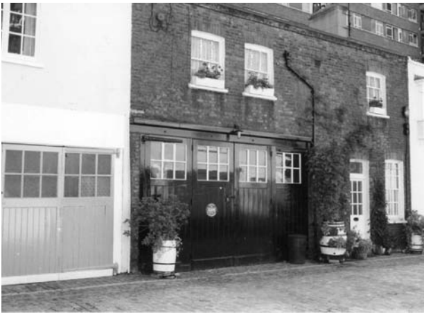
Figure 56: Traditional timber carriage doors such as those above have been lost in many of the mews building in Dorset Square.
