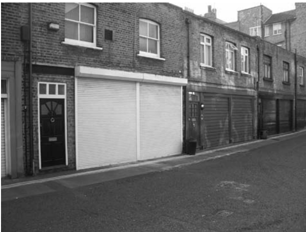
Figure 142 and 143: Examples of modern garage doors which have a detrimental effect on mews character
