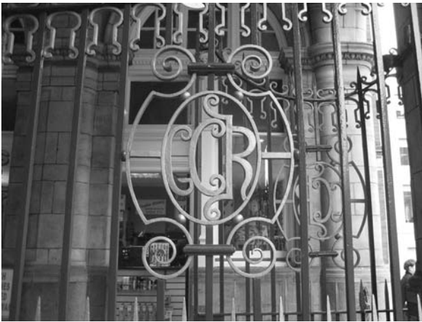
Figure 111-113: (top) Elaborate detailing to gates of Francis Holland School; (middle) Boundary Wall to Francis Holland School; (below) Detailing to gates of Marylebone Station
