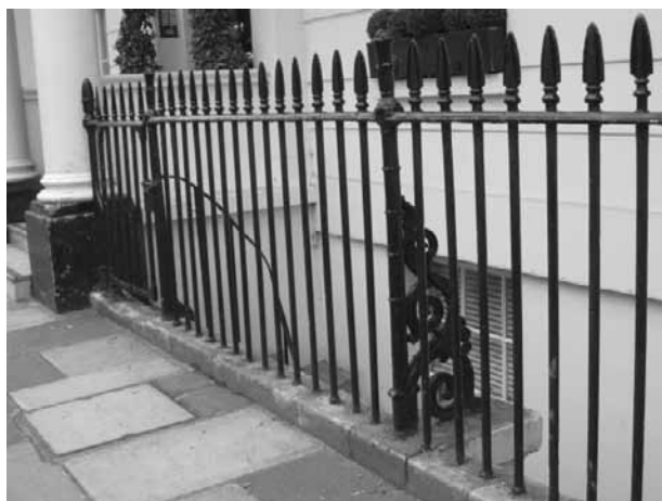
Figure 143: The most common design of railings fronting Belgravia terraces, with spearhead finials and more elaborate standards with support panels.
