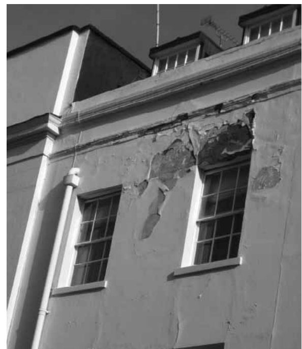
Figure 226: Peeling paintwork Chester Row.
