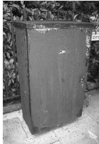
Figure 243: (left), service box painted with anti-graffiti paint Figure 244 (below), Ebury Street.
