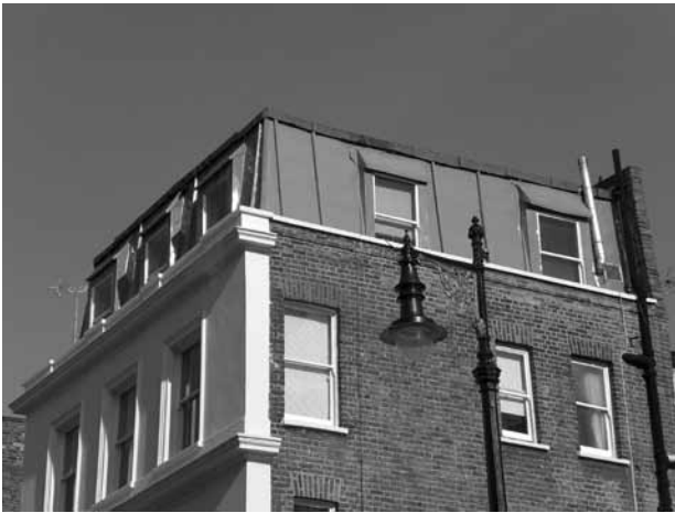
Figure 230: (above) Poorly detailed mansard, 81 Chester Square.
