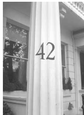
Figure 116: ( left ) Black painted house number on Doric column of projecting porch, 42 Eaton Square
