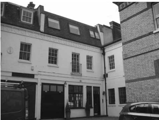
Figure 232: Some roof extensions have been poorly executed with steeply pitched roof slopes and non-traditional window detail (No.23 Grosvenor Crescent Mews).
