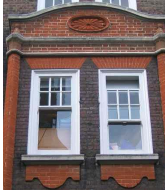
Figure 25: Mansion block window detail showing double sliding sashes with multi-pane top sash and plain lower sash and bright red brick dressings
