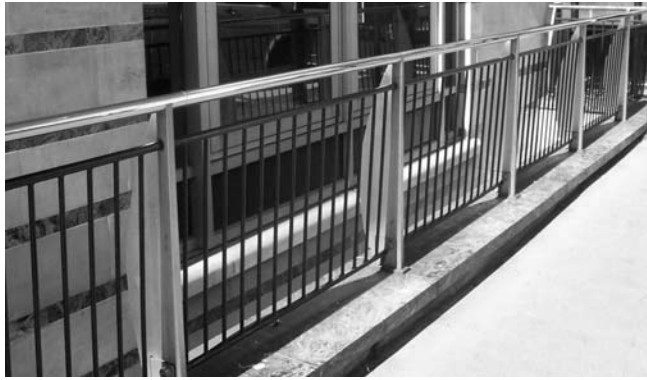
Figure 83: No. 120 New Cavendish Street Example of railings enclosing a modern commercial premises
