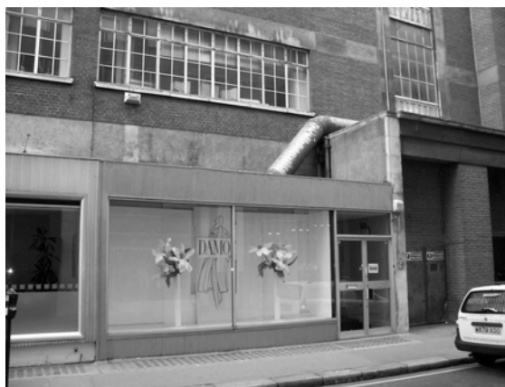
Figure 111 : 10 Winsley Street, No attempt has been made to disguise this large metal flue, which is unduly prominent on this elevation
