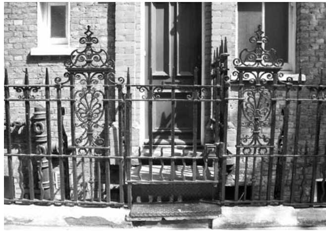
Figure 76: Elaborate wrought iron area railings enclosing a mansion block along Hanson Street
