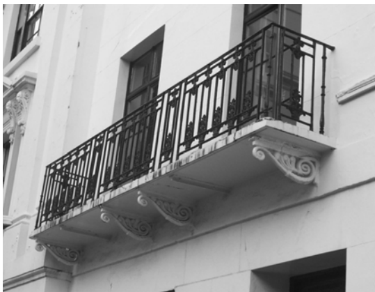
Figure 26: Balconies at first floor level are principally of cast iron panels supported on decorative cast iron brackets. These balconies run the length of the south side of the square, and survive on most of the north side.
