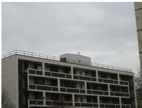
Figure: 39: Simple flat roof of 6-storey block with prominent projecting water tank.
