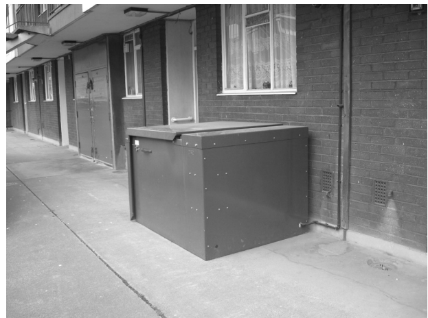
Figure 65: Large metal box for services, not integrated within the building
