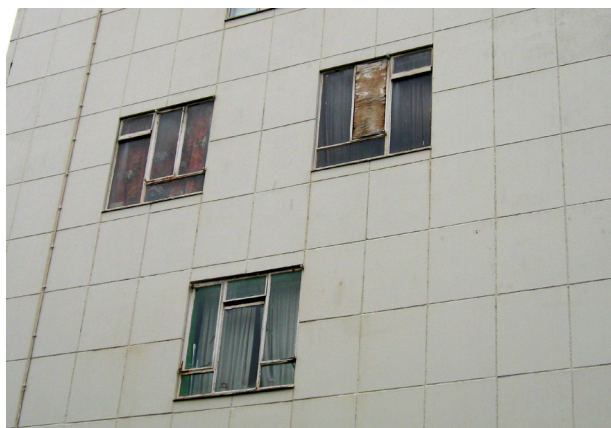
Figure 62: Windows in need of maintenance, Pembroke House
