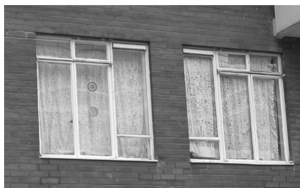
Figure 58 & 59: ( top ) replacement uPVC windows and ( below ) original windows
