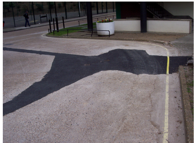
The black asphalt repair to this concrete slab roadway are another example of an unfortunate choice of materials.
