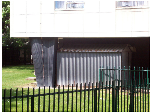
Figure 64: Pembroke House, the open area to ground floor level has been infilled with a corrugated metal structure
