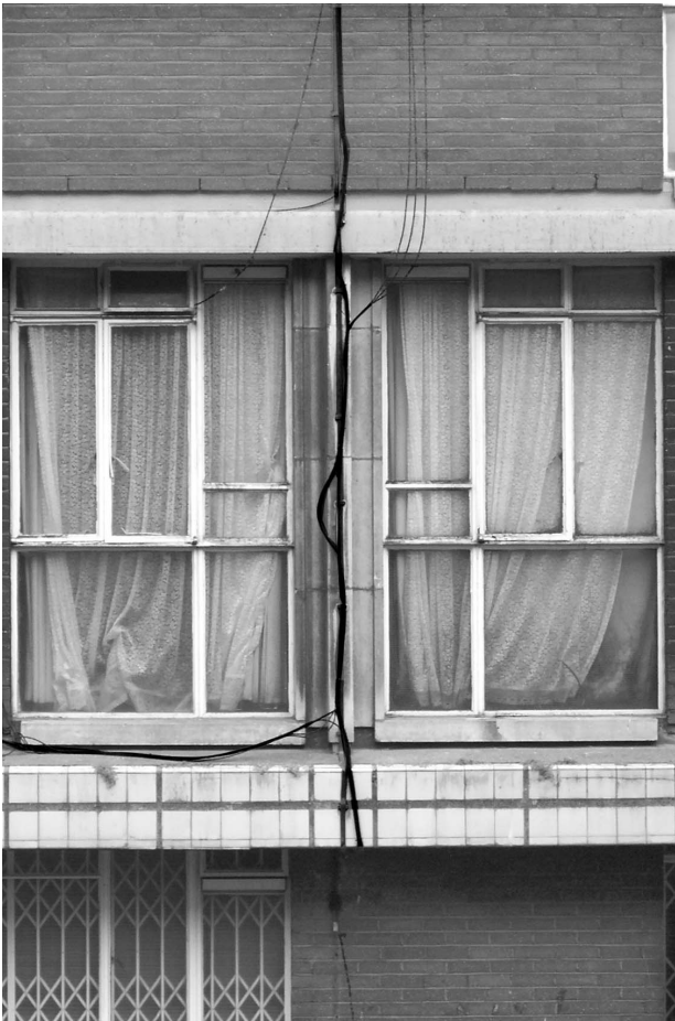
Figure 63: Wires draped across building elevation
