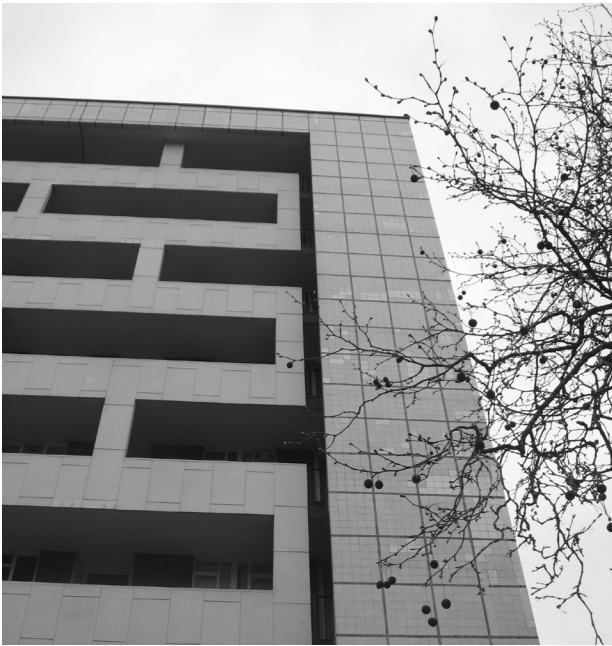
Figure 19: The shadow gap around the access balconies means that they appear to ‘float’ while the black railings are imperceptible from the ground.
