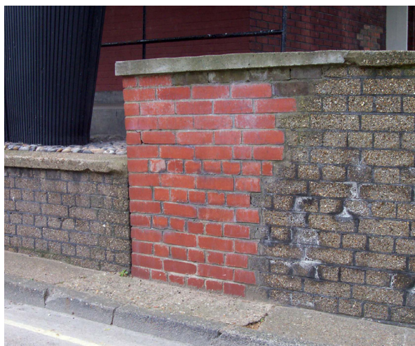
Figure 61: Replacement brickwork which does not match the original
