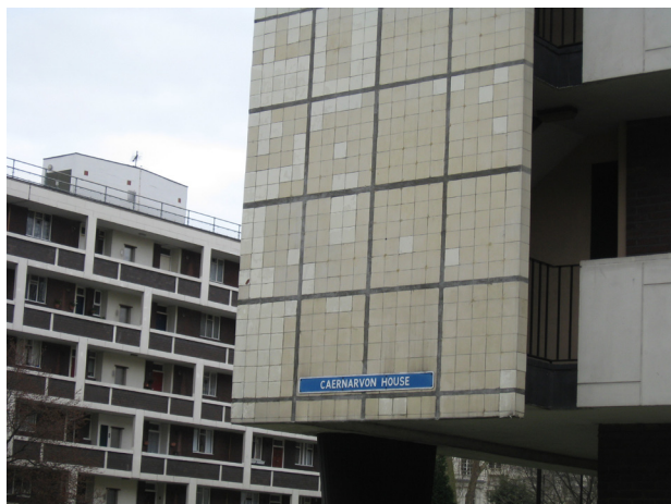
Figure 60: Piecemeal replacement of tiles, Caernarvon House
