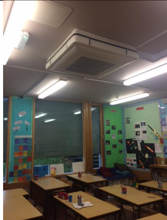
Years 4, 5 and 6 classrooms: interior remote controller and cassette (six units)
