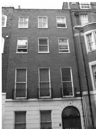
Figure 132: Harley Street. The loss of original glazing bars pattern and fanlight detail has changed the character of many Georgian townhouses
