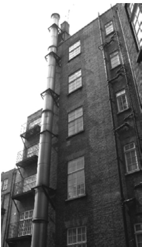
Figure 137: Large metal flue in Hallam Mews
