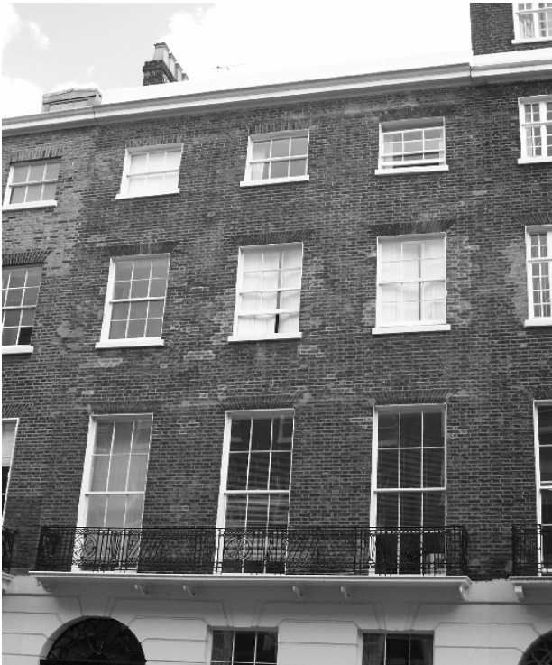
Figure 15: Typical hierarchy of sash windows to Georgian townhouse on Upper Harley Street, with 6-over-6 sashes to first and second floors and 3-over-3 sashes above
