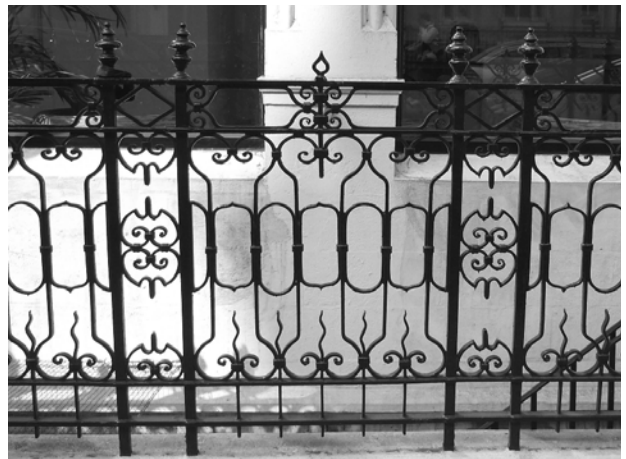
Figure 100: Early 20th century railings with cast iron standards and delicate wrought iron panels
