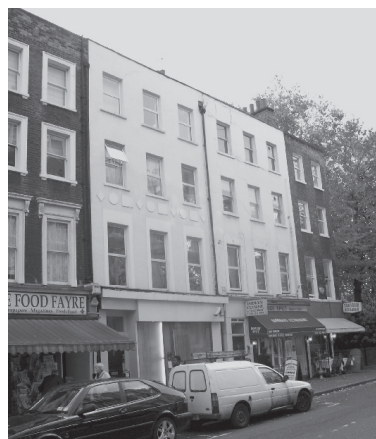
Figure 133: 50-51 Paddington Street have had the original brickwork rendered and uPVC windows added at first floor level
