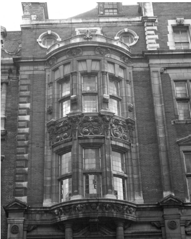
Figure 141: The stone dressings to Nos. 55-91 Knightsbridge would benefit from cleaning special character and architectural interest. Parkside, on the north side of Knightsbridge, has recently been cleaned, resulting in a great improvement in the appearance of the building. On the south side, no. 55-91 Knightsbridge is currently badly stained, and would benefit from a similar treatment.
