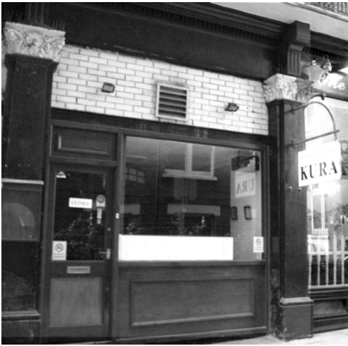
Figure 137: Within this traditional shopfront surround a poor quality modern shopfront has been inserted.
