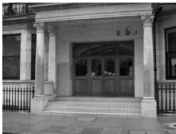
Figure 129: Alterations to door and portico in Ennismore Gardens. The middle column of the portico has been removed and new doors inserted
