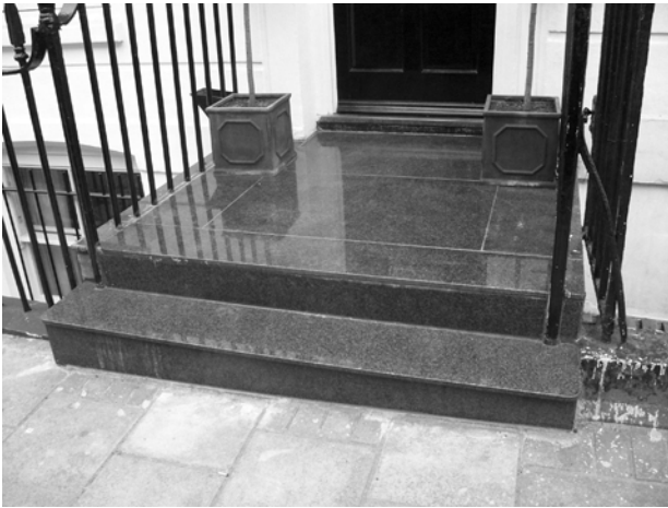
Figure 130: Shiny marble replacement front steps stand out in the streetscape
