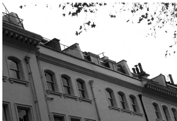
Figure 128: Missing dentil cornice detail, Ennismore Gardens
