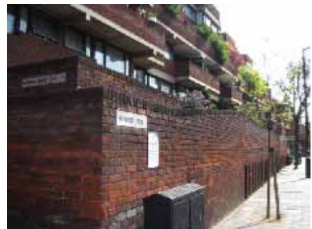
Figure 97-100: Top and centre red brick walls and timber stained gates to gardens. Bottom , walls fronting Tachbrook Street
