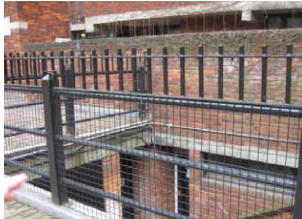
Figure 164: the simple railing detail has been modified in places for security purposes. A simpler treatment may be more appropriate.
