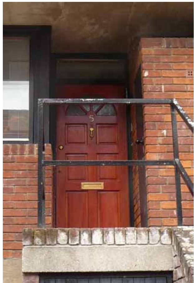
Figure 152: Inappropriate replacement door, Goodyer House
