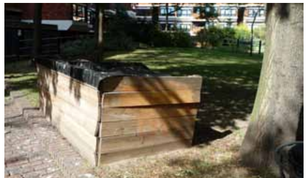
Figure 133: Composting boxes have been provided within the gardens, which provide an important amenity, although some are not in good repair
