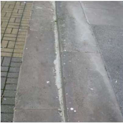
Figure 70: Original stone kerb to the circumference of each of the Lutyens' courtyards
