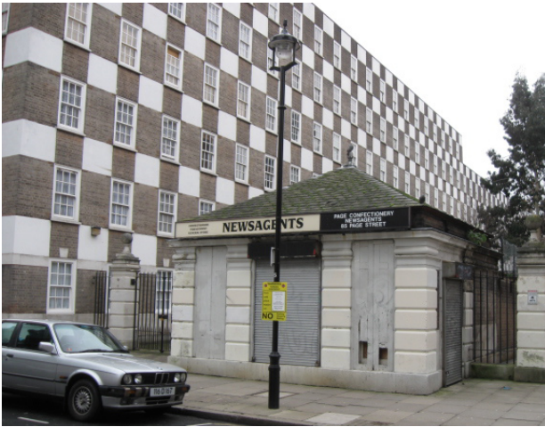
Figure 93: Vacant no. 85 Page Street with damaged wooden shutters and roller shutters which further contribute to its negative impact on the conservation area
