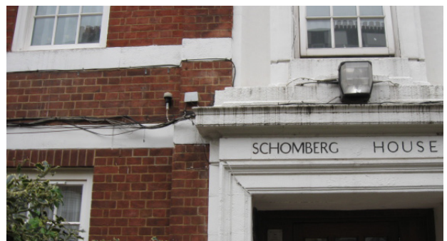
Figure 90-92: Examples of wires
