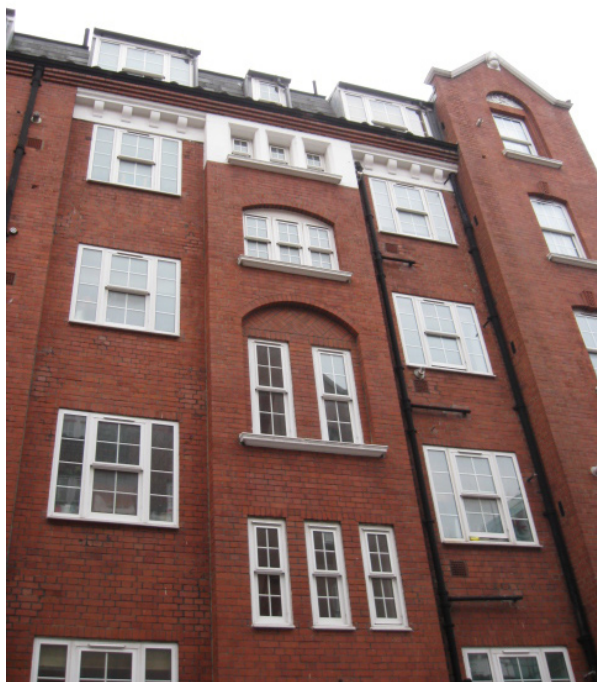
Figure 20: Fenestration pattern above each entrance ( above ) is repeated along the length of each block.
