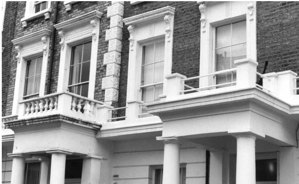
Figure 51: Inappropriate horizontal bar railings inserted in the place of traditional balustrade.
