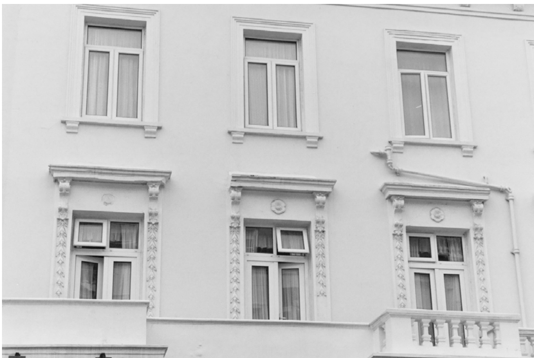
Figure 50: Replacement windows. The original windows have been replaced with uPVC casement windows, crudely designed with inappropriate glazing bar detail
