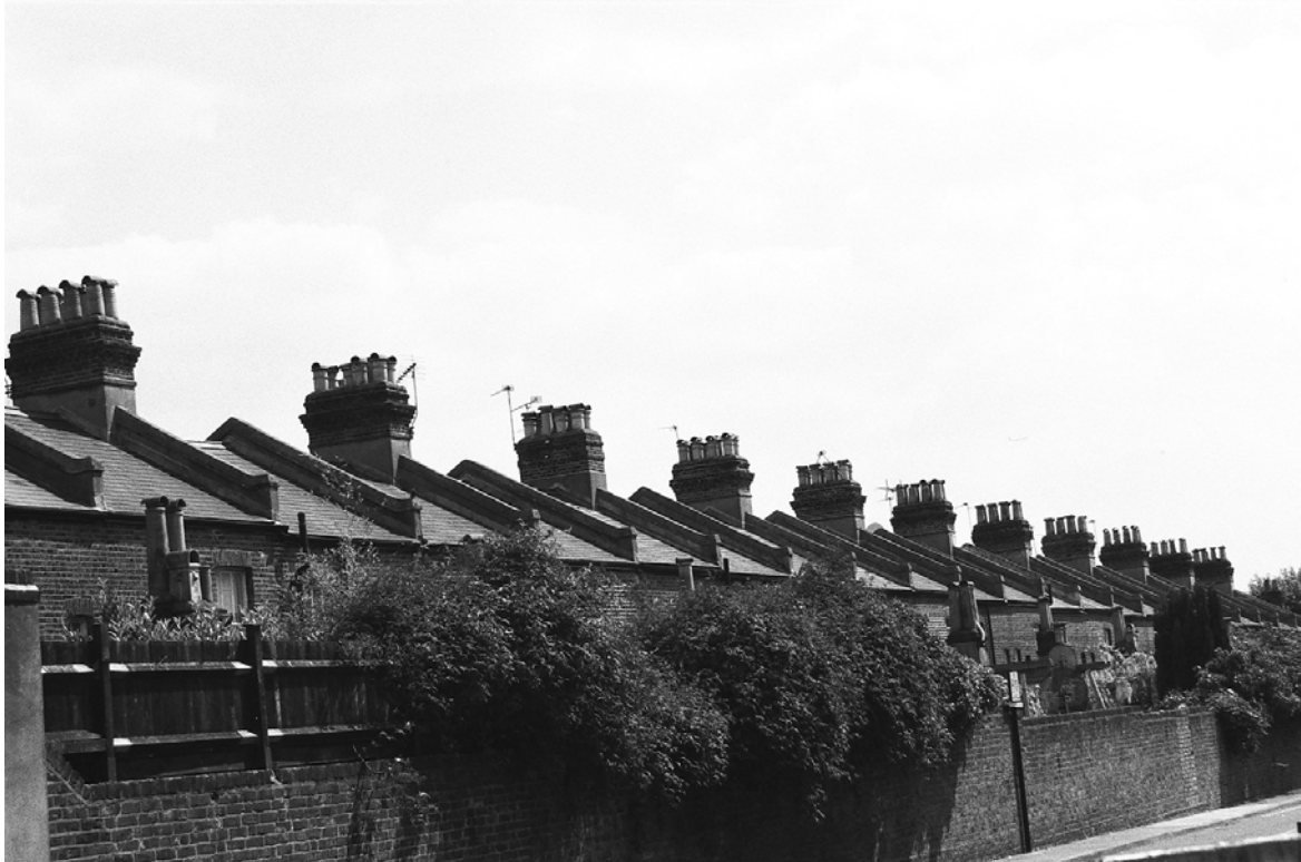
Figure 13: The regular rhythm of the roofscape, punctuated by stout chimneystacks and raised party wall upstands.
