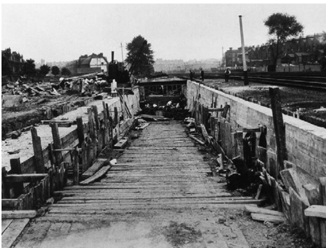
Bakerloo and Watford Junction extension, to include a station at Queen's Park, 1914
