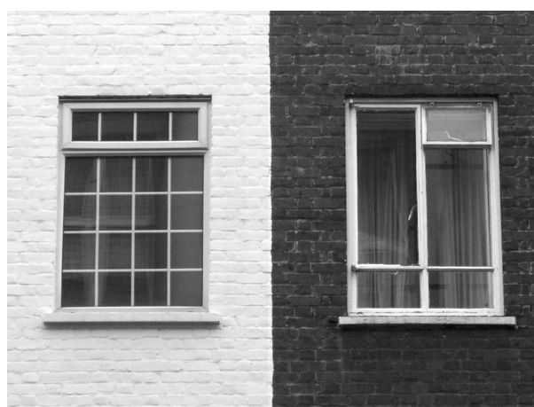
Figure 89: Replacement uPVC Window (left) and original steel framed window (right)
