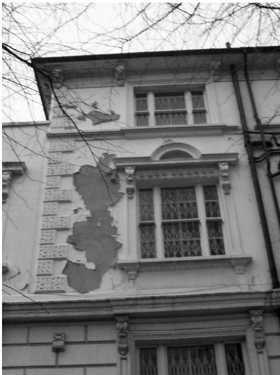
Figure 119: Poorly maintained stucco
