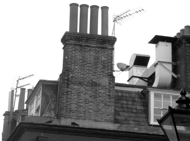
Figure 59: Roof-top plant at No. 26 James Street
