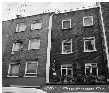
Figure 62: Poor quality replacement windows, 50 & 52 James Street
