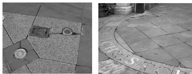
Figures 60 & 61: Damaged paving to Barrett Street/St Christopher's Place
