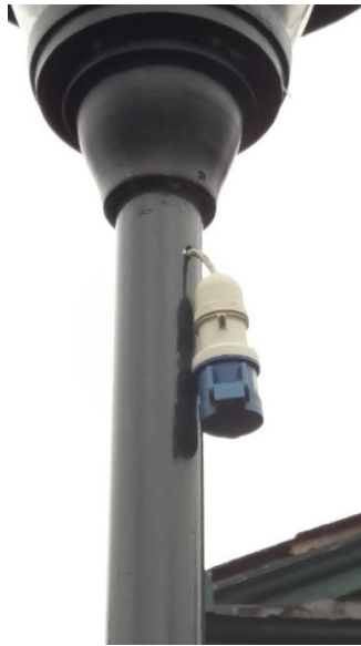
Unacceptable cable entry in column
