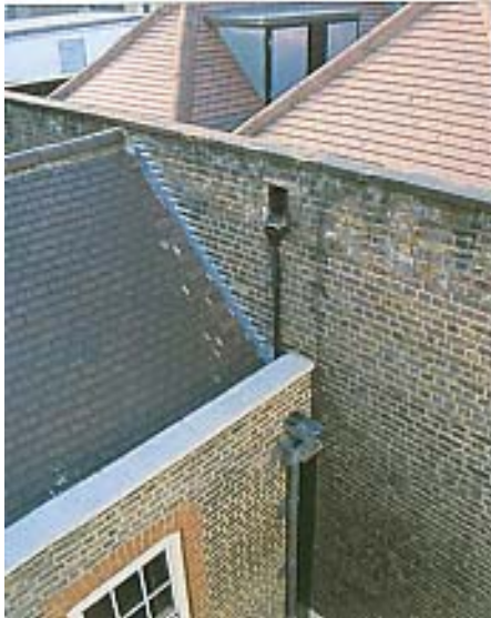
Roofscape in Meard Street, Soho, showing early eighteenth century roof form clad in clay tiles. Note the renewed lead rainwater pipe and Portland stone copings in the foreground.
