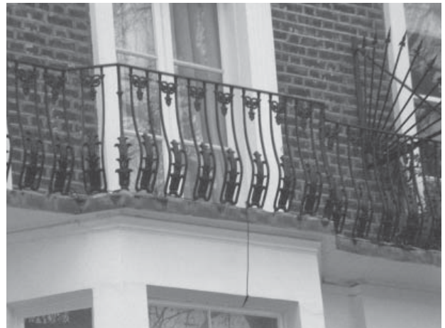
Figure 81: Mid C19th cast iron balconies to Vincent Square properties, with decorative palmette design to uprights
