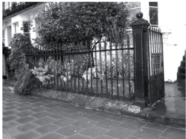
Figure 77: Original cast iron railings, gates and gate piers to No.13 Vincent Square
