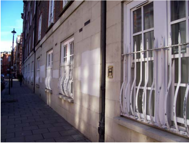
Figure 103: Replacement windows and poorly maintained ground floor facade, Queen Mary Building
