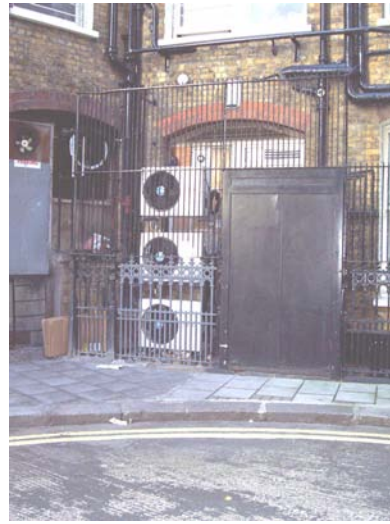
Figure 104: air conditioning units on King Scholars Passage
