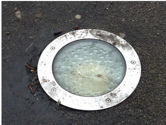
Water ingress following normal maintenance operations
