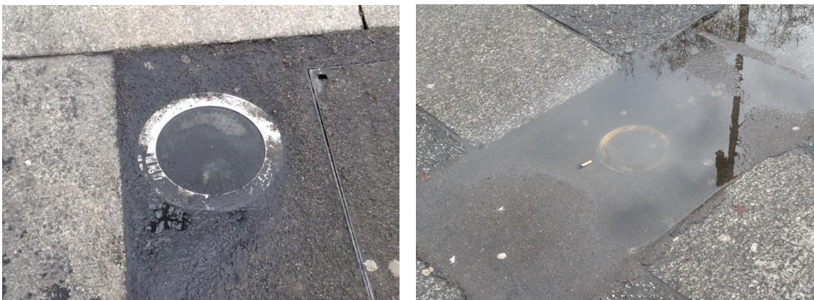
Up lighters installed with poor drainage
