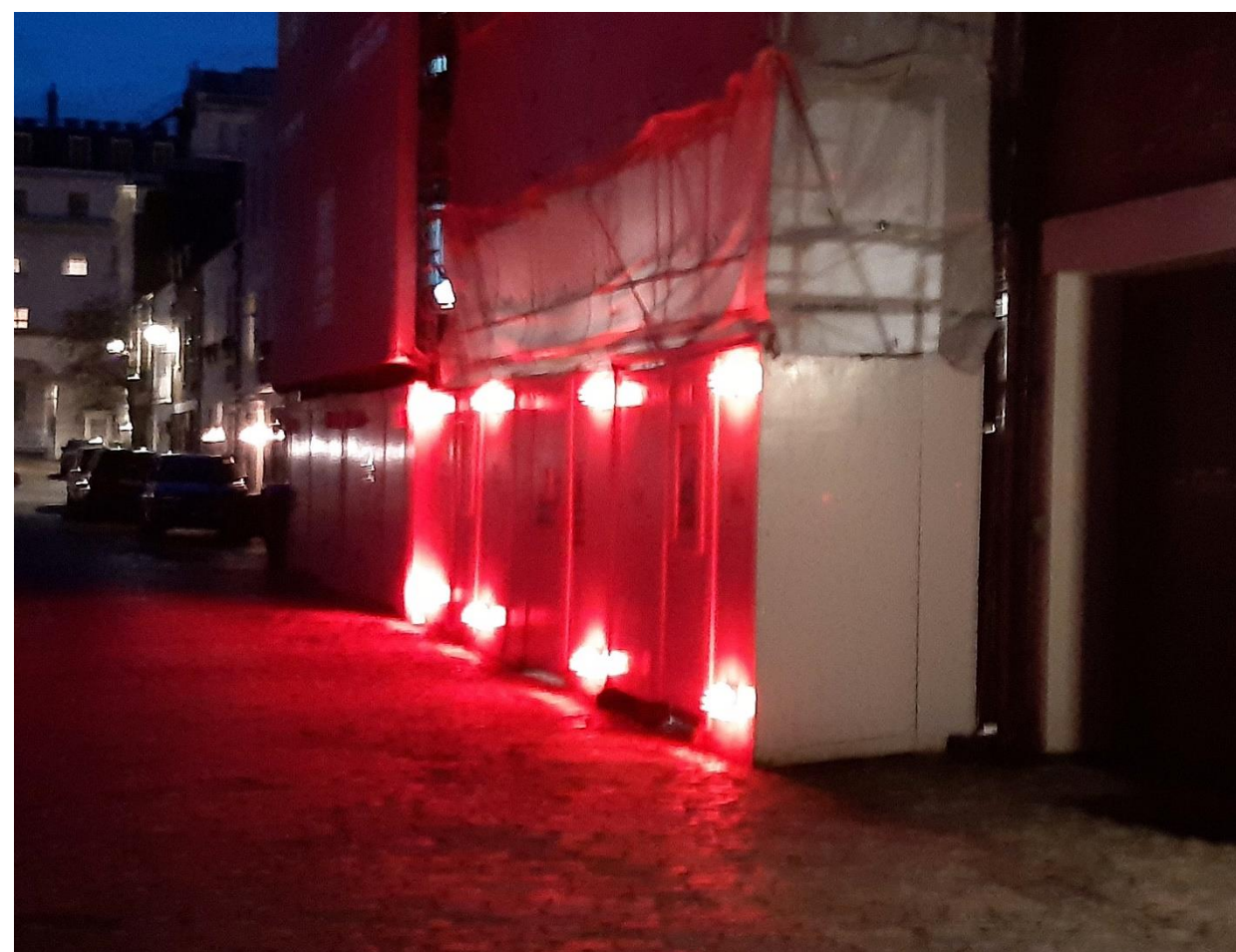
Image 58: Example of poor hoarding lighting
