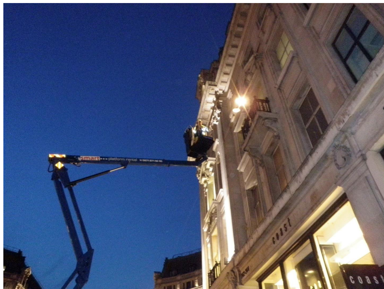
Image 59: Specialist tower wagon required to access wall mounted lighting
