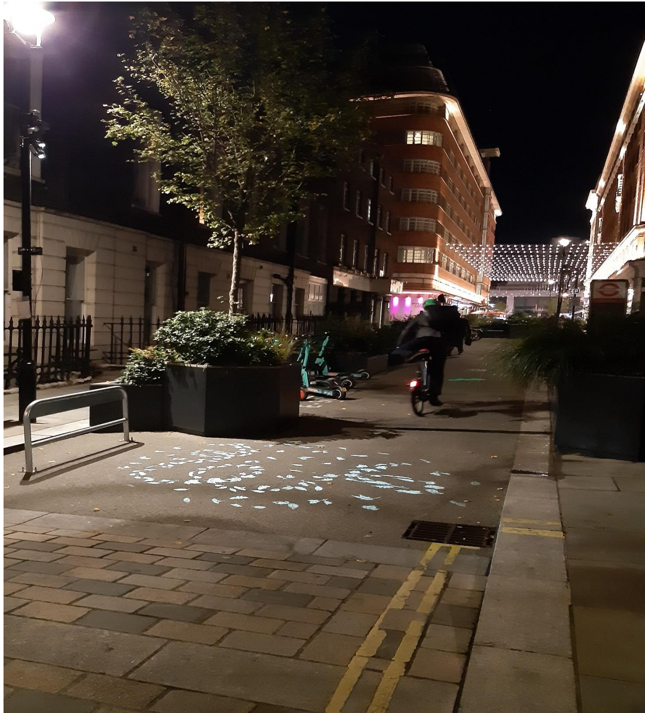
Image 23: Quebec & Old Quebec Street Spot light and wall catenary lighting
