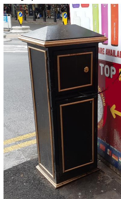
Image 44: Metered Feeder Pillar
