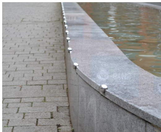
Figure 33: Example of studs used to protect the stone edge, and therefore prevent damage.
