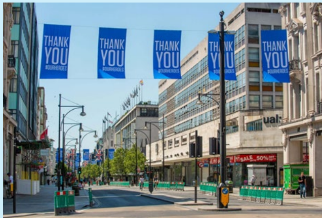
Figure 60: King Street, St James's Westminster, 6-week repair and replacement of footpaths and kerbs.
