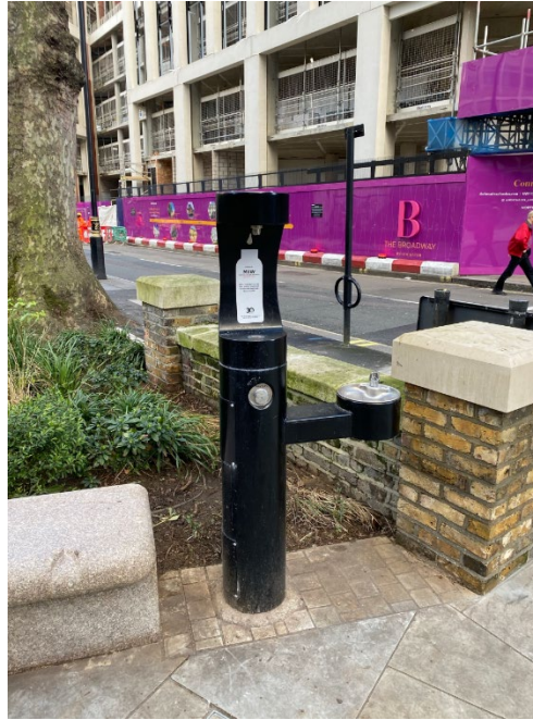
Figure 35: Drinking water fountain, Christchurch Gardens.
